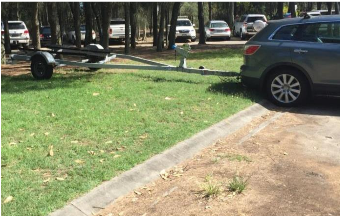
Figure 21: Dish drain used at rear of sealed portion of car and trailer space
