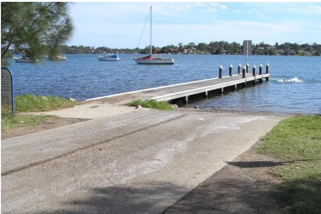
Figure 20: Extension of concrete surface beyond ramp crest
