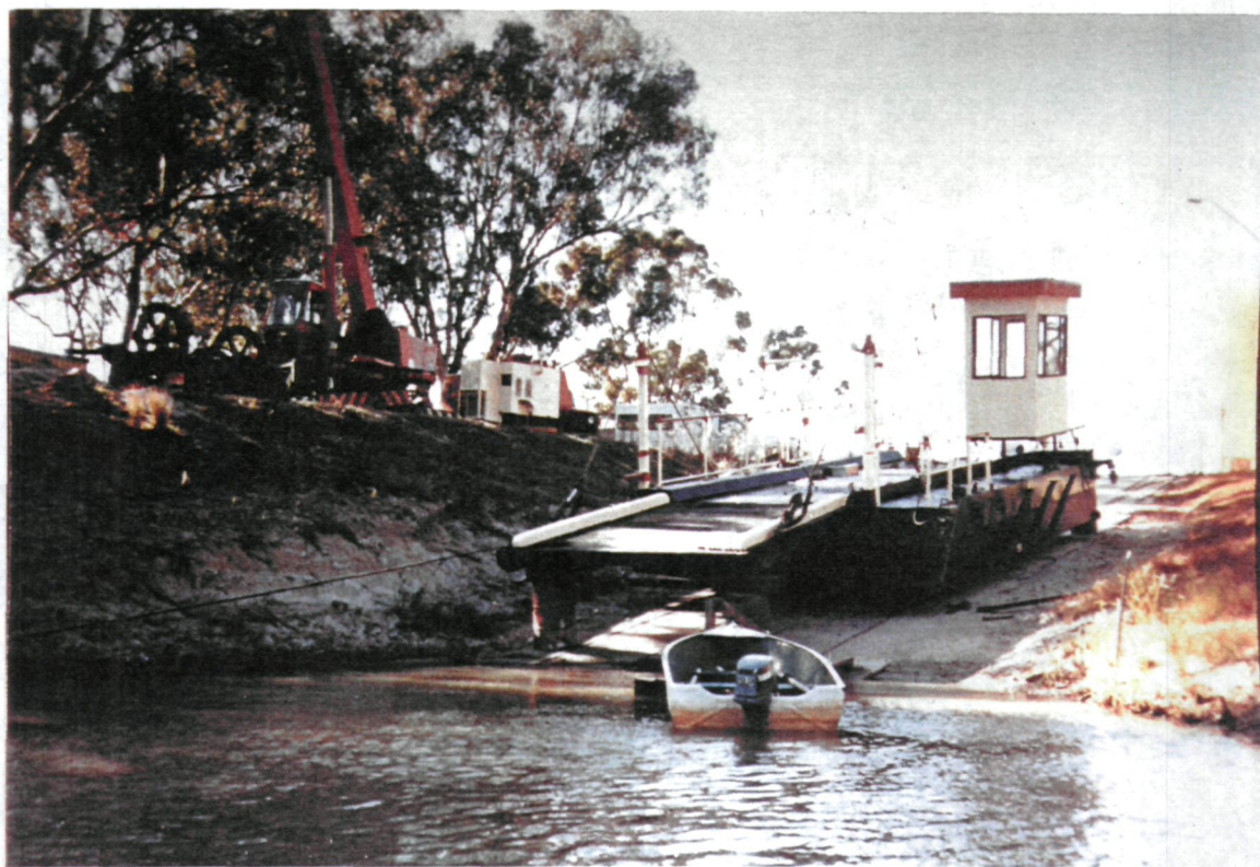
Speewa ferry on the banks of the Murray River during an overhaul
