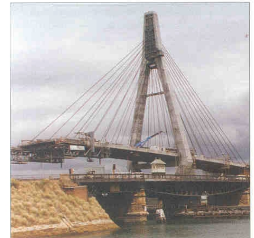
The Anzac Bridge during construction and the 1903 Glebe Island swing bridge, in 1994
