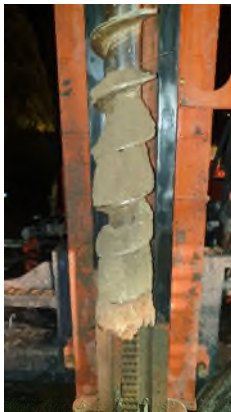
Photo 21. 02.12.2020 Close-up of soil in auger at GBH08 with gravelly sand fill overlying red residual clay.
