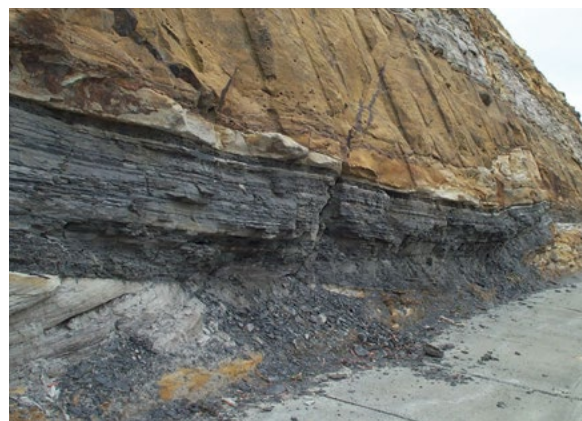
A crumbly shale band, which if higher up the cutting would need to be stabilised.
