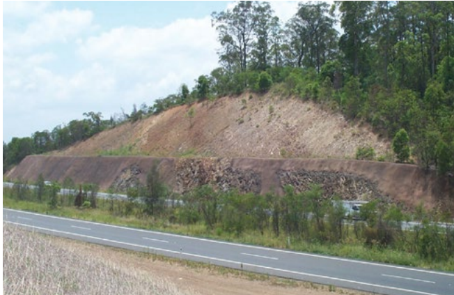
A dark earthy red/grey/brown colour helps recede the shotcrete into the rock of the lower half of the cutting on the Pacific Highway near Taree.
