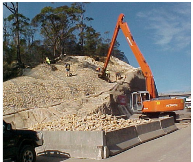
Rock filled mattresses placed over shotcrete application, Great Western Highway at Linden.
