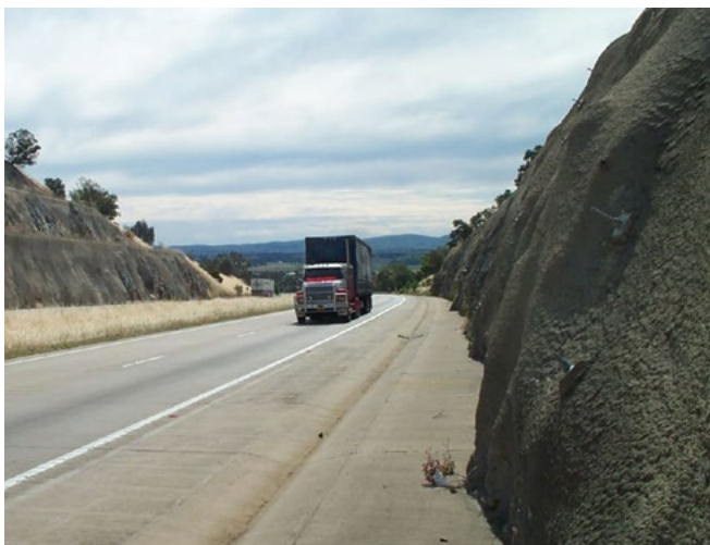
Two cuttings on Hume Highway, one with a setback and limited shotcrete (left), the other adjacent to the road requiring significant shotcrete coverage.
