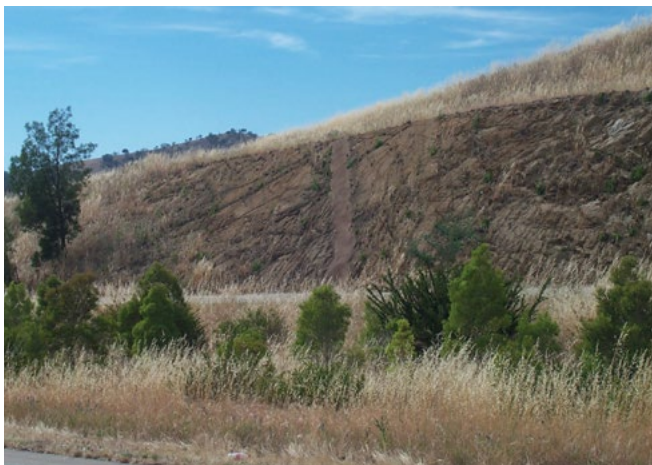
Excellent colour match on this cutting on the Hume Highway renders the shotcrete practically invisible. Colour matching works best where the rock is monochromatic.
