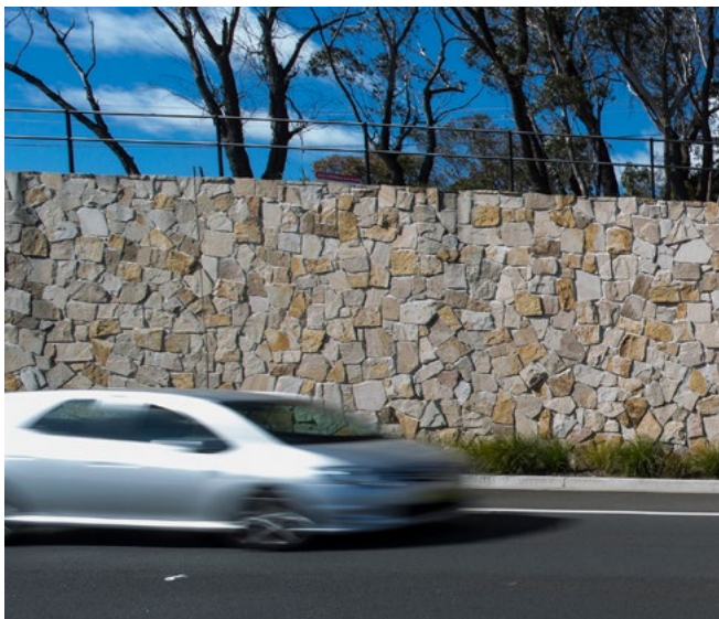
Materials and characteristics of new elements were carefully designed to fit with the local area, and two service roads were constructed for safer access to properties.
