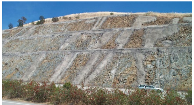
Two cuttings with similar stability problems. Precision design and progressive stabilisation can minimise the extent of shotcrete (Hume Highway).
