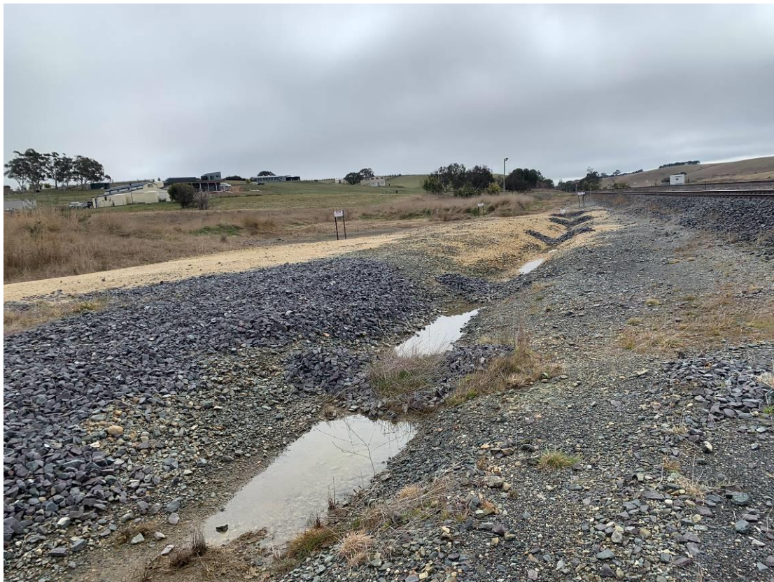
Photo 15: Rock armour upgradient of trainline running from the middle to the north culvert. Some sediment visible on rock armour. Pooled water in rock armoury visible. Water is clear and not running off-site. Facing north-east.
