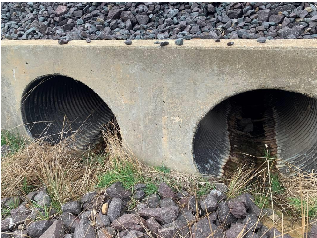
Photo 16: Upgradient of northernmost culvert. No evidence of surface water run off on site. No evidence of sediment buildup on rocks. Rock armor and natural vegetation allow for sediment control in surface water.
