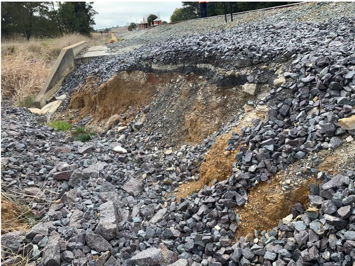
Photo 9: Visible evidence of erosion due to loss of ground cover (ballast material) upgradient of southernmost culvert. Remaining stable and no major further erosion since last inspection. Facing north-east.
