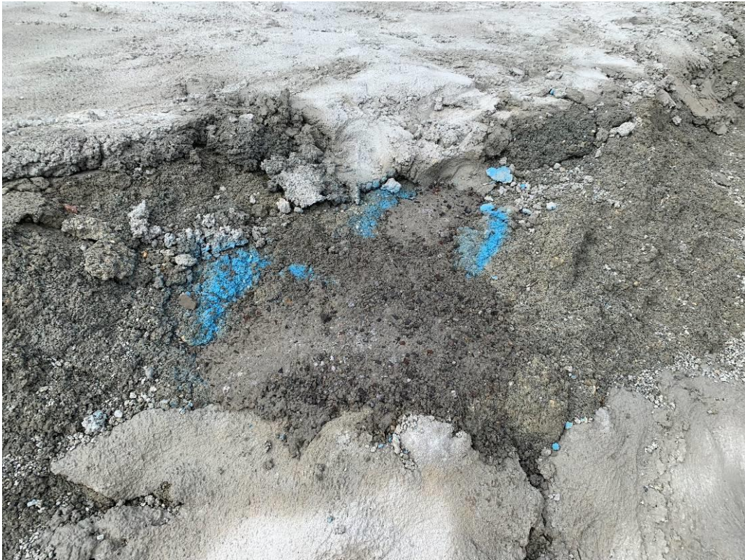
Photo 21. Two exposed geofabric layer markers on the main stockpile which were identified during the previous inspection (19/07/23), that have since been filled in with concrete.
