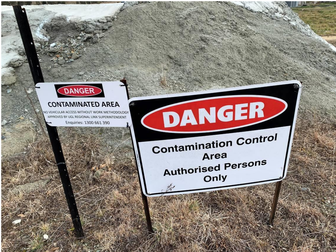
Photo 18: Repaired exclusion zone signage in good condition. This signage was reported as damaged on the last inspection visit (19/07/2023).
