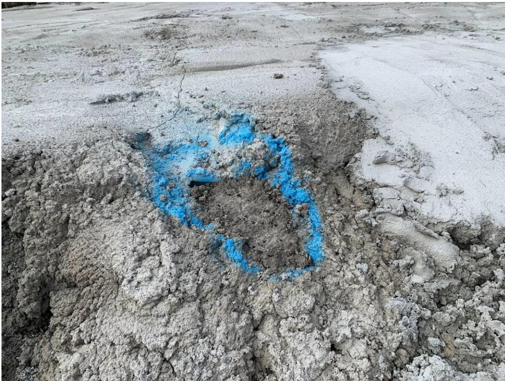
Photo 20. Exposed geofabric layer marker on main stockpile which was identified during the previous inspection (19/07/23), that has since been filled in with concrete.
