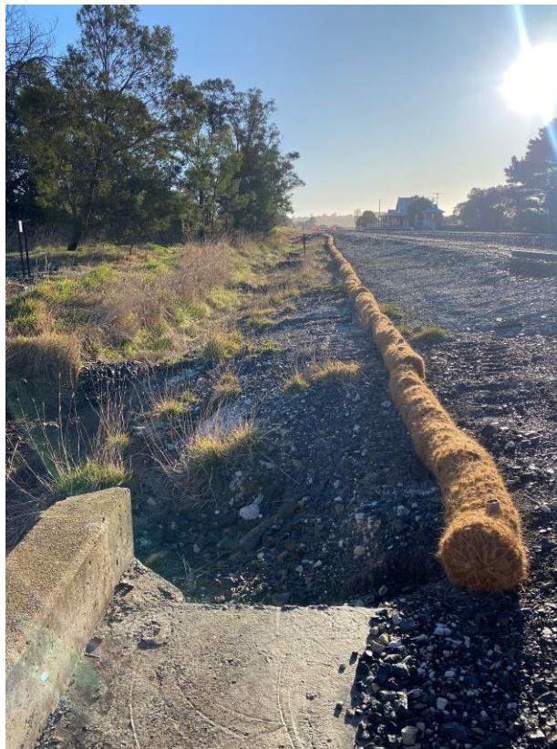
Photo 10: Upgradient of southernmost culvert showing previous silt fencing replaced by Coir sediment control logs, used as control measures for sediment control. Facing north.
