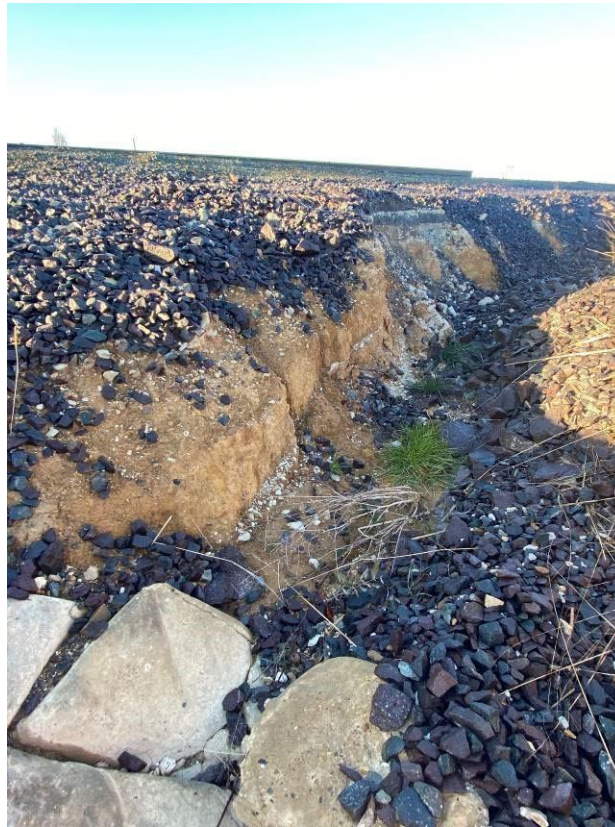
Photo 9: Visible evidence of erosion due to loss of ground cover (ballast material) upgradient of southernmost culvert. Remaining stable and no major further erosion since last inspection. Facing south.
