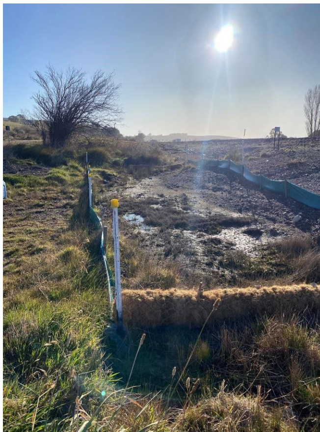
Photo 14: Upgradient of trainline culvert facing north, showing minor pooling on site near rock checks and silt fencing. New Coir sediment control log placed in drainage channel running towards middle culvert.
