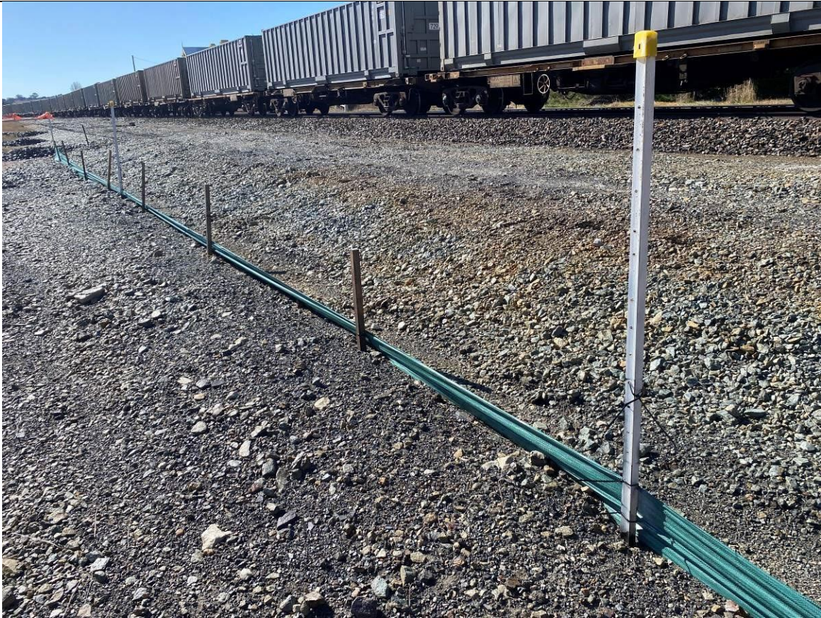
Photo 25. Damage to silt fencing between southern and middle culverts. Ties holding fencing to stakes are no longer functioning and silt fence cannot remain up. Ramboll recommends fixing or replacing this fencing.
