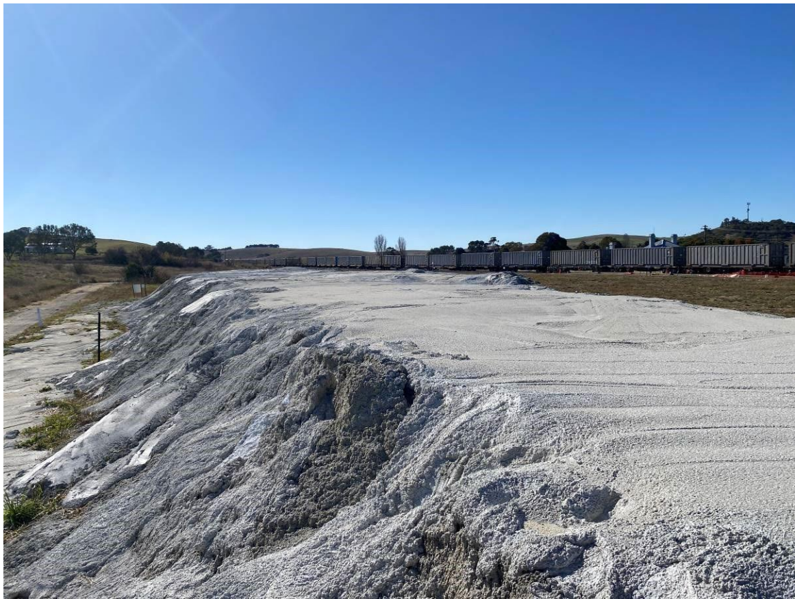
Photo 22. Picture of stable stockpile capping on site. Minimal cracks and breaks can be seen on the topside of the stockpile.
