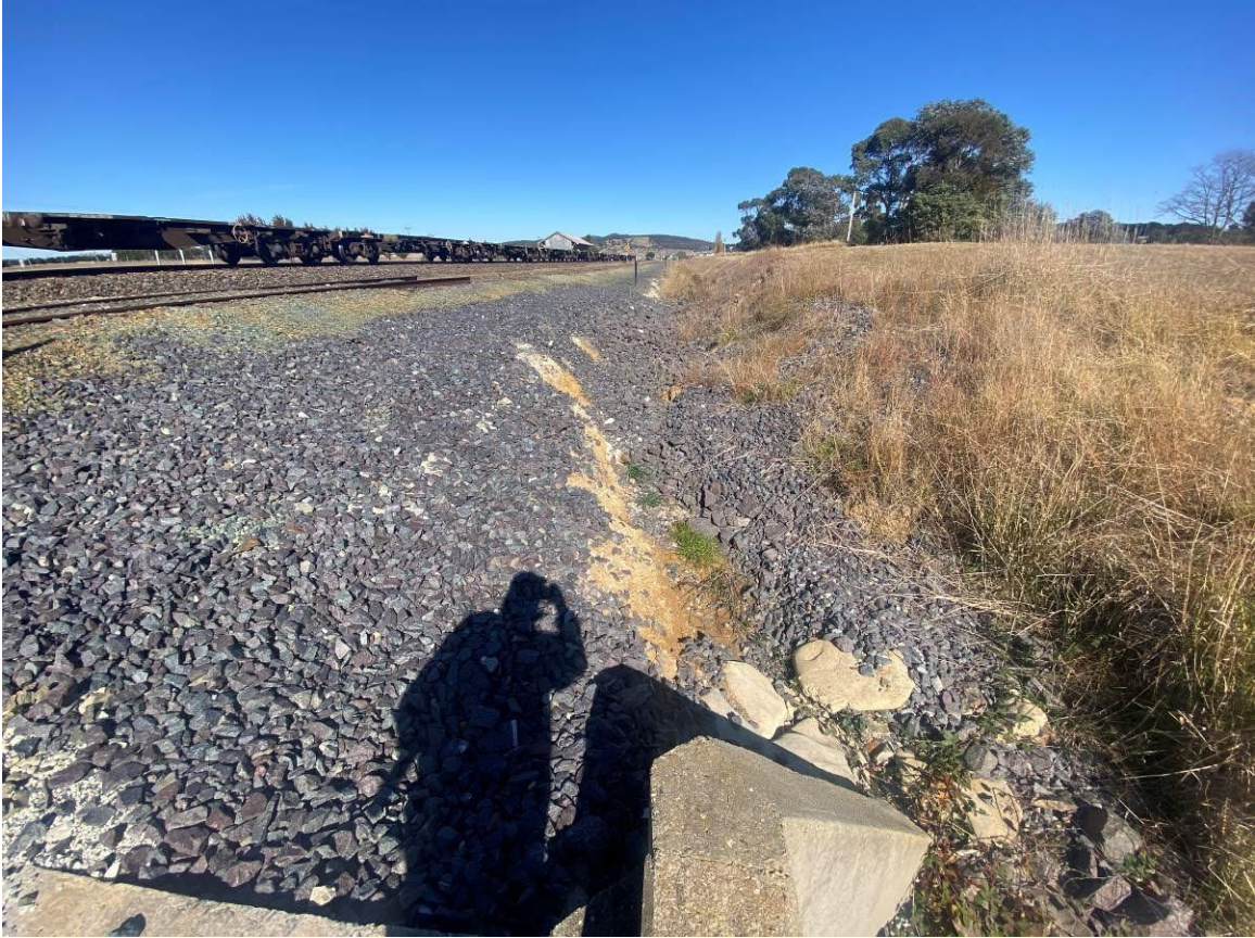
Photo 24. Evidence of erosion upgradient of southern most culvert noted in site inspection dated 20 April 2023 remains on site but stable.
