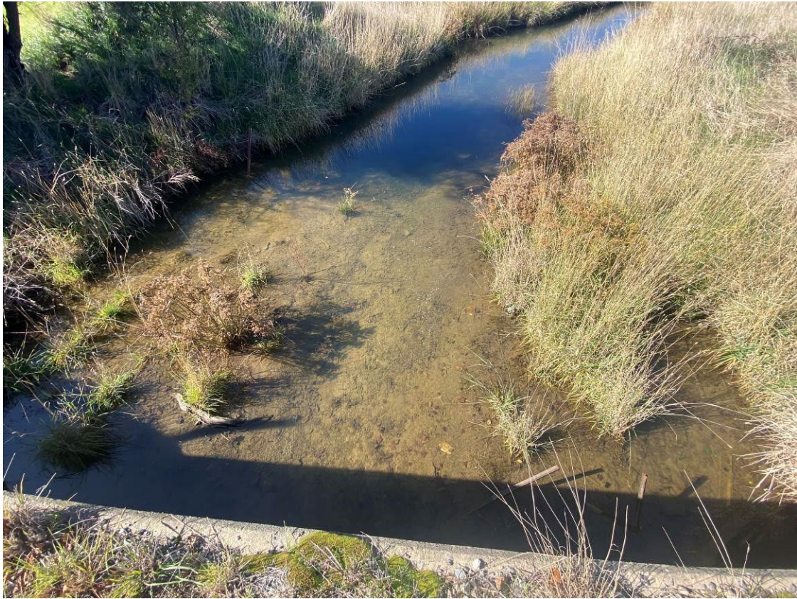
Photo 4: Outlet of culvert under Golburn street, downgradient of southernmost culvert on site, showing evidence of surface water run off on site. Water remains clear with no turbidity and no observable sediment.
