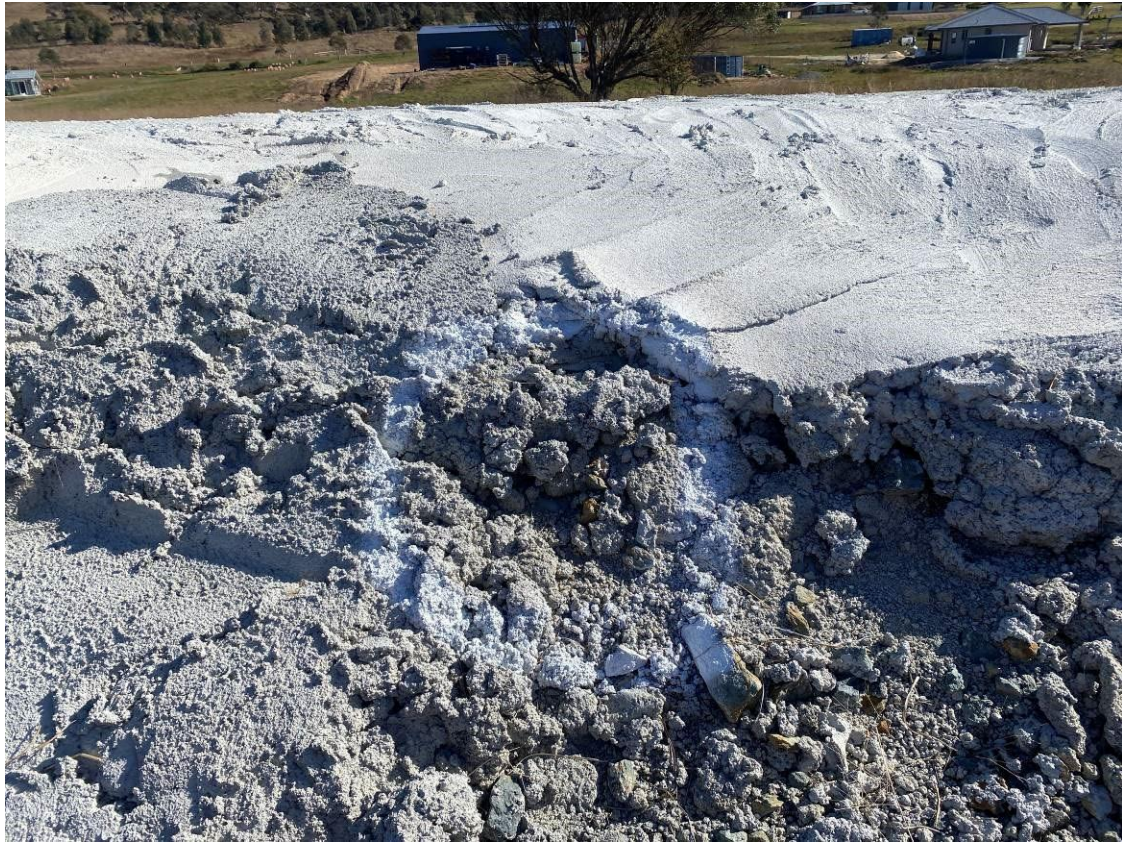
Photo 18: Geofabric marker layer visible in stockpile capping remained from previous inspection Approximately 10cm x 2cm. UGL representative stated patching works will take place Friday 19 May 2023.
