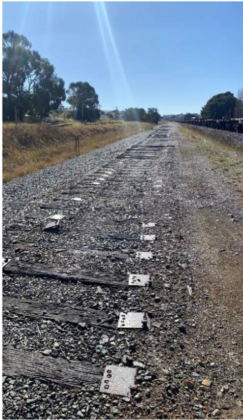
Photo 23. Poly sealant application noted in inspection checklist 15 March 2023 remains on Woodlawn siding. Gravels are sealed together and layer of sealant evidence by shine.
