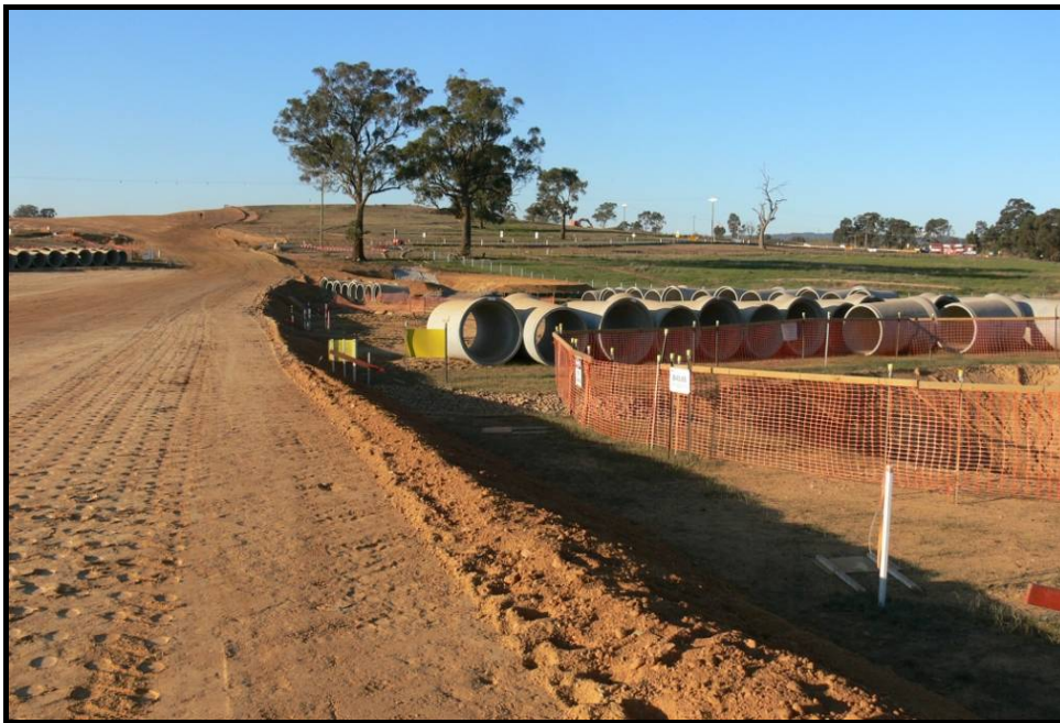
Plate 15 - Earth windrows at the edge of fills to control the exit of 'onsite' water down the fill batters to sediment retention structures.
