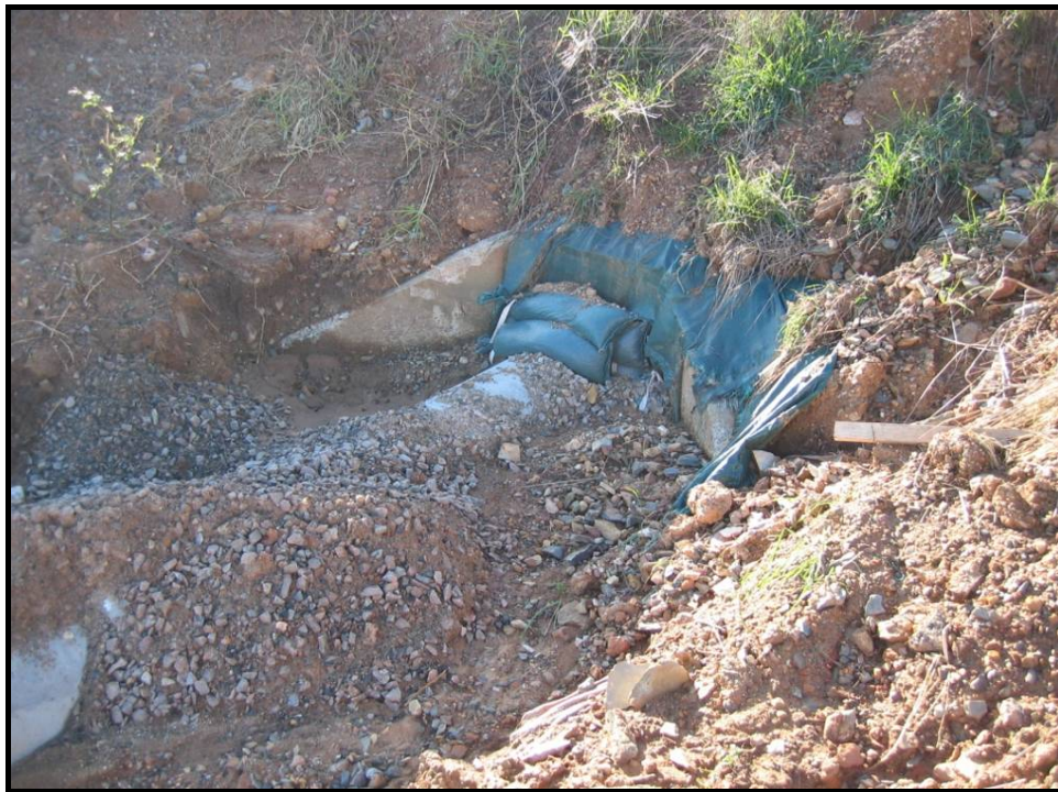
Plate 8 - Temporary extension of existing pipe to allow for placement of fill on new carriageway adjacent to existing. Note the seal around pipe joint to prevent sediment ingress.
