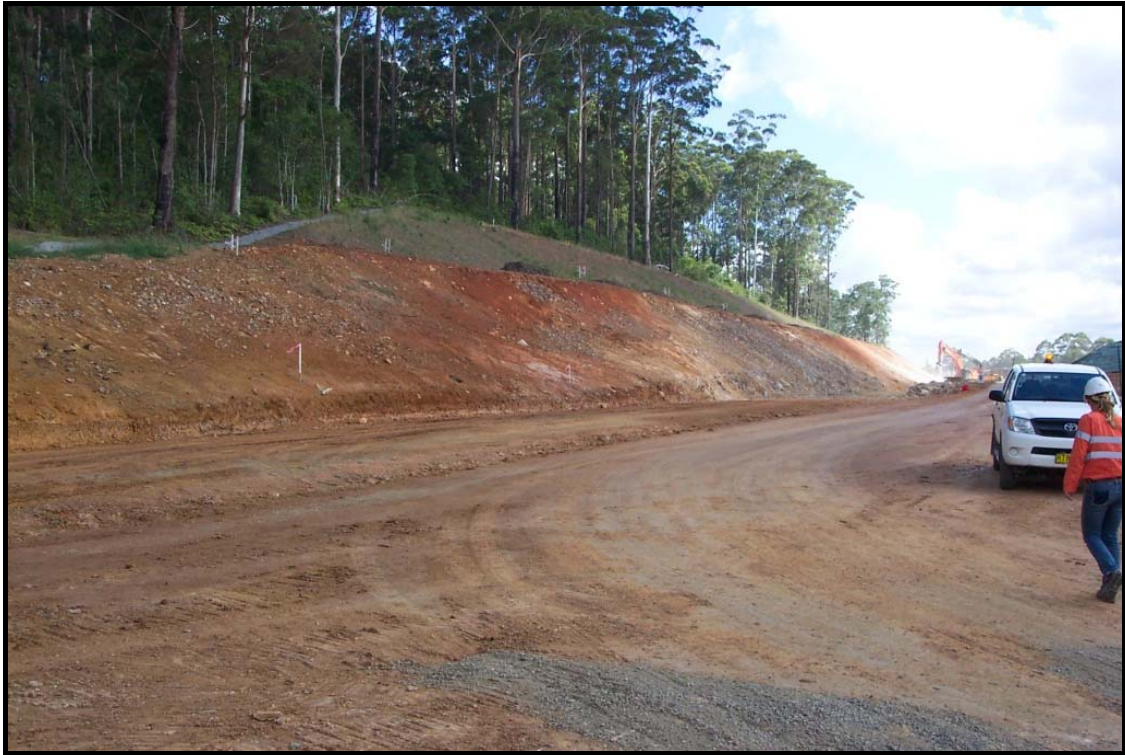
Plate 19 - Progressive stabilisation of a cut batter above a berm drain. Flows in the berm drain should remain disconnected from the cut-off drain behind the cut face until the batter face is rehabilitated.
