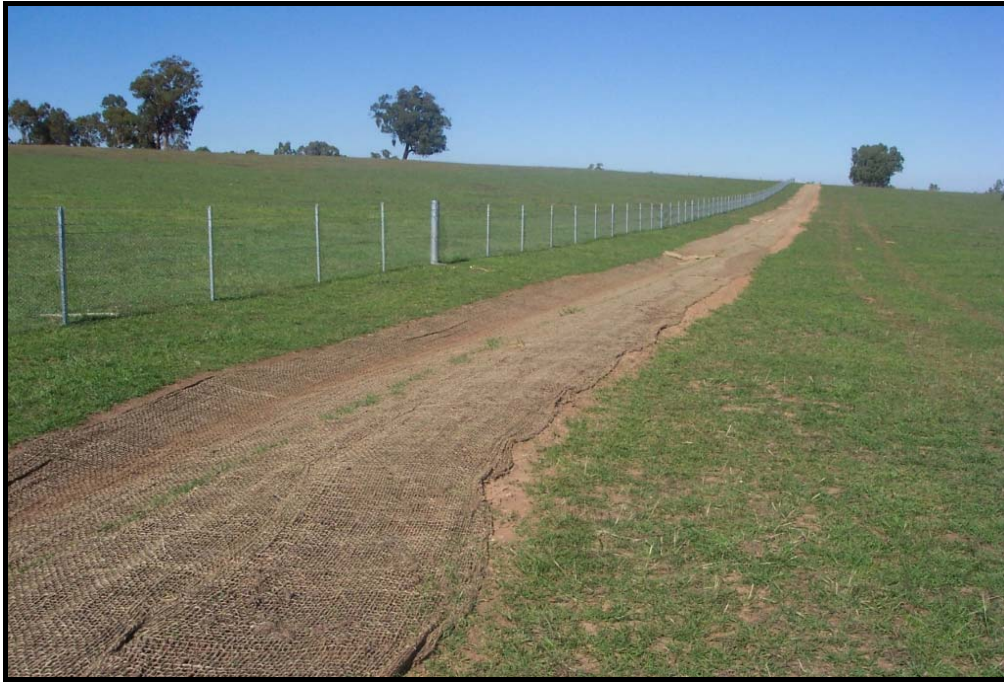
Plate 12 - Lined drain on the high side of the alignment to manage 'offsite' water.
