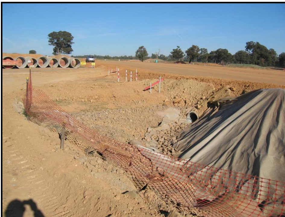
Plate 4 - Temporary pipe to convey 'offsite' water around culvert works area. While this is a suitable solution for temporary cross-drainage there is a significant risk of contamination of 'offsite' water due to lack of erosion and sediment controls around the pipe and channel.
