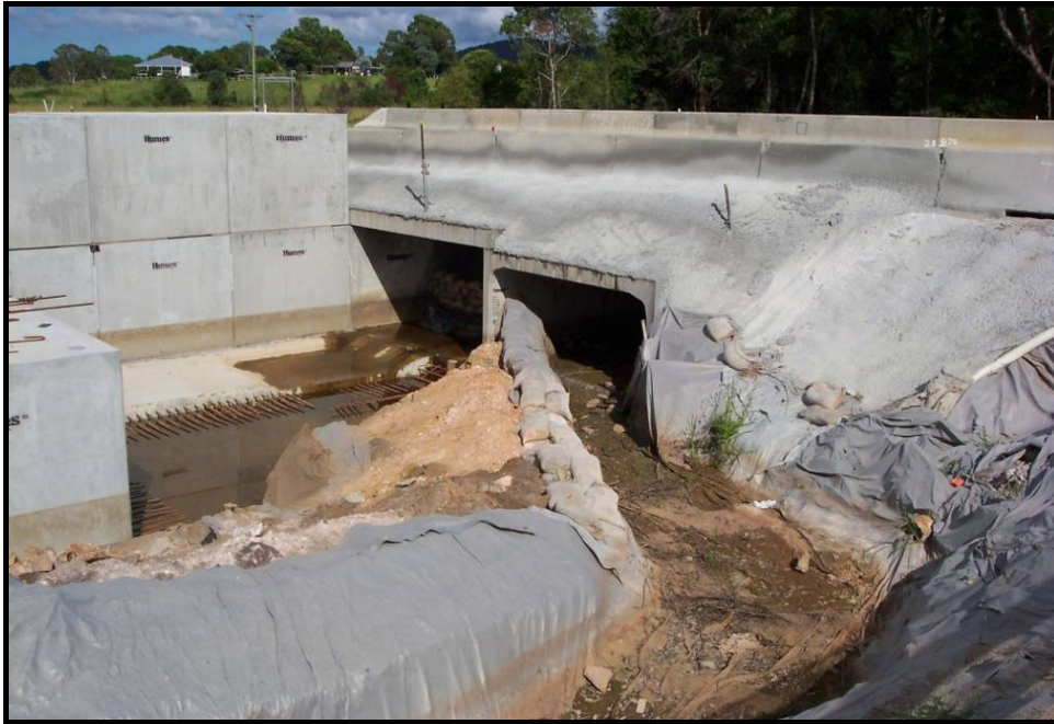
Plate 7 - Use of a half-height partial block of a multiple-cell culvert during culvert extension works.
