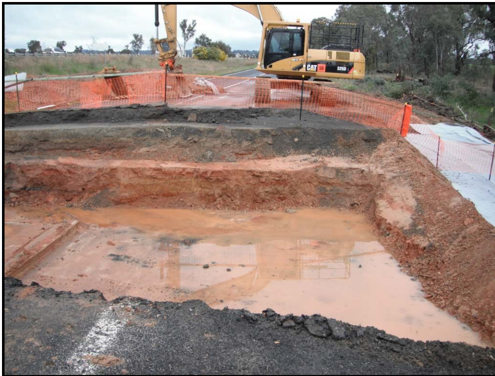
Plate 9 - Water flowing into excavation for an online culvert extension – needs to be treated prior to discharge. Diversion of ‘offsite’ flows is preferable.
