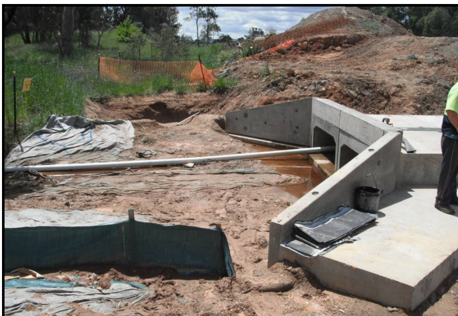
Plate 6 - Temporary pipe inside new, extended culvert to convey 'offsite' water through the works area until culvert (including rock-lined outlet) is complete.
