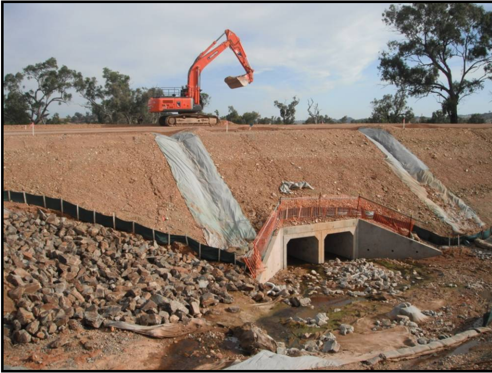
Plate 14 - Lined batter chutes to minimise erosion on a fill batter and to control flows.
