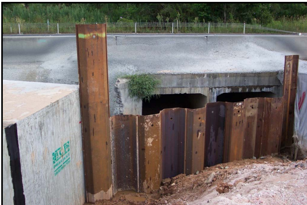
Plate 2 - Use of sheet piling to divert 'offsite' flows between new and old culverts. This level of control might be necessary where space is limited.
