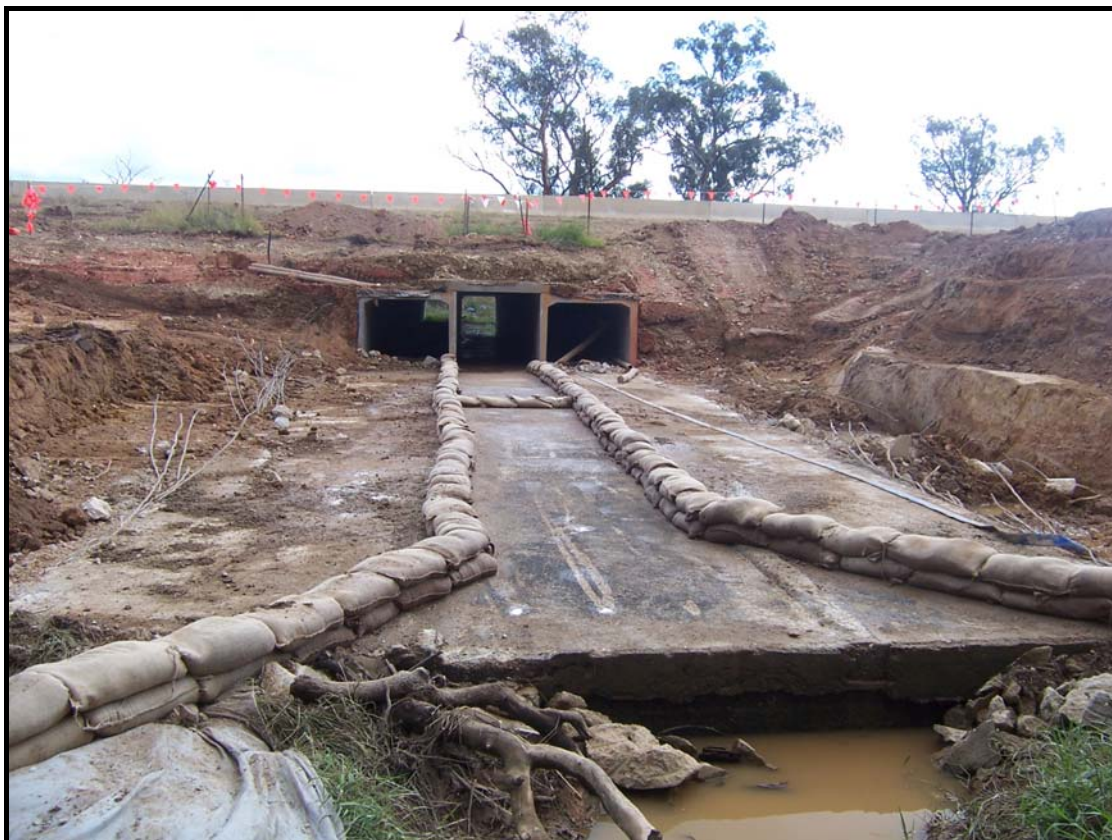
Plate 10 – Replacement of part of an existing culvert, with offsite water temporarily managed through a sandbagged channel on the old base slab.
