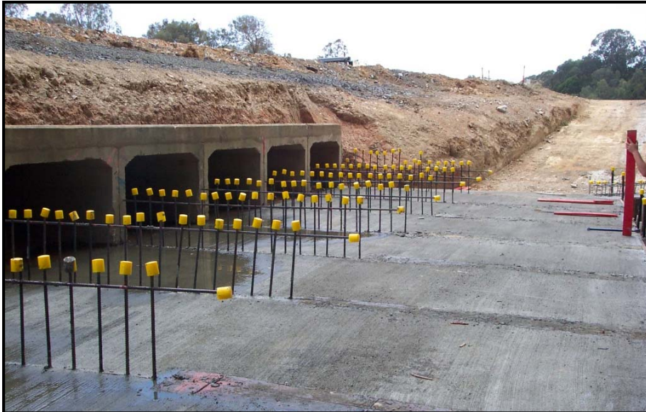
Plate 5 - Extension of an existing seven-box culvert for construction of an additional carriageway, Northern Hume Alliance project. Bunding is required at the edge of the concrete pad to keep 'offsite' water out of the works area.
