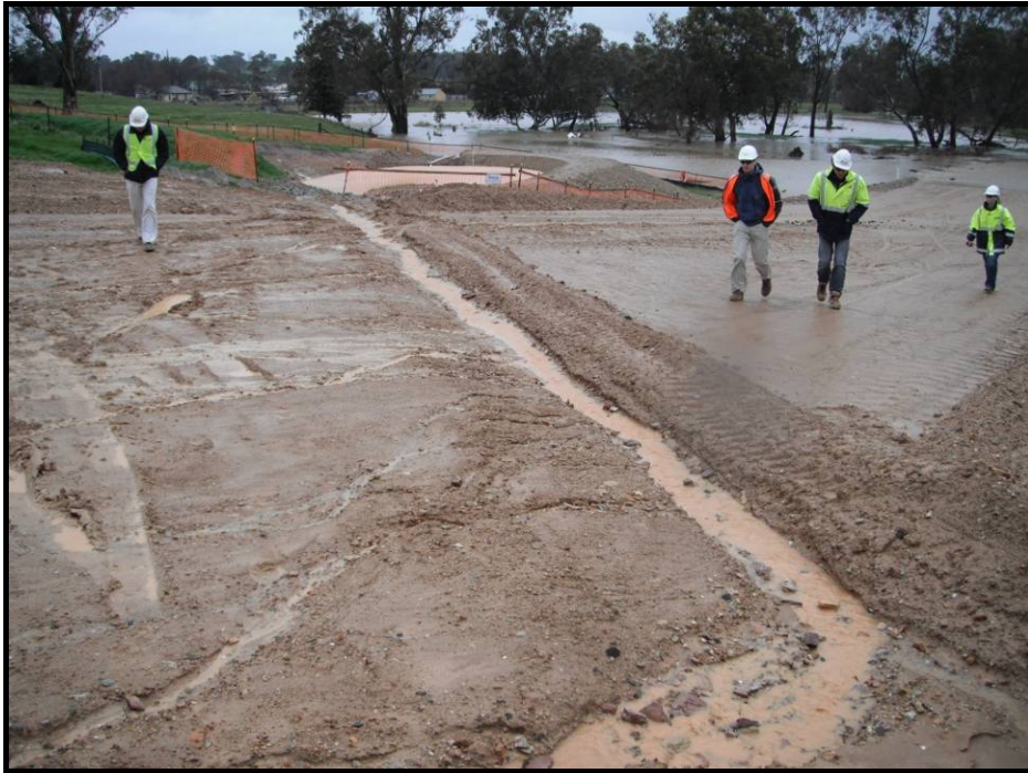
Plate 18 - Temporary cut drain across the formation to direct 'onsite' runoff to a sediment basin. Cut drains should also be used to break up a catchment into smaller erosive slopes when rain is imminent or during periods of site closure.
