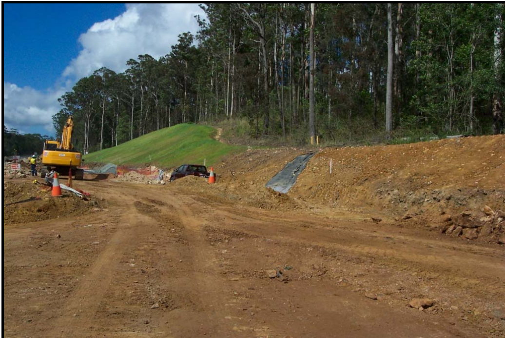
Plate 11 - 'Offsite' water in the cut-off drain and upslope depression is spilling onto a piece of black plastic, then into the works area. Temporary cross-drainage should be provided to prevent this scenario.
