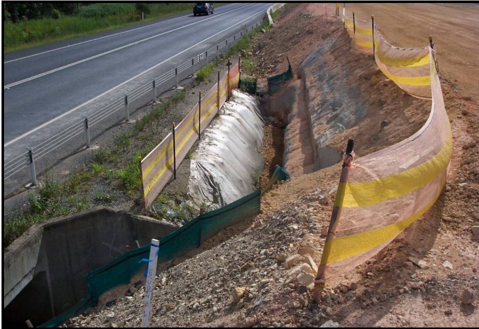
Plate 3 - Extremely space-constrained scenario where the new culvert is at a differing alignment to the existing, with insufficient space between carriageways to effectively divert flows.
