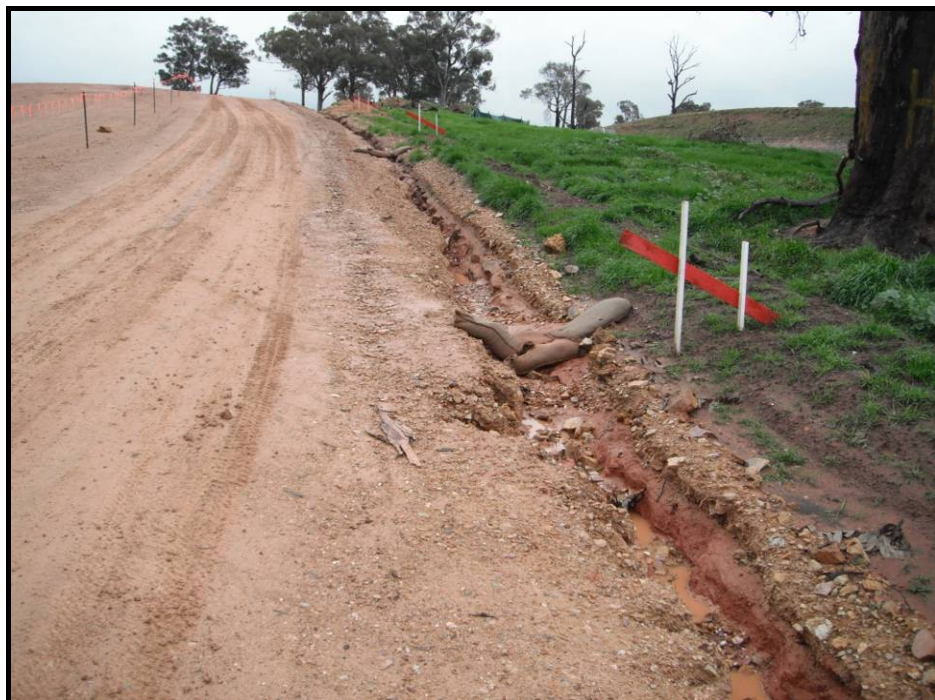
Plate 17 - Unlined drain at edge of formation showing significant erosion despite regular sandbag check dams. Lining of this drain would prevent erosion.
