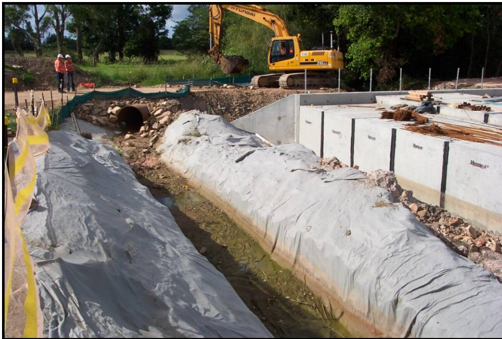
Plate 1 - Temporary creek diversion during construction of an online culvert, Pacific Highway Coopernook to Herons Creek project.
