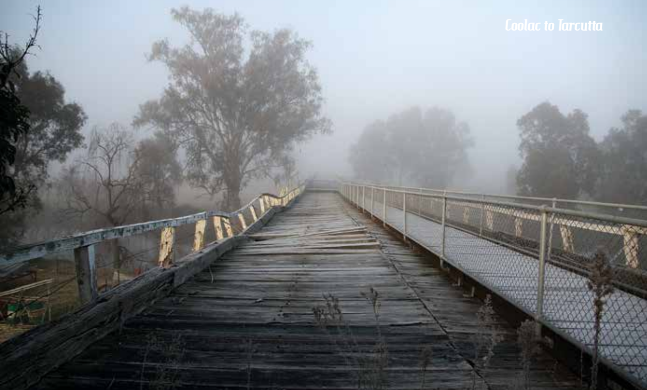
Former Hume Highway timber trestle bridge across the Murrumbidgee River floodplain, Gundagai
