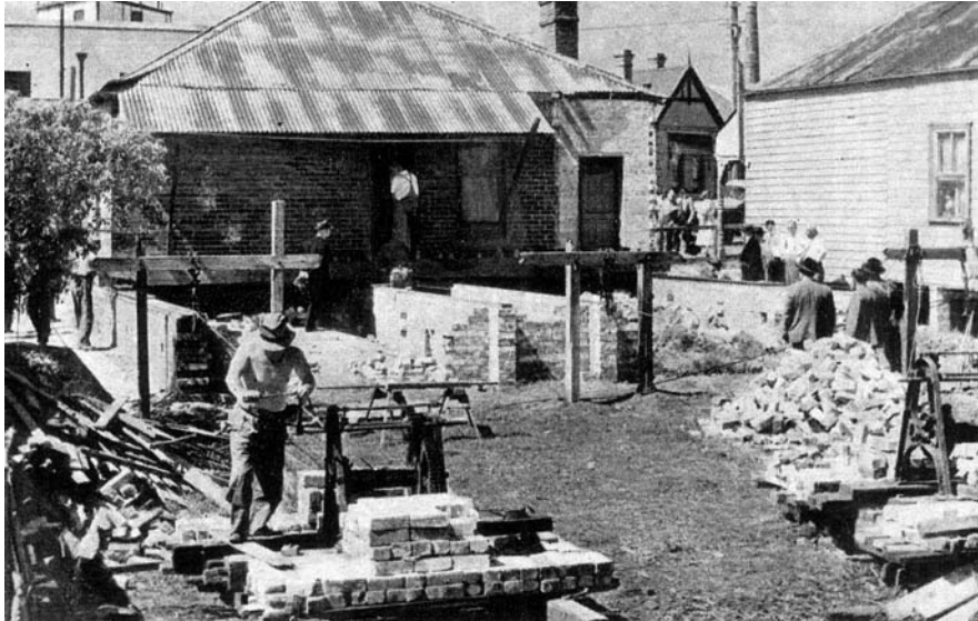
Figure 8 Moving House! A brick cottage affected by road widening was moved as an experiment by the DMR in 1950. This shows the cottage before moving. DMR, Annual Report , 1950, opp p 12
