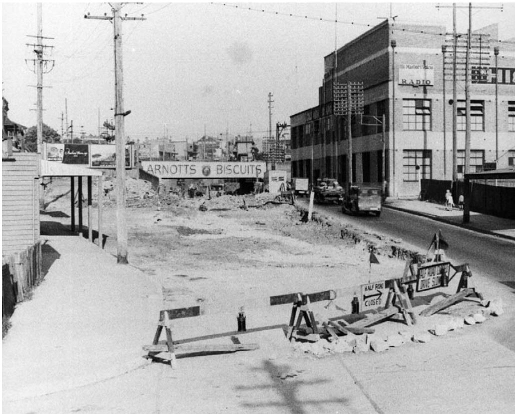
Figure 11 Maintenance, October 1938. Upgrading roads was a constant chore as seen on Parramatta Road near the Homebush underpass. Source: GPO1, 32541
