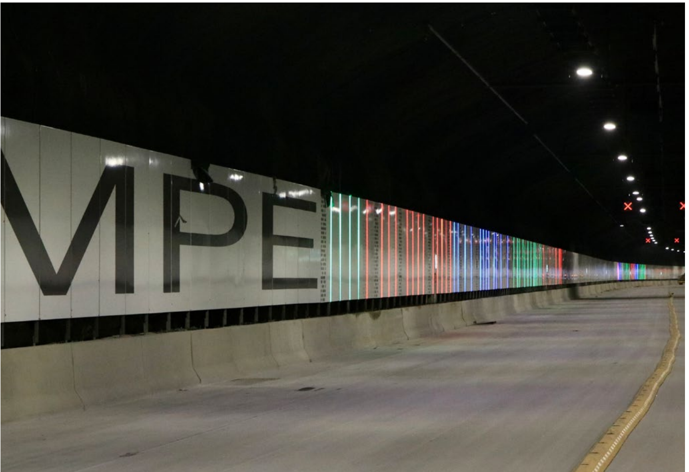
In the M4-M8 tunnel Lighting and strong colours are important in making the total 23km journey visually stimulating. If they can be modified in the control centres to reflect a calendar of events such as road safety week and the Mardi Gras then there is an added dimension to the visual interest.
