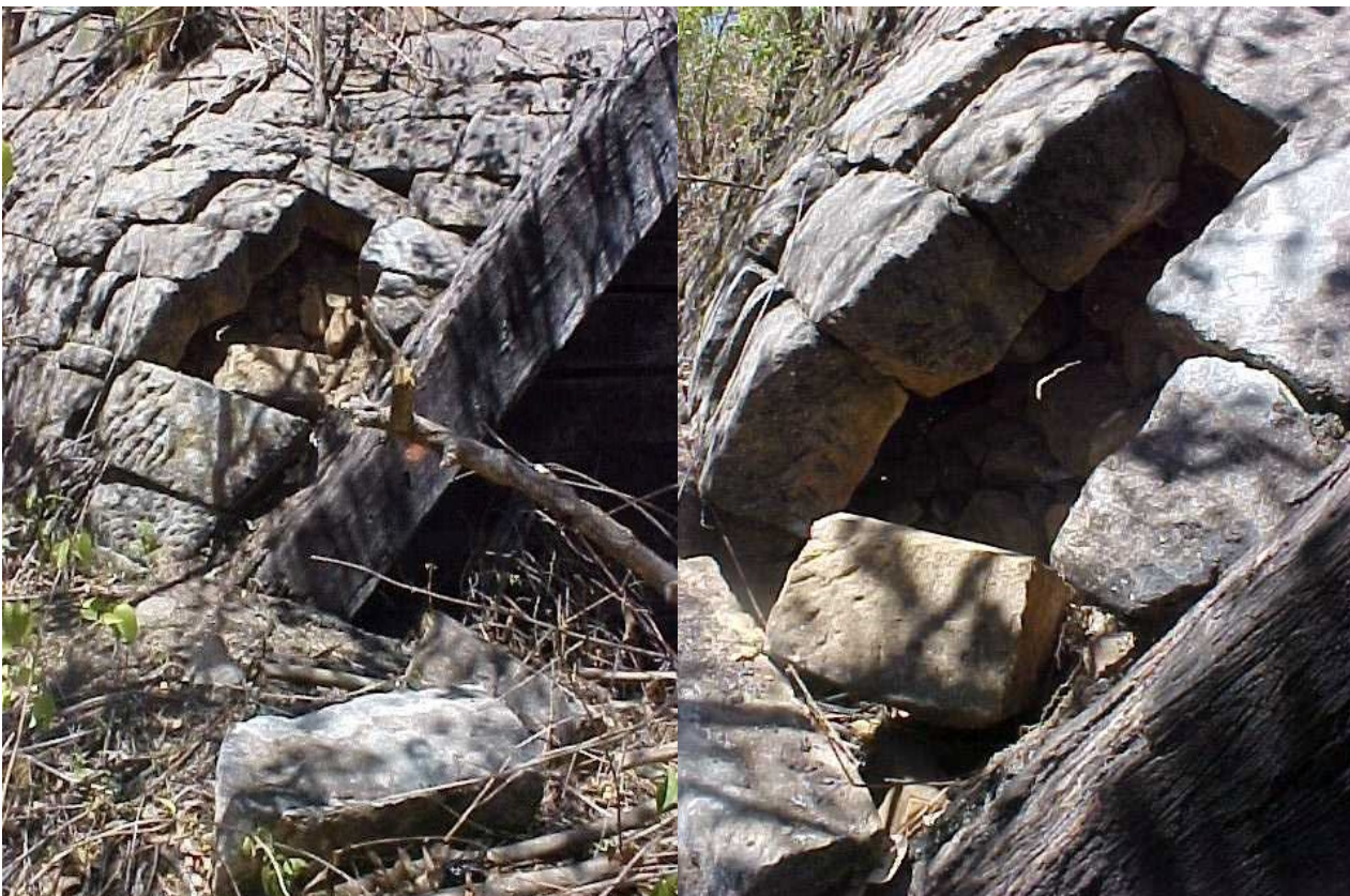
Figure 2-47: Signs of failure of embankment beginning in 2003
