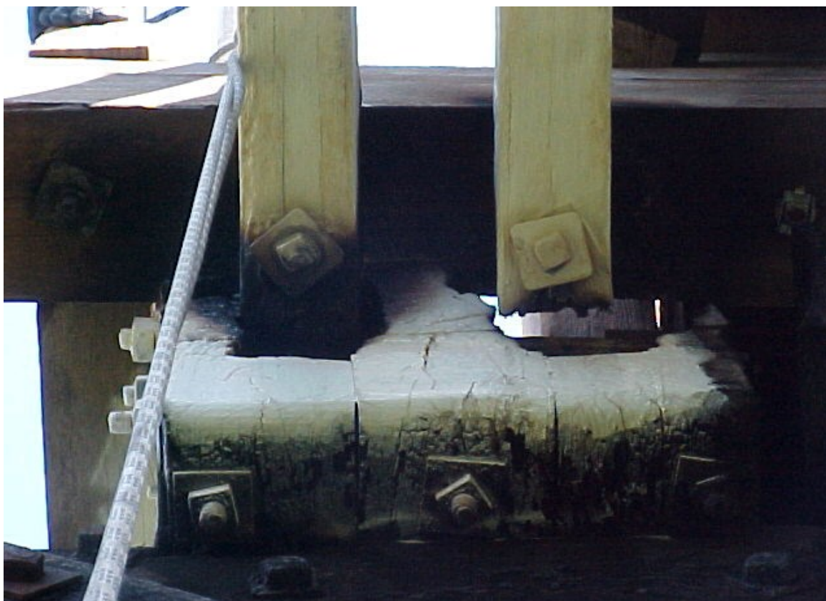
Figure 2-43: 2003 fire damage showing bottom chord damage
