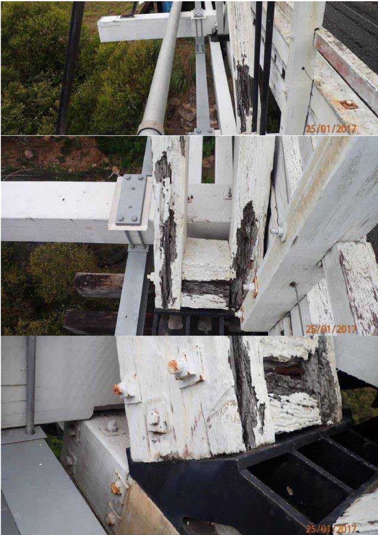
Figure 2-63: Photographs of typical deterioration of principals and diagonals, 2017 inspection 129
