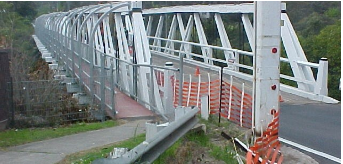
Figure 2-46: Temporary external footway during 2004 repairs
