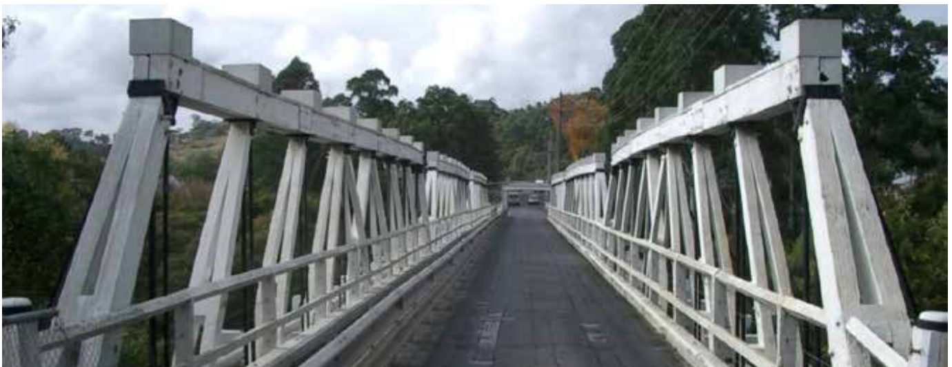
Figure 2-58: Visually dominant “castellated” flashing on top chords
