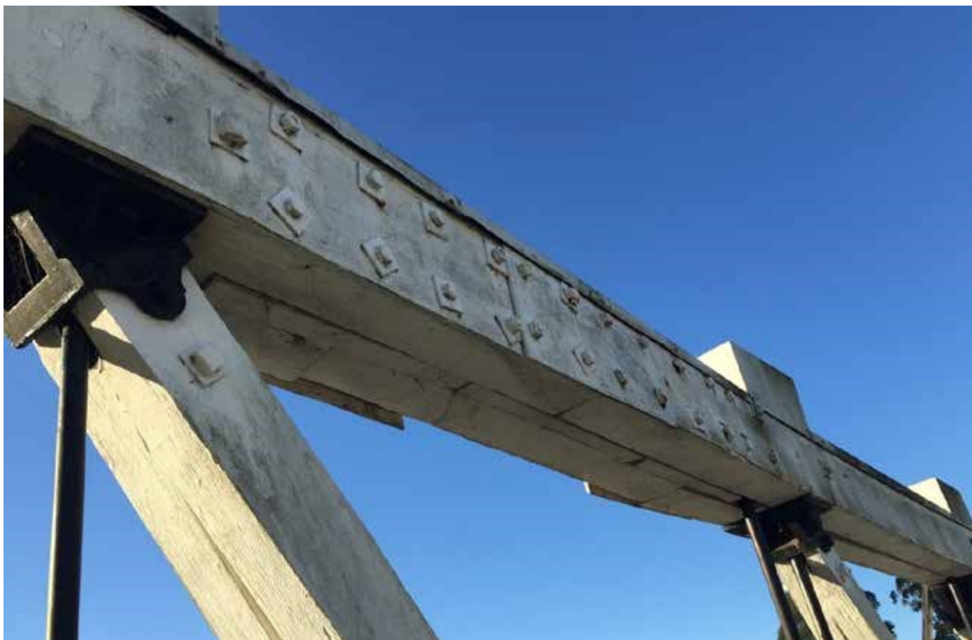
Figure 2-56: Additional splices at G-H in Span 2 Upstream
