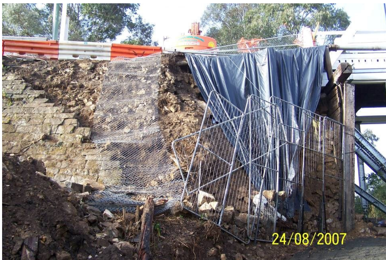
Figure 2-48: Failed abutment and embankment due to slip in 2007
