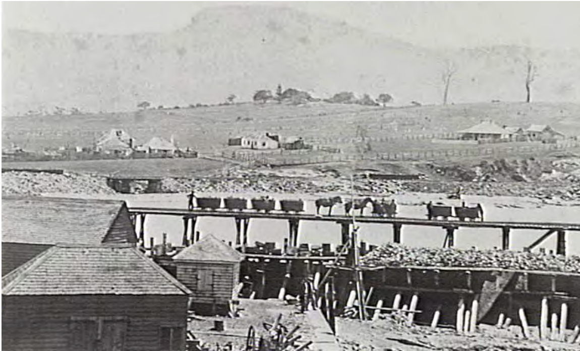
Figure 3.3 Construction of Belmore Basin, looking west and showing temporary levee (Source: Boleyn & Boleyn 1999, p.13)
