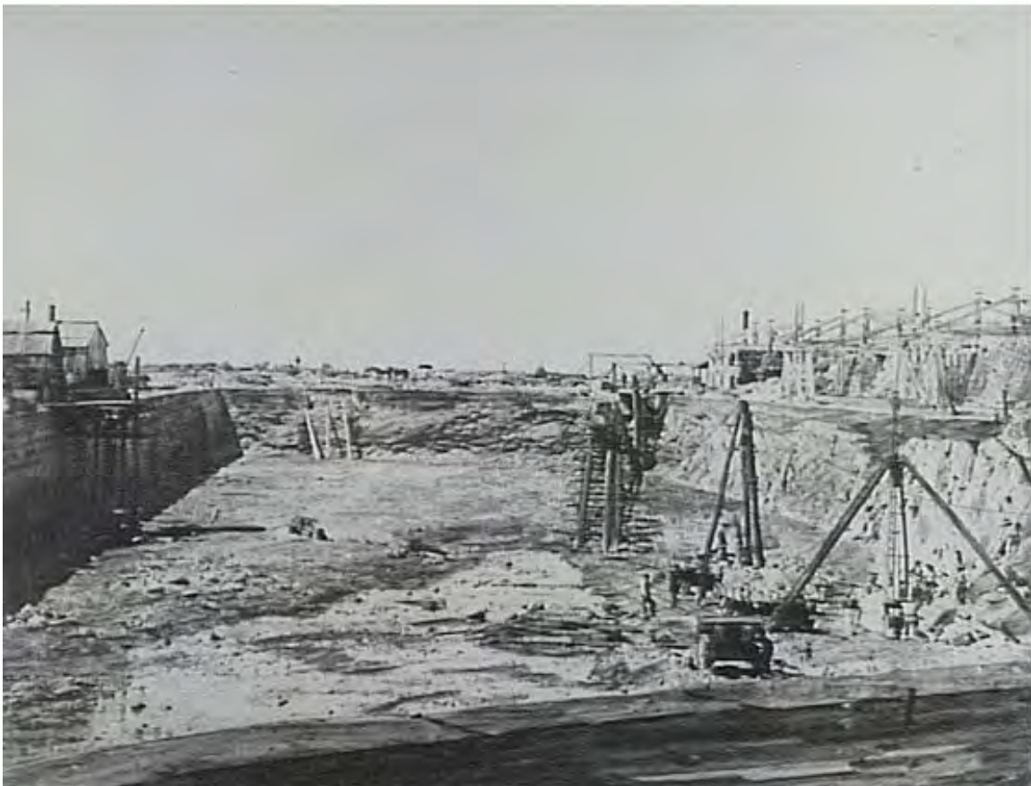
Figure 3.4 Wollongong Basin [c.1860 to 1880] (Source: State Archives and Records Authority of New South Wales, ID: 114E7bX1)
