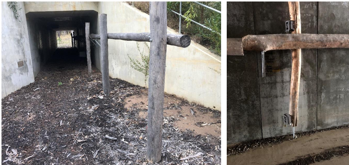
Plate 1: All monitored box culverts contained fauna furniture and some featured mulch spread over the concrete floor (left). Cameras were installed on the center post within each culvert – one viewing along the rail and the other along the floor (right).
