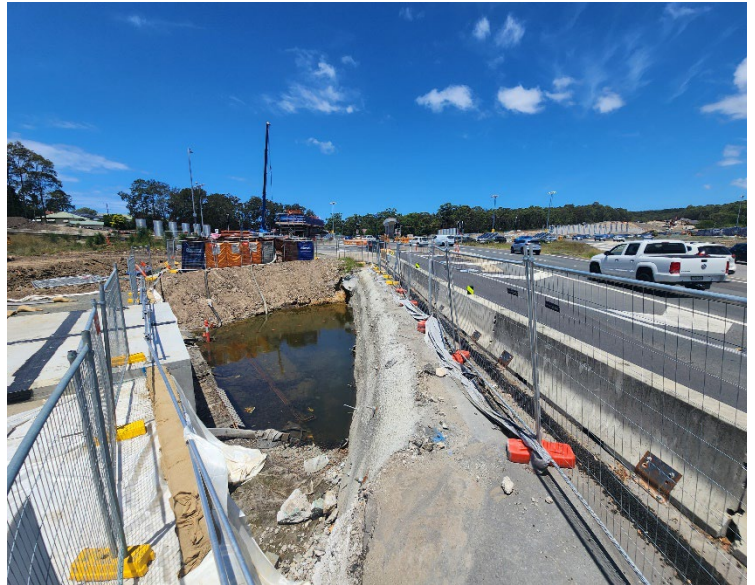
Image 2: Northern Interchange, view of the works on the northern side of Newcastle Road.
