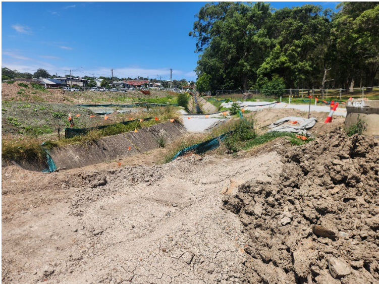
Image 3: Northern Interchange, view of the works on the southern side of Dark Creek. the culvert diversion can be seen in the photo, being used as a temporary sediment basin.
