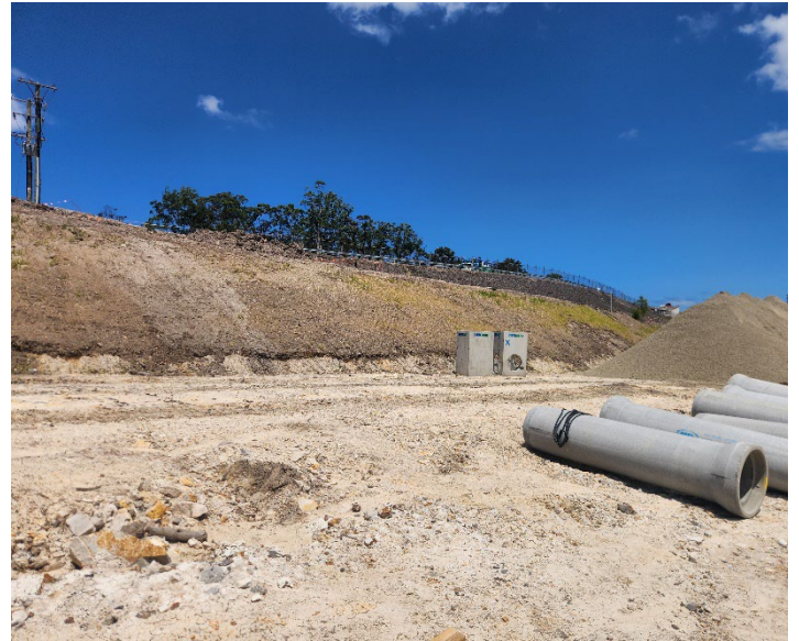
Image 6: Main line looking east towards John Hunter Hospital. This area is currently in the process of being handed back to the RP2J project.
