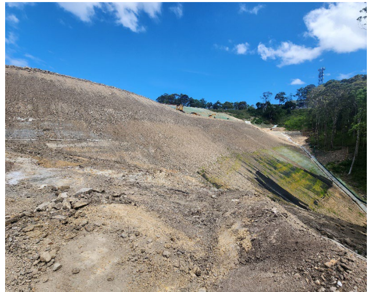
Image 8: Southern Interchange, the batter is in the process of being stabilised with various forms of final landscape designs.
