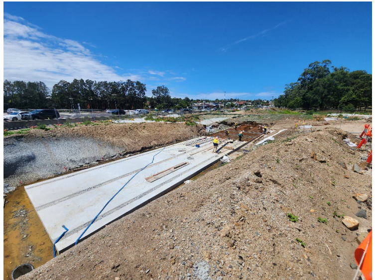
Image 4: Northern Interchange, the realigned Dark Creek culvert works. Southern side of Newcastle Road.
