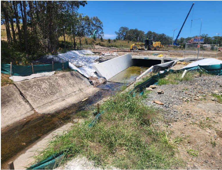
Image 1: Northern Interchange, view of the Dark Creek works on the northern side of Newcastle Road.
