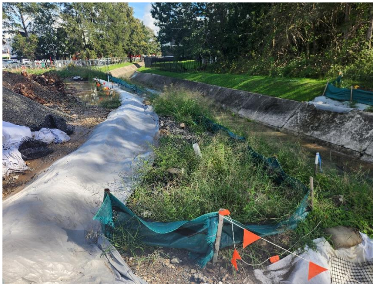
Image 3: Northern Interchange, view of the works on the Northern side of Dark Creek, behind McDonalds.
