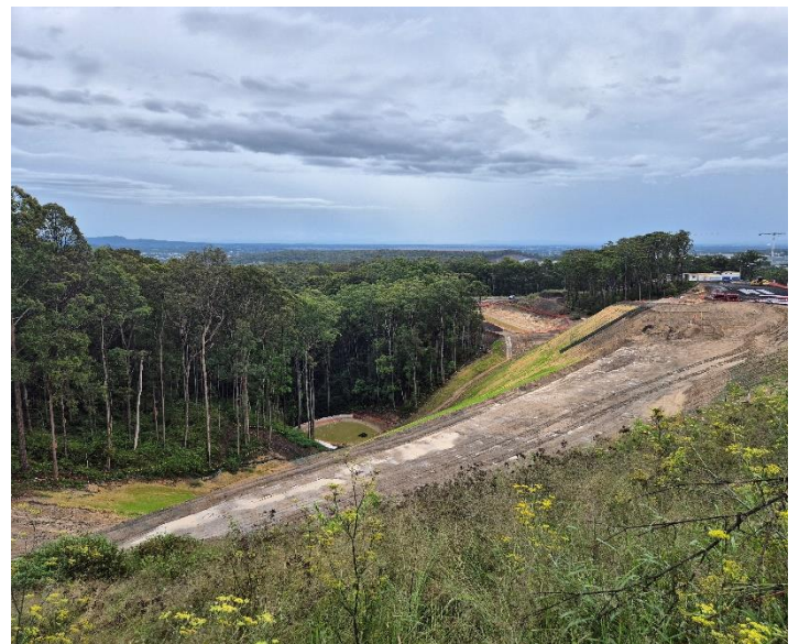
Image 8: View of the Southern Interchange looking north from Lookout Road. The light green on the batter is recent revegetation using MacMat and hydromulch.
