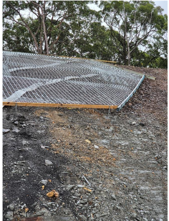
Image 6: Western batter on the mainline showing the formwork prior to application of shotcrete. No. 2
