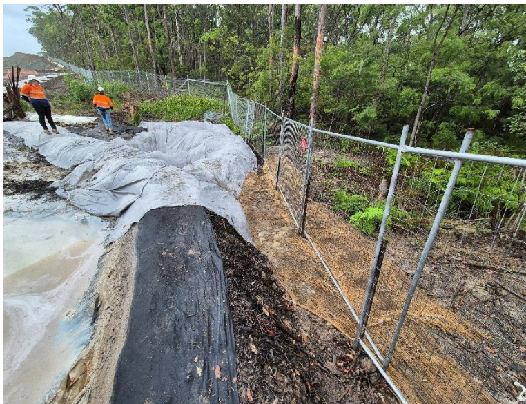
Image 7: Mainline near Creek 3 showing repairs to ErSed controls and remediation of surrounding area following major rain event.
