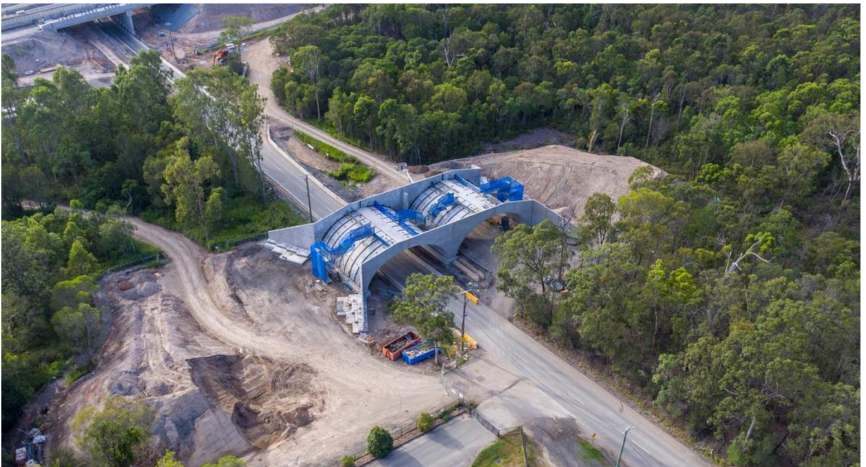
Figure 3-5 Example of a fauna overpass detailing the construction impacts at Illaween Street, Brisbane Fauna Crossing (Source Transurban Group)
