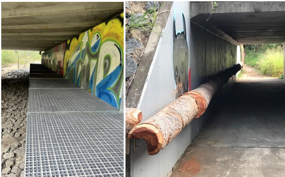
Figure 4-4 Examples of underpasses with fauna ledges, fiberglass ledge at Deadman's Creek Bridge, Heathcote Road (NSW) and natural log ledge under Pine Mountain Road, Salvin Creek (QLD). 18
