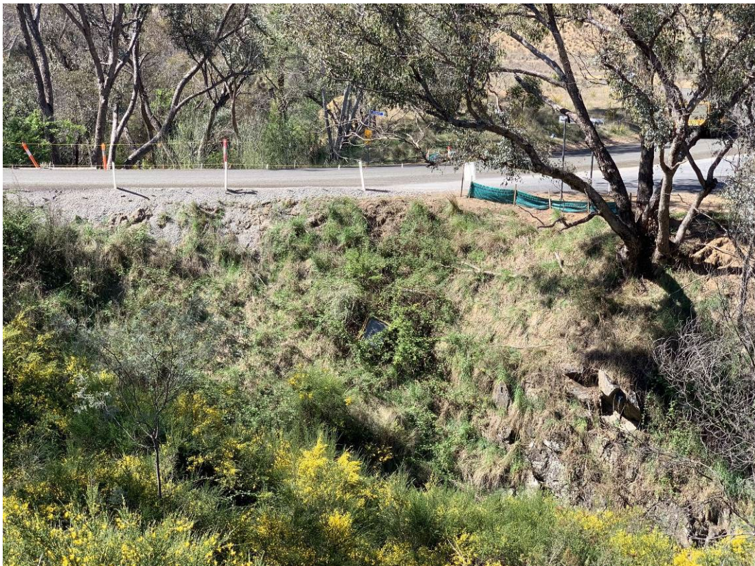
Photo 18: Captains Flat Road and Copper Creek Road intersection. Significant road upgrades and resurfacing have occurred on Captains Flat Road. Sediment silk screens are in place. A piece of construction signage appears to have fallen off the road towards Copper Creek.
