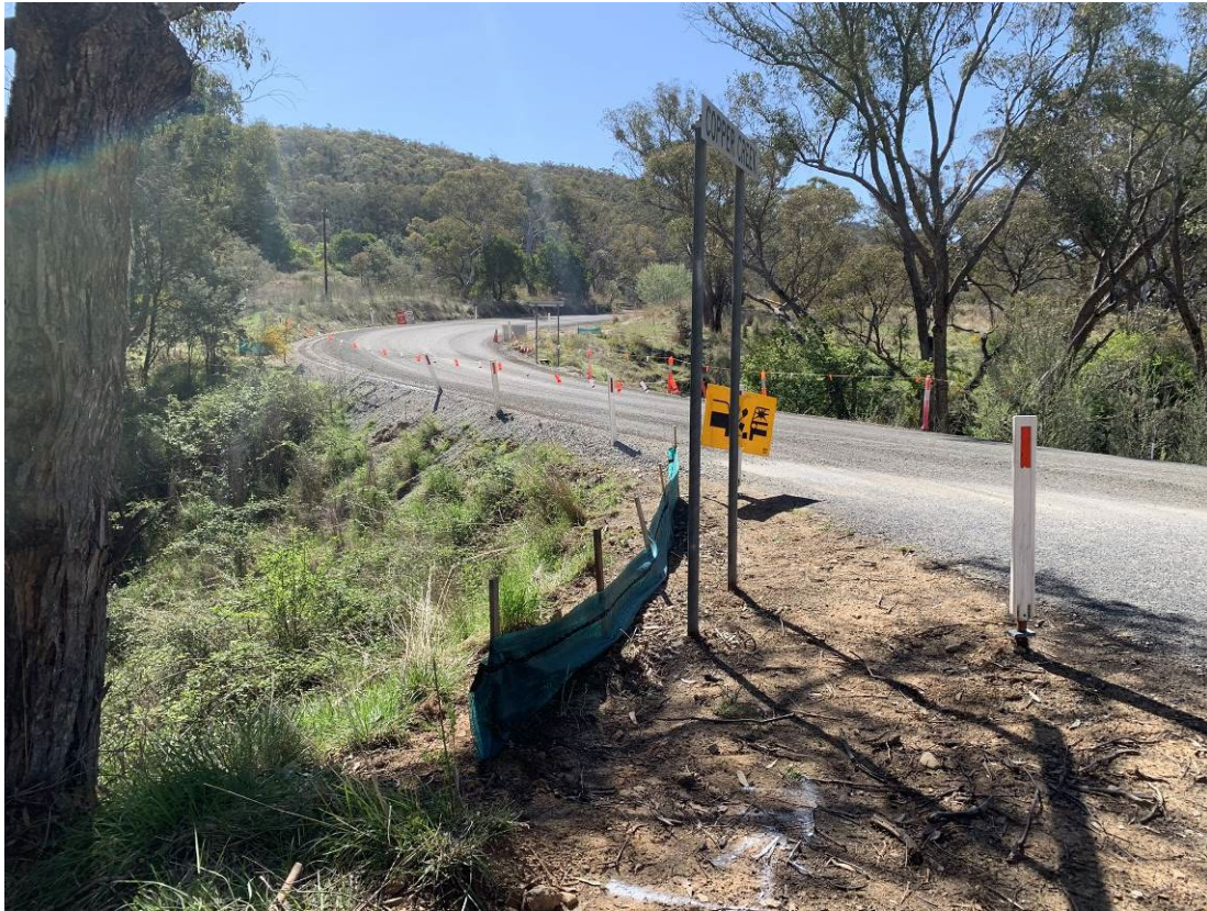
Photo 17: Captains Flat Road and Copper Creek Road intersection. Significant road upgrades and resurfacing have occurred on Captains Flat Road. Sediment silk screens are in place.
