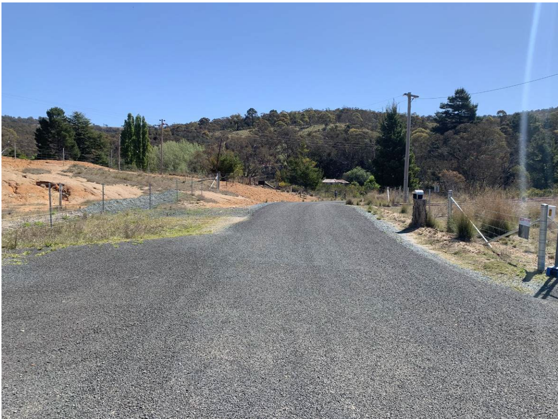
Photo 10: Sealed road over Copper Creek Road crossing, preventing inadvertent access to site materials underneath.
