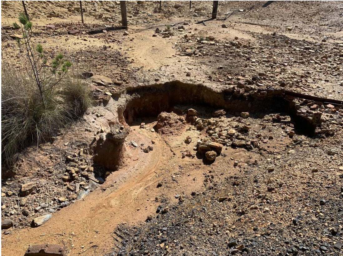
Photo 5: Evidence of erosion of soils on site. No evidence of current surface water runoff into Coppers Creek. Located south of the State Emergency Service (SES) facility.
