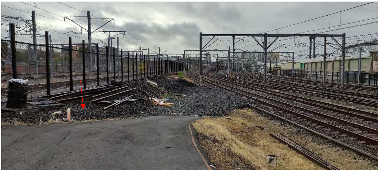
Plate 5.1: Photograph of the new turning bay and proposed new retaining wall (red arrow), looking east, south-east. (Source: Transport for Tomorrow, 2024)
