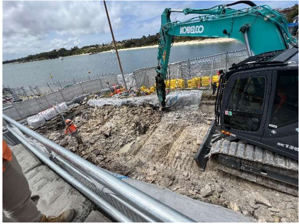
Photo LP12: La Perouse ramp construction - Site tightly constrained. Erosion and sediment controls in place.
