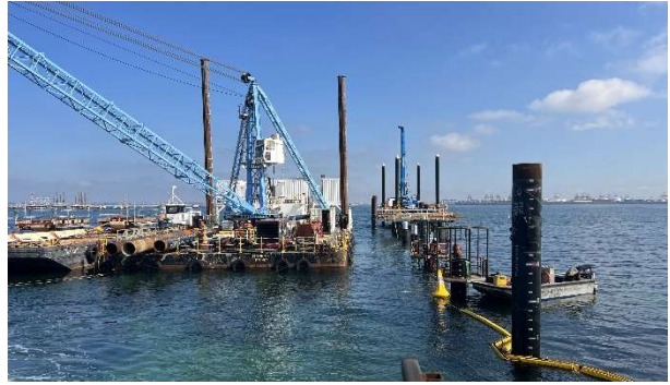
Photo K10: Piling Barge. Boom deployed around localised works. Spill kit observed upon the barge.
