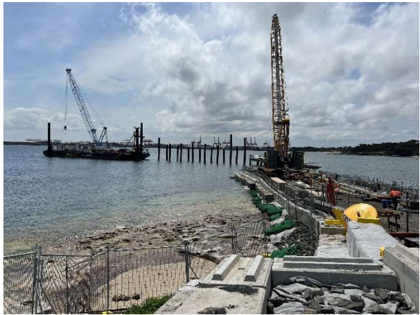
Photo LP10: La Perouse crane platform - Platform constructed upon the rock shelf. Rock shelf protected by geofabric and rock ballast. Piling and piling barge.
