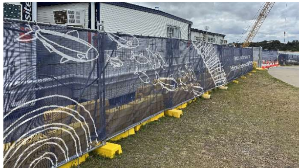
Photo LP2a and LP2b: La Perouse site compound - Boundary screen with local indigenous artwork. Site compound signage with project details.
