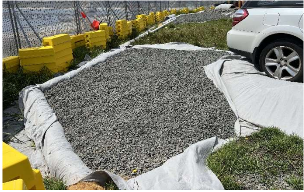
Photo LP8: La Perouse site compound – Soak aways and perimeter bunds as per the ESCP. Perimeter bunds rather than sedimentation fences were installed due to no-dig order.
