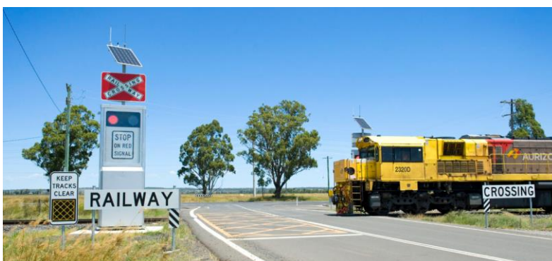
Figure 13: The RAXS System operating in Queensland.
