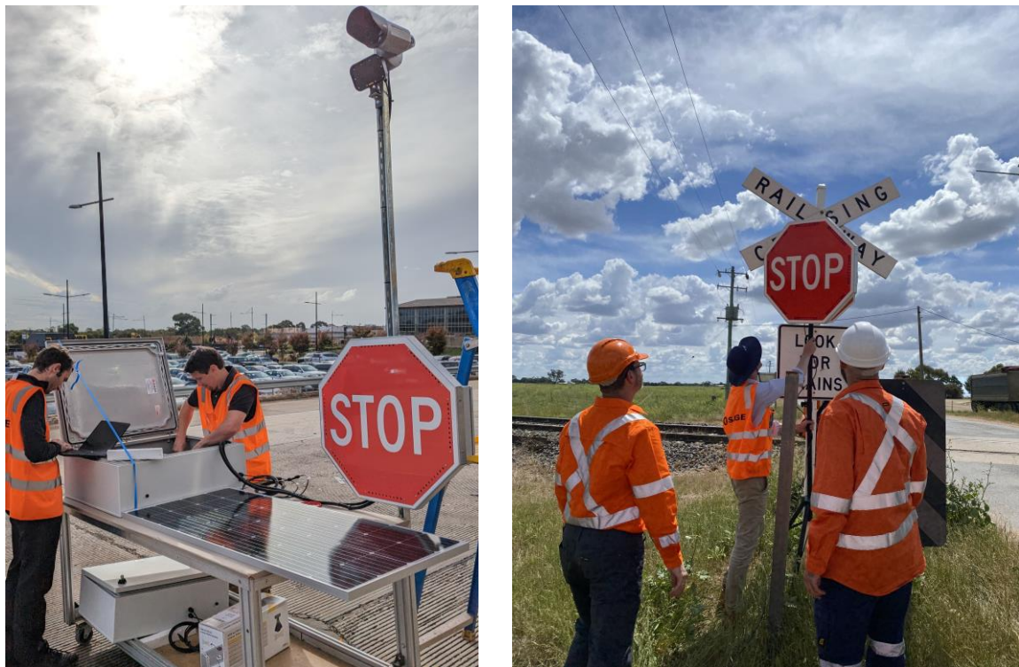
Figure 14: Onsite Installation of the Augmented Stop Sign trial.
