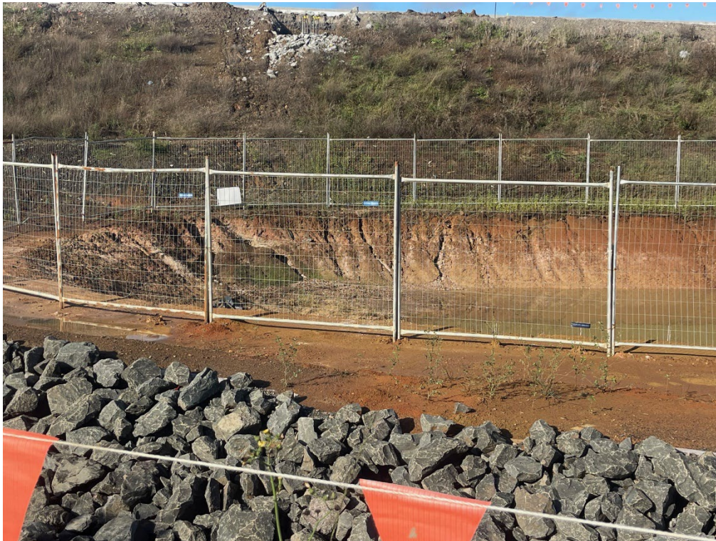
M12C-03-OBS-02 - Sediment basin 9 – rill erosion on basin batters.
