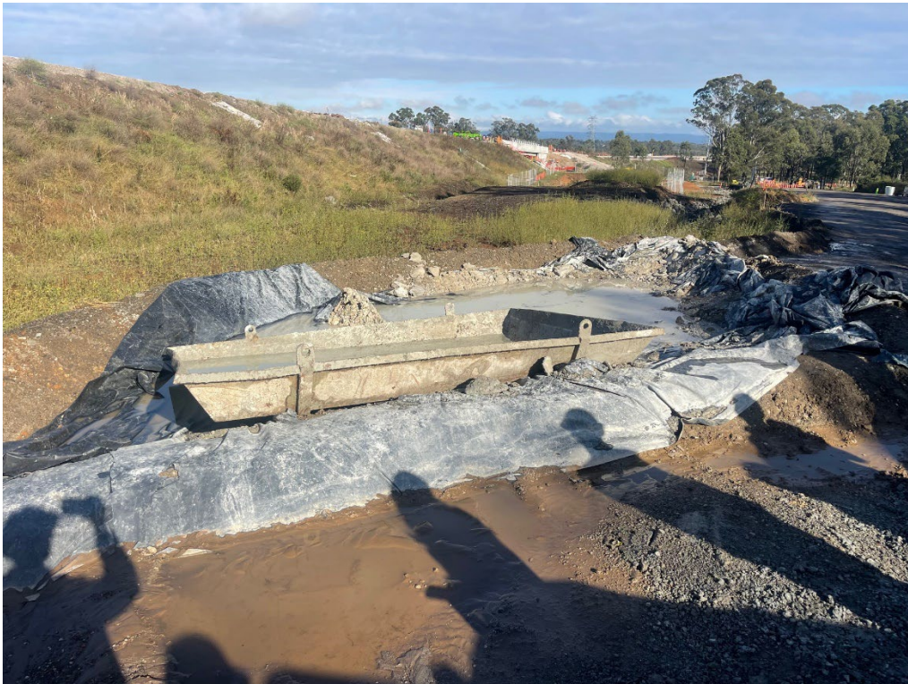
M12C-03- OBS -05 - Gate 5 – concrete washout location. Maintenance of plastic lining required.
