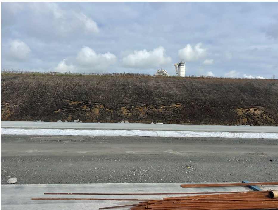
Cut 22 – showing slumping of batter and slippage of compost hydro mulch.
