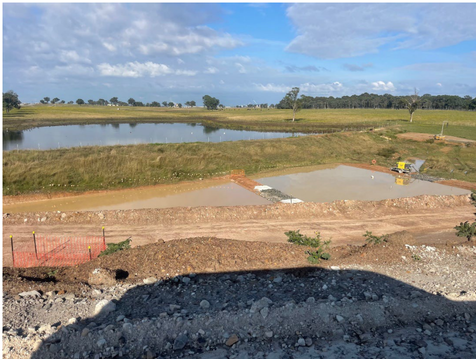
Permanent basin with overflow into rock channel.
