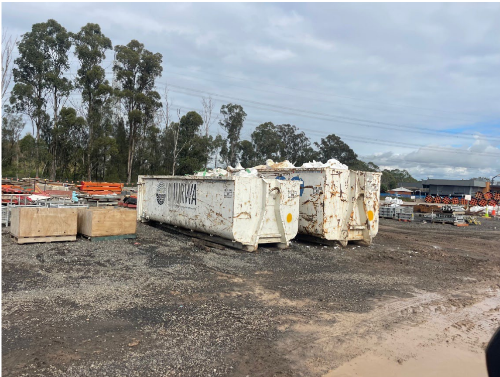
Gate 7 / Bridge 9 laydown area – waste bins at capacity.
