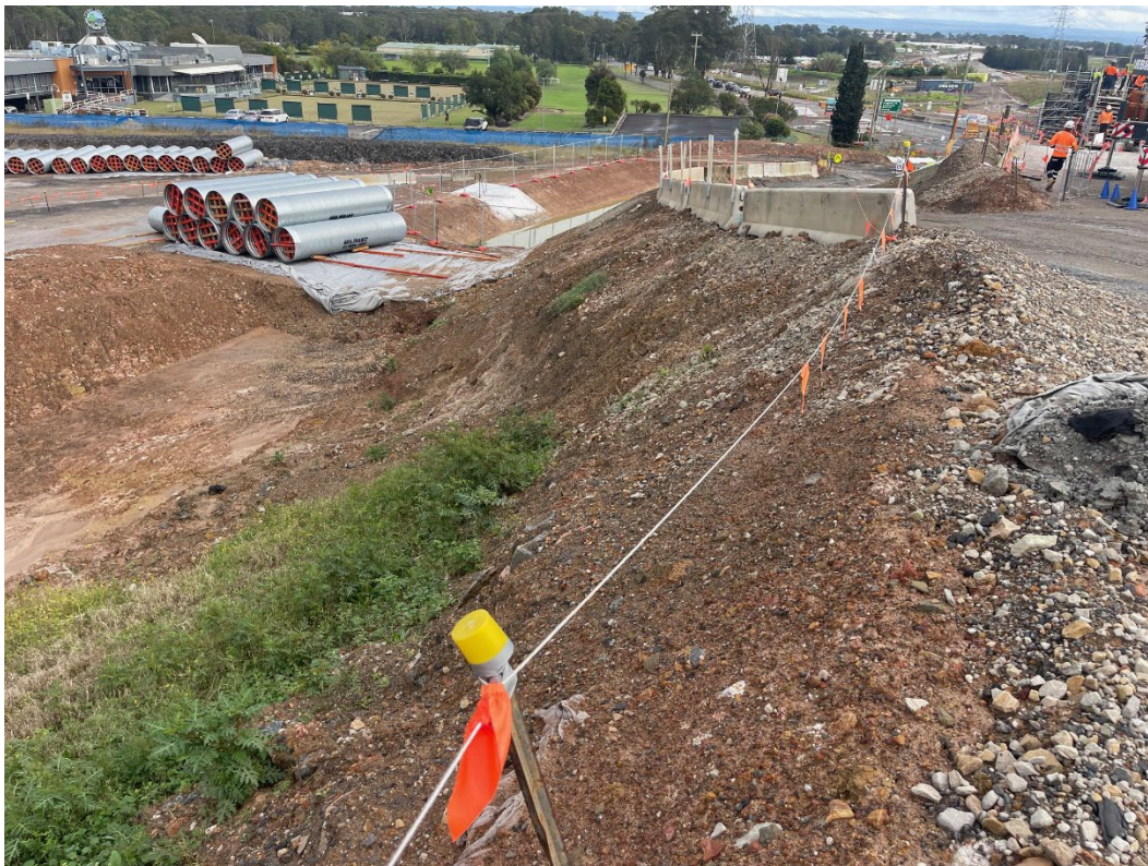
Bridge 9 – stabilisation of batter recommended.
