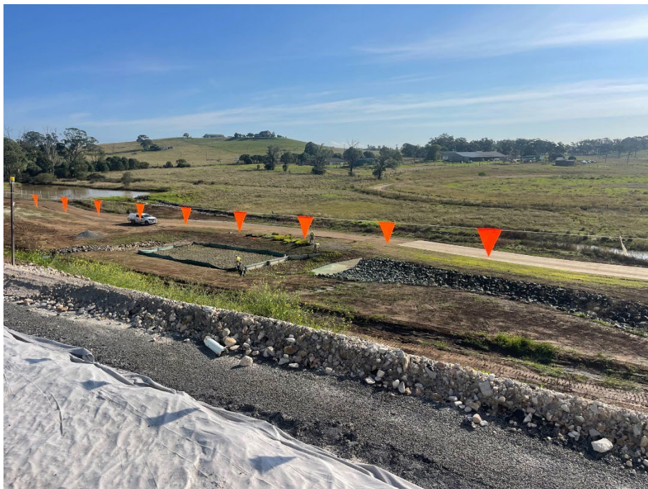
One of the four bioretention basins where organic pollutants are removed from surface runoff prior to discharge.
