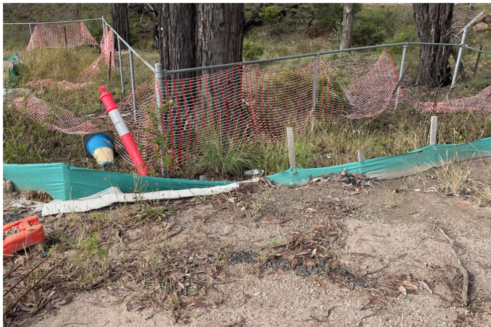
M12C-03- OBS -06 - Stockpile yard – sediment fence at capacity requiring maintenance.
