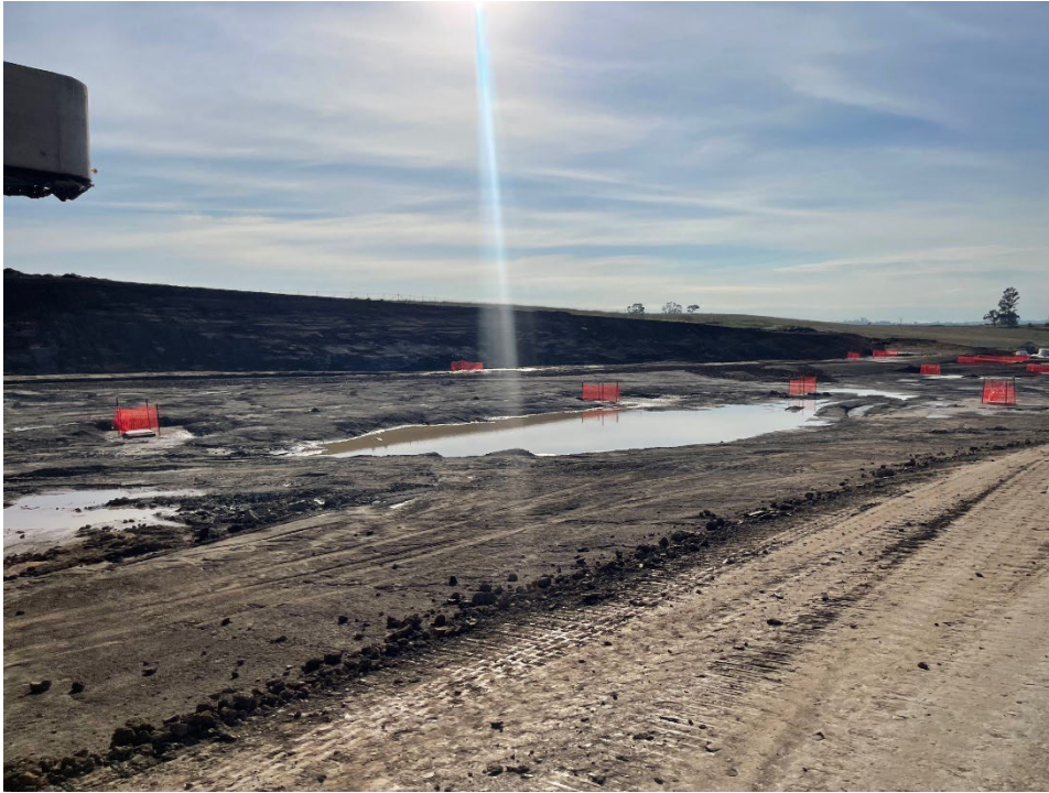
Low points within main alignment holding water from recent rainfall.
