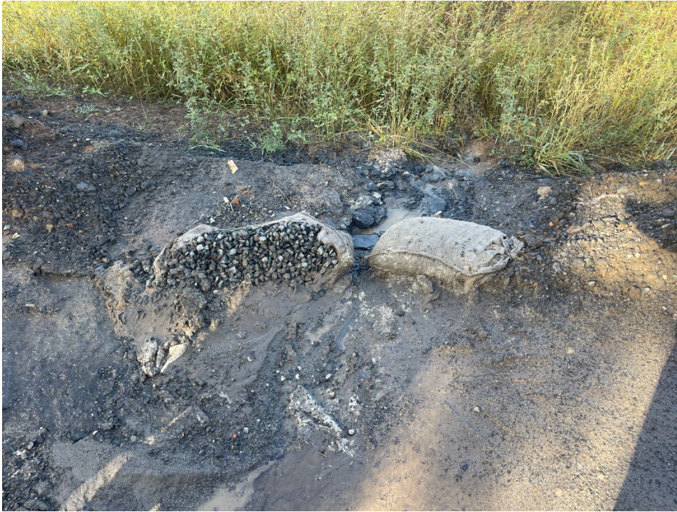
M12C-04-OBS-01 - Gate 5 – failed ERSED controls requiring replacement.
