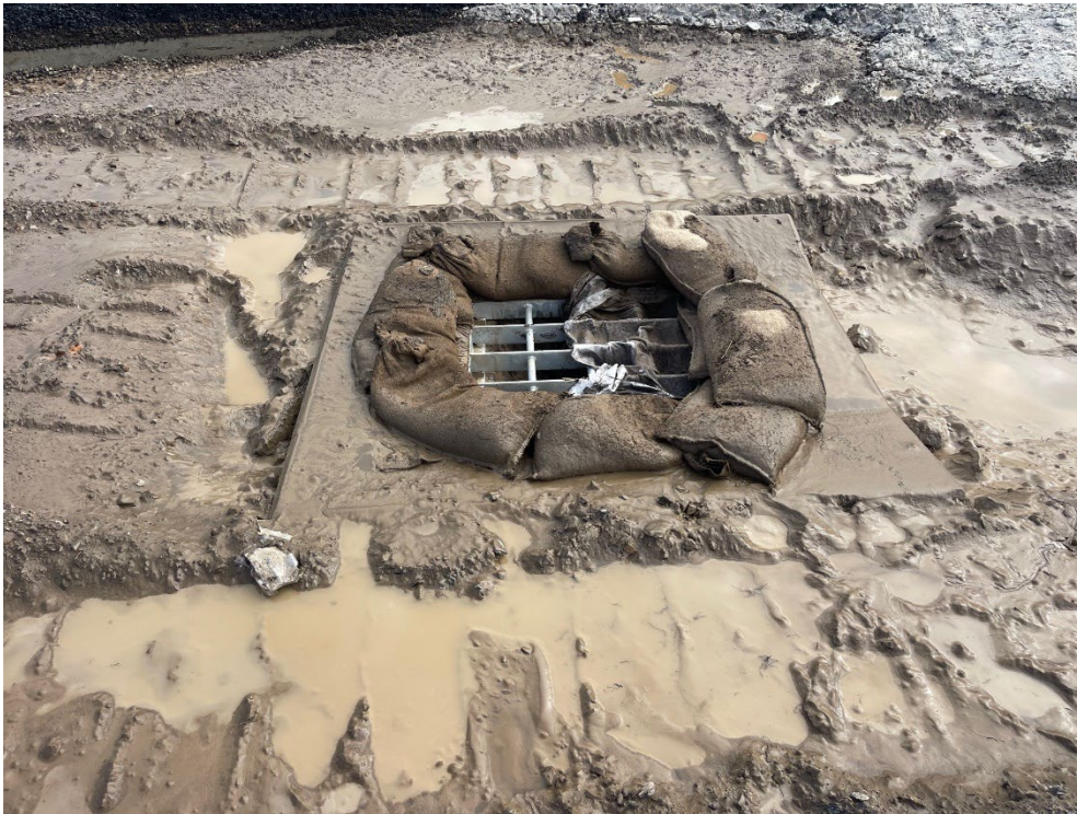
M12C-03- OBS -04 - Some stormwater pits requiring maintenance of ERSED controls.
