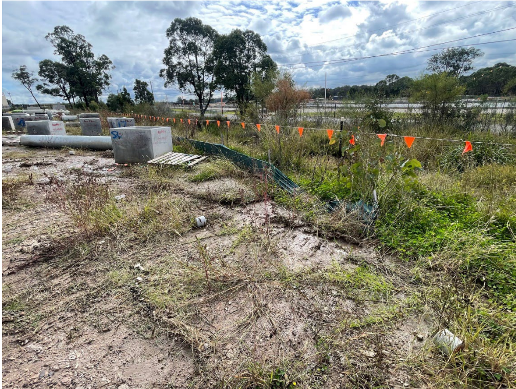
M12C-03- OBS -06 - Stockpile yard – section of sediment fence either completely failed or has been removed.
