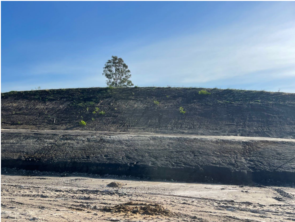
Cut batter where previous hydro seed product failed to germinate and take hold. Batters were being resprayed with a new seed product at the time of the audit.
