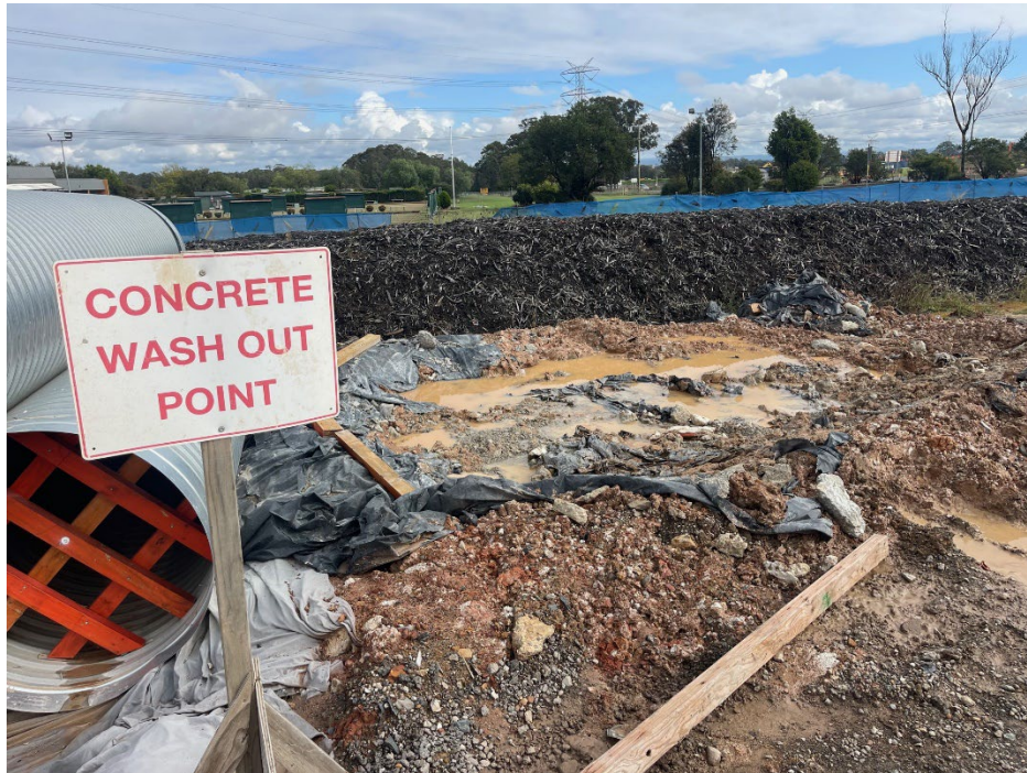
M12C-03- OBS -05 - Gate 7 / Bridge 9 laydown area – designated concrete washout location showing failure of containment bunds and plastic lining – requiring maintenance.
