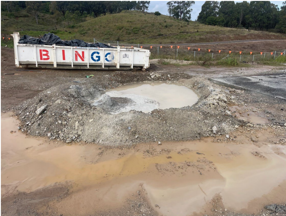
M12C-03- OBS -05 - Northern end of alignment - concrete washout area. No signage or plastic lining utilised.
