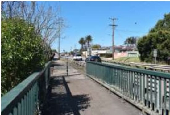
Figure 38: SE Pedestrian footbridge over Redbank Creek next to Bells Line of Road
