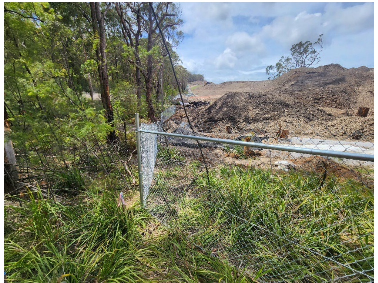
Image 4: Main line at Creek 2 fence has been repaired and ErSed controls reinstated as per Soil Conservationist advice.
