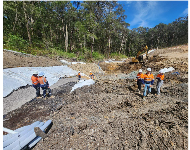
Image 6: Main line at Creek 3 (east) where repair works and headwall are being constructed.
