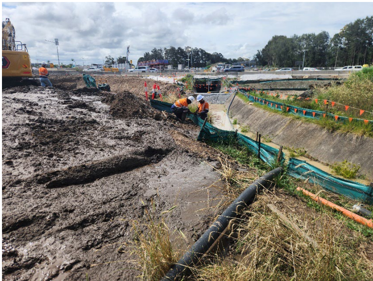
Image 7: Northern interchange, Dark Creek culvert extension works north of Newcastle Road. This part of Dark Creek has been taken offline and is acting as a sediment basin; it is not part of the Dark Creek culvert.
