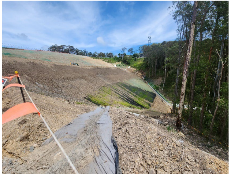
Image 2: Southern Interchange, view of the batter stabilisation and rehabilitation following the rain event. Repair work to be undertaken.
