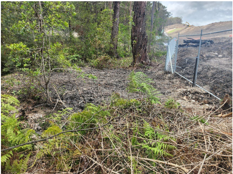
Image 3: Main line at Creek 2 clean-up of sediment from the rainfall event.
