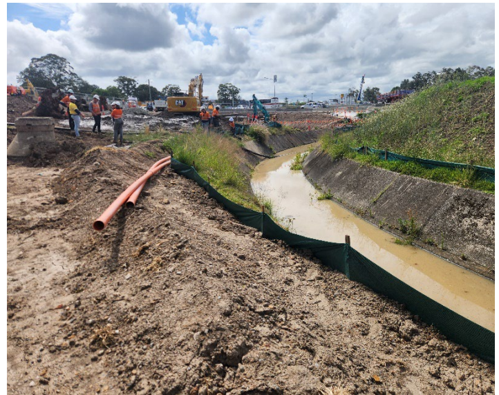
Image 8: Northern interchange, Dark Creek culvert extension works north of Newcastle Road. This part of Dark Creek has been taken offline and is acting as a sediment basin; it is not part of the Dark Creek culvert.
