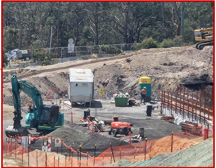
Image 2: Southern Interchange, close up view of the structure team working on bridge footings, adjacent to Lookout Road
