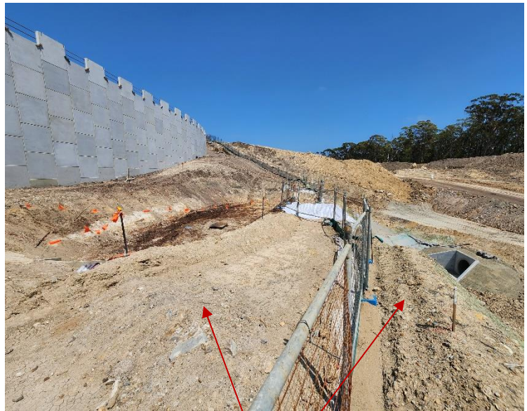
Image 4: Main line at the JHH / RP2J interface. JHH sediment basin under construction and RP2J clean water drain.
