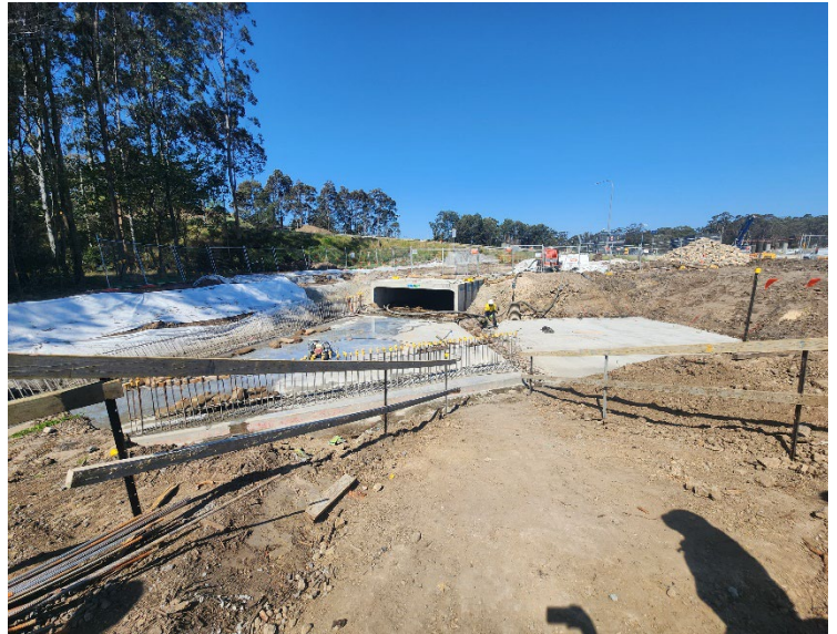
Image 2: View of the Dark Creek culvert works on the north western side of the Newcastle Road roundabout.
