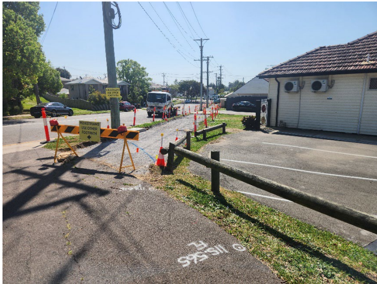
Image 3: New pathway along Illoura Street, Council works. Allows connection of temporary Shared Pathway connection.
