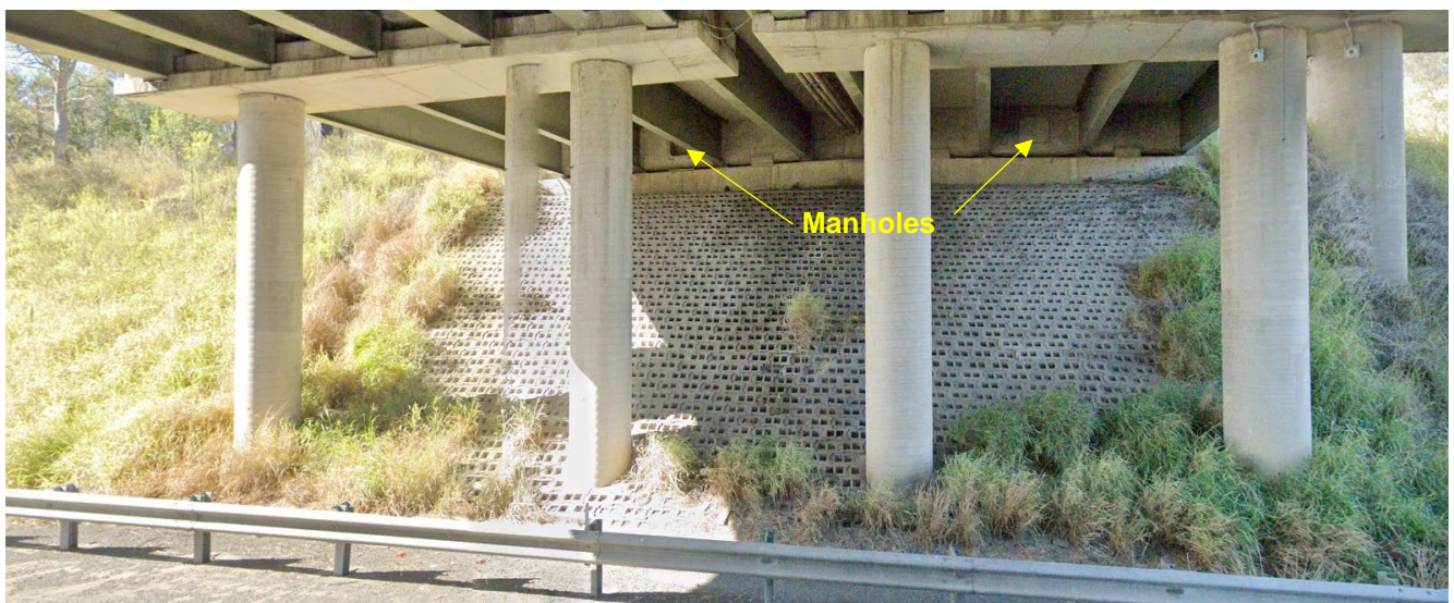
Note: the northern manhole cover appears to be missing Source: Google Street View, photo date May 2023
