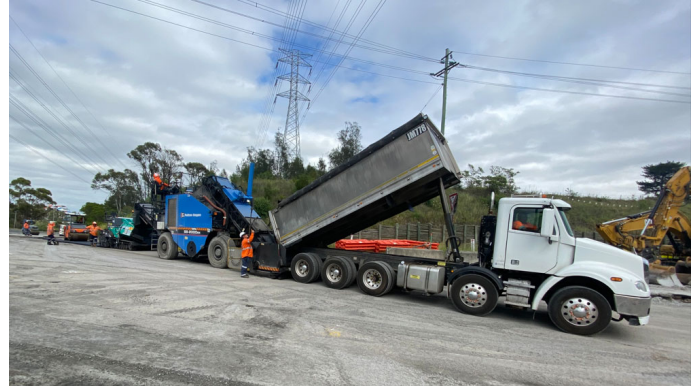
Pavement works on Prospect Highway at the newly upgraded M4 Motorway eastbound intersection.
