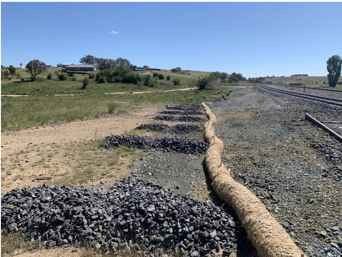
Photo 12: Rock checks running alongside former Woodlawn siding towards the middle culvert. No evidence of sediment build-up in rock armoury or Coir sediment control logs.
