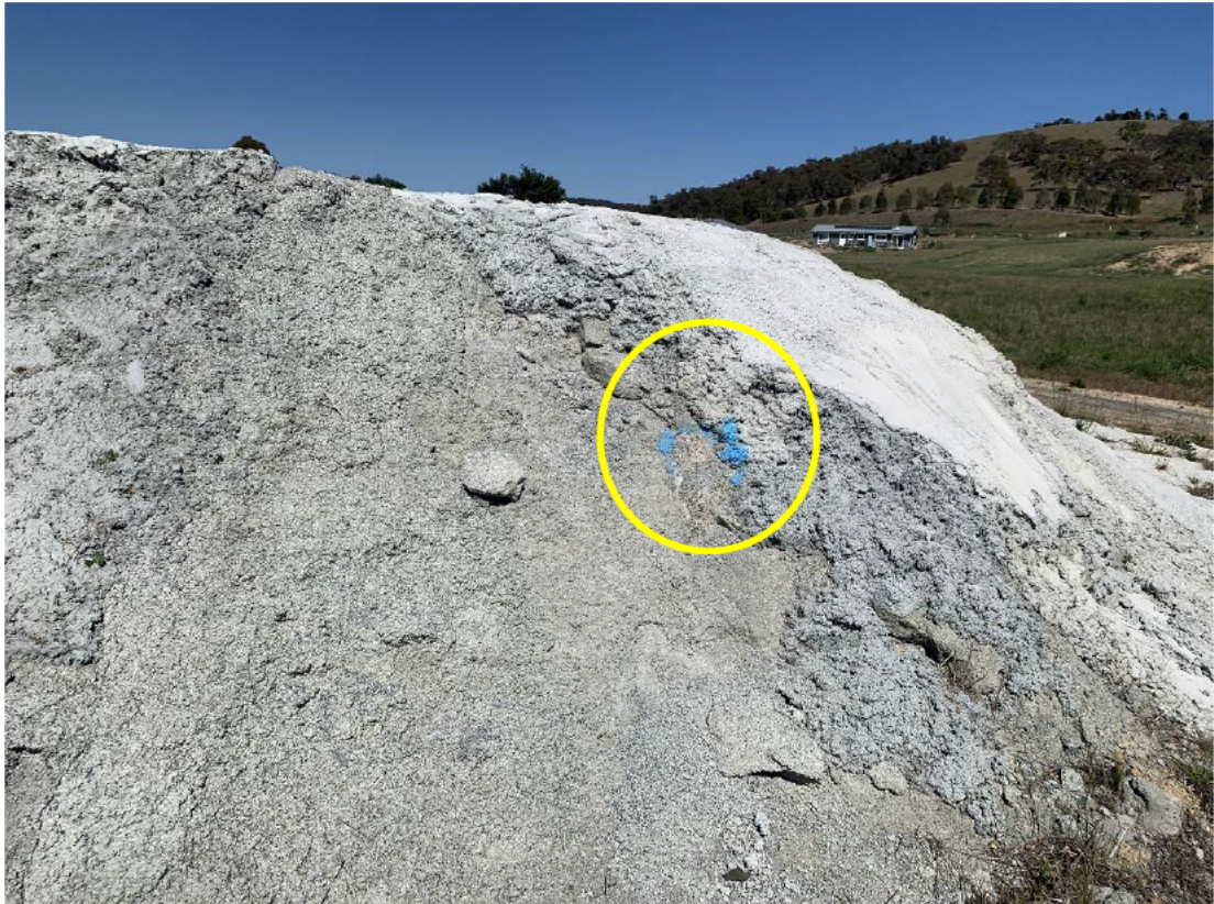
Photo 19: Exposed geofabric layer marker on main stockpile which was identified during the previous inspection (14/09/23), that has since been filled in with concrete. Repaired location indicated by yellow circle. Located on North-Eastern side of stockpile.
