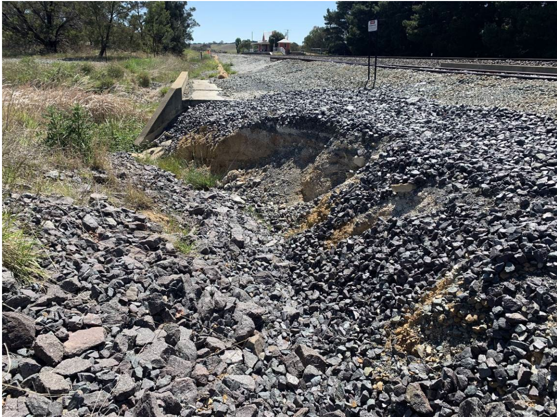
Photo 9: Visible evidence of erosion due to loss of ground cover (ballast material) upgradient of southernmost culvert. Remaining material is stable and no major further erosion is noted since last inspection. Facing north-east.
