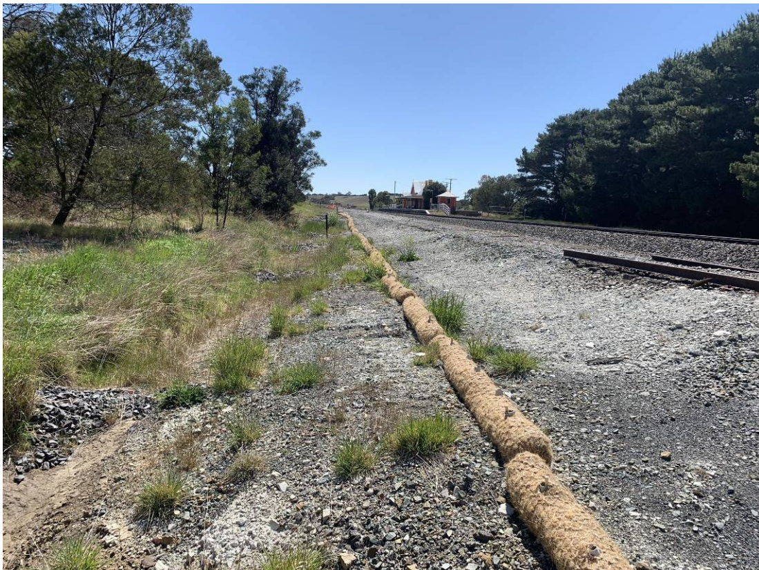
Photo 10: Upgradient of southernmost culvert showing Coir sediment control logs, used as control measures for sediment control. Facing north-east.
