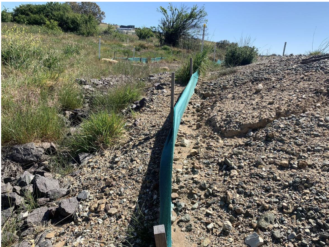
Photo 14: Upgradient of middle trainline culvert facing east. Silt fencing is clear with some sediment visible.
