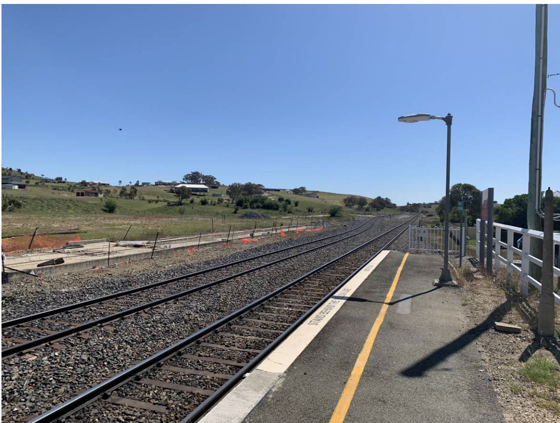
Photo 2: Picture at north-eastern end of Tarago railway station facing north-east. No airborne dust visible.
