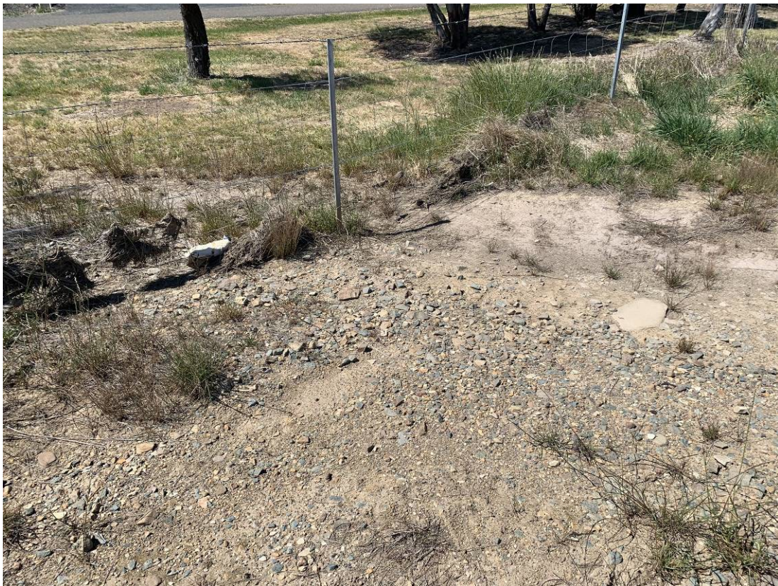
Photo 5: Downgradient of middle culvert. No water or damp soil found pooling adjacent to site boundary fencing compared to previous inspection (14/09/23). No surface water currently running off site at middle culvert.
