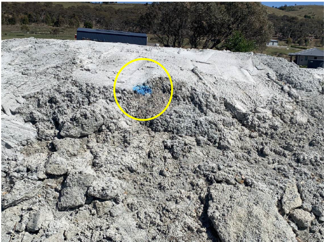
Photo 20: Exposed geofabric layer marker on main stockpile which was identified during the previous inspection (14/09/23), that has since been filled in with concrete. Repaired location indicated by yellow circle. Located on South-Eastern side of stockpile.
