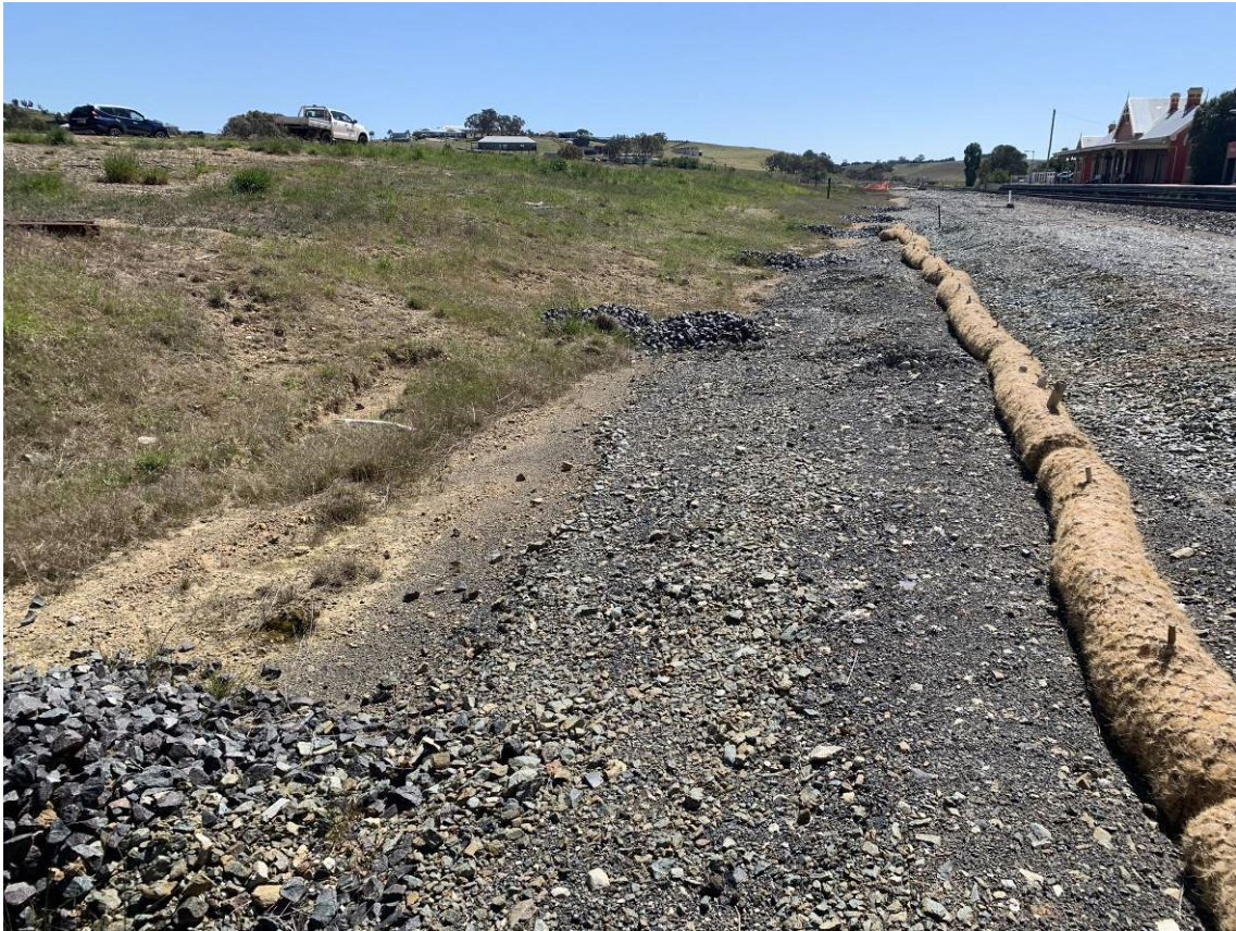
Photo 11: Rock checks running along former Woodlawn siding and between southern and middle culverts. Silt fencing replaced by Coir sediment control logs.
