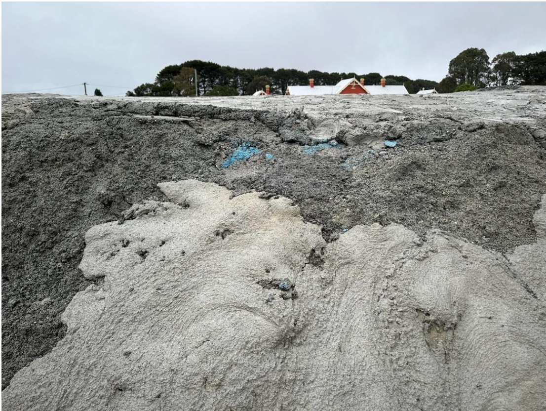
Photo 14: Location of previous stockpile capping that was visible and then covered with cement. Cement mixture appears to have sufficiently covered area and been maintained for an extended period of time even with rainfall.
