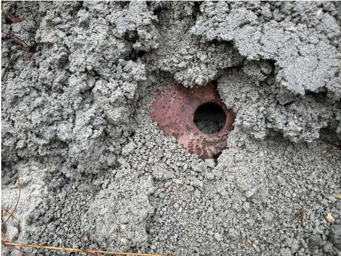
Photo 13: Geofabric marker layer visible in stockpile capping underneath metal plate. UGL Representatives on site advised of location.
