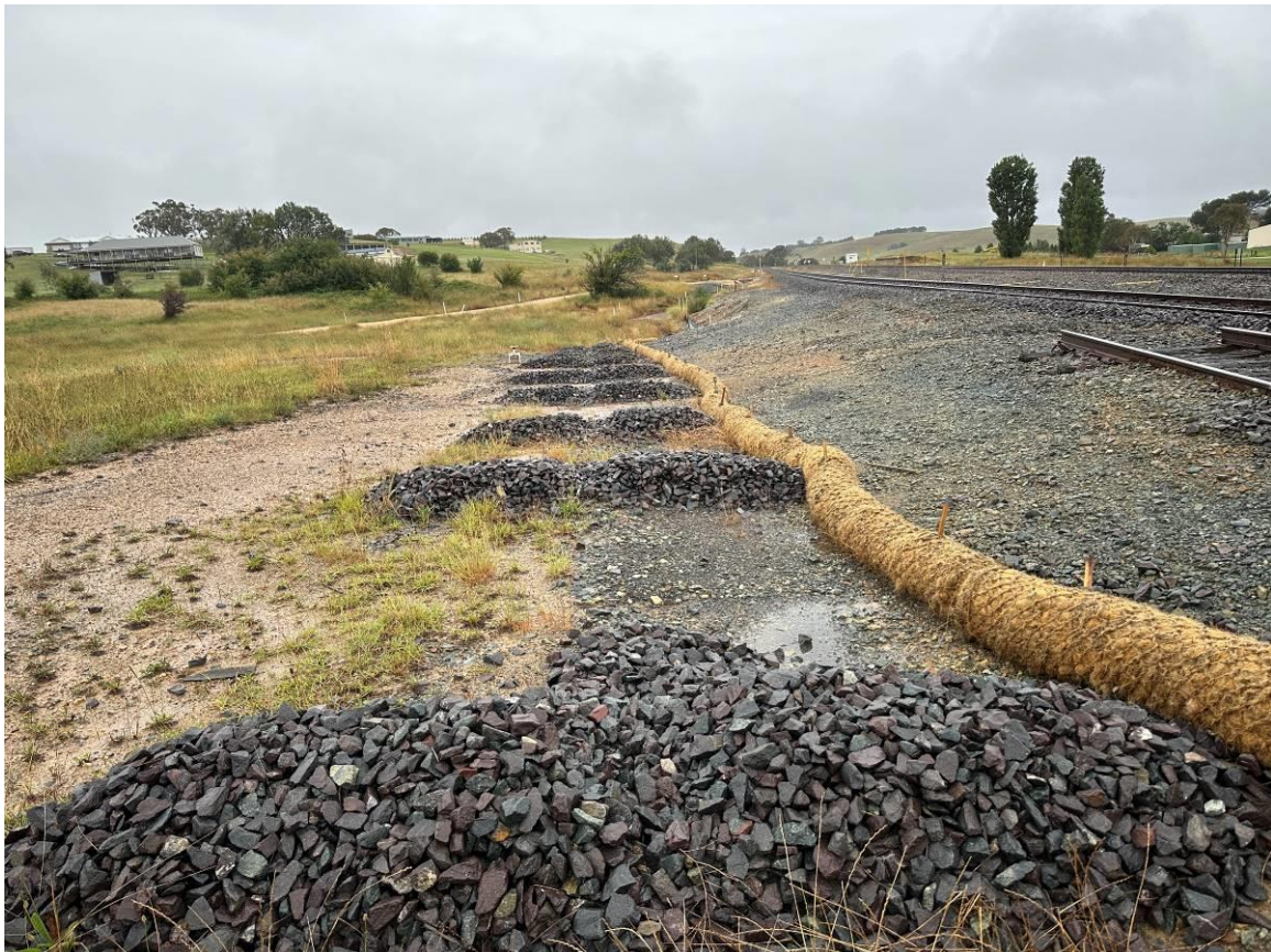
Photo 8: Upgradient of middle culvert with no flowing surface water. Sediment control rock armour appears in good condition.
