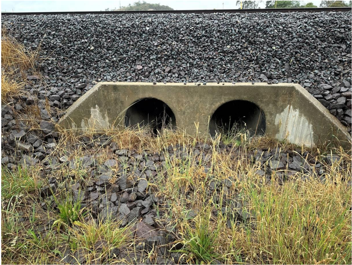
Photo 11: Upgradient of northernmost culvert. No surface water flowing through culvert. Minimal sediment build up on rock armoury.
