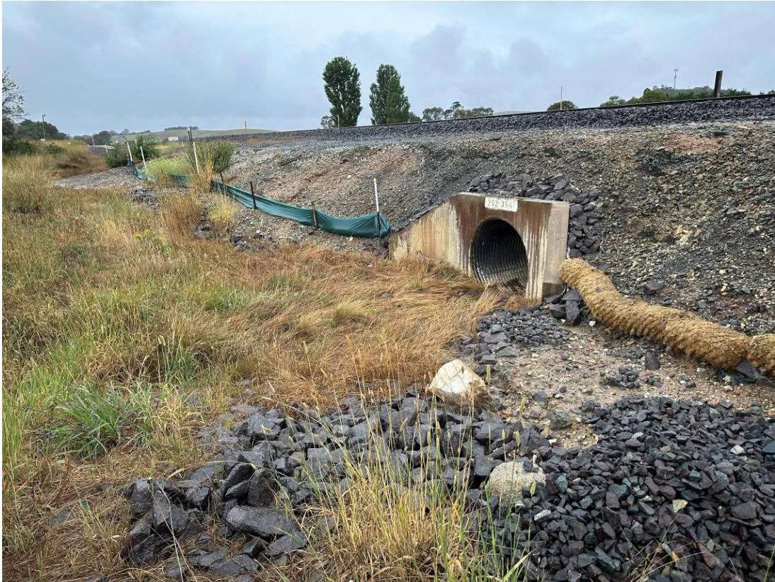
Photo 9: Upgradient of middle culvert upgradient of the railway line with no flowing surface water. Minor observed build-up of sediment fencing.
