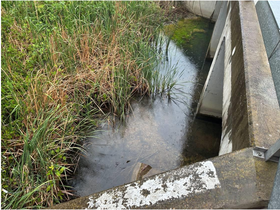
Photo 3: Downgradient of southern culvert with surface water flowing offsite. Surface water is clear with low turbidity.
