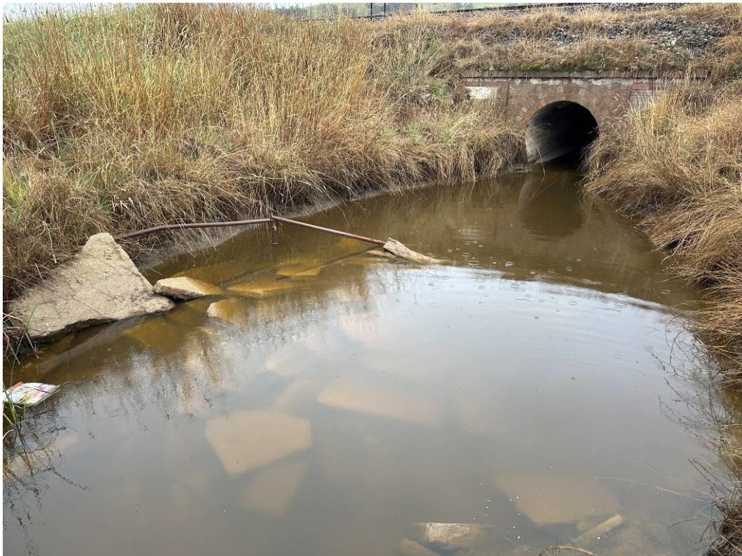
Photo 6: Downgradient of middle culvert with pooled surface water. Surface water was clear with low turbidity.
