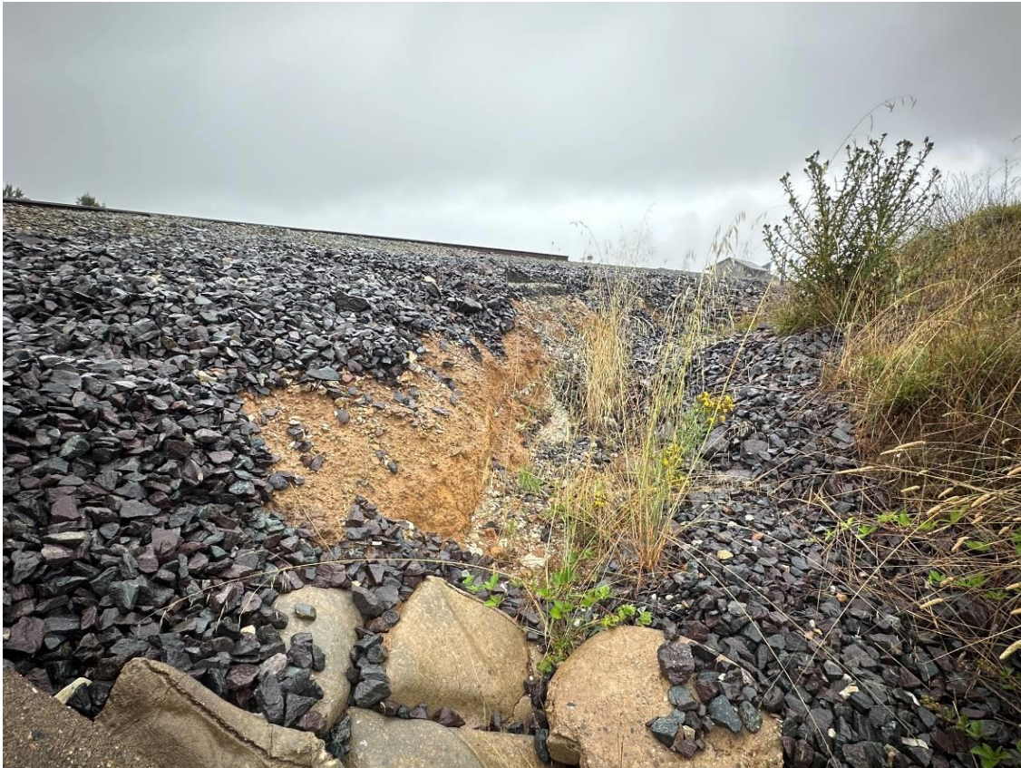
Photo 15: Visible evidence of erosion due to loss of ground cover (ballast material) upgradient of southernmost culvert. Remaining material is stable and no major further erosion is noted since previous inspections.
