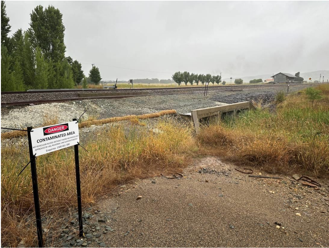
Photo 5: Upgradient of southern culvert showing coir sediment control logs and reed bed vegetation with natural sediment control.
