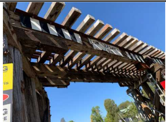
Span 7 missing centre girder & corbel above pier 6
