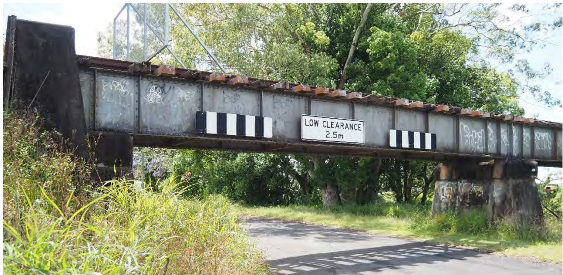
Figure 7-1 Crane Street low clearance 2.5 m (Source: FBE)
