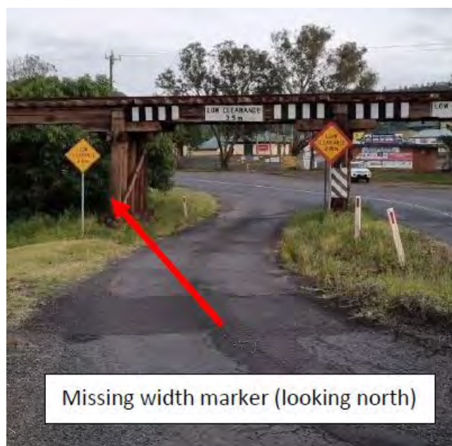
Photo 27: Missing width marker – Winterton Parade viaduct eastbound
