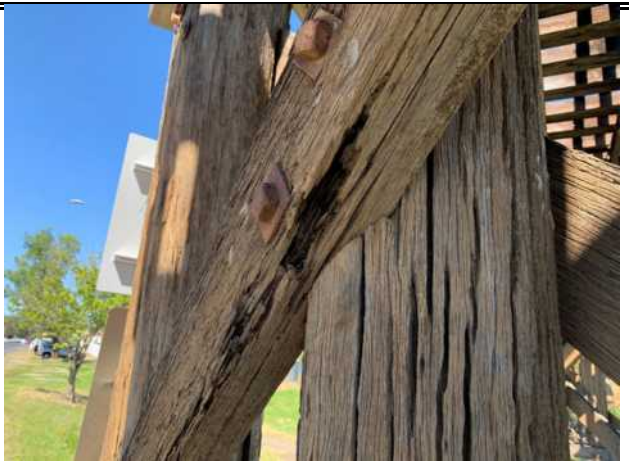
Pier 4 north diagonal brace hollow & evidence of white ants centre of brace
