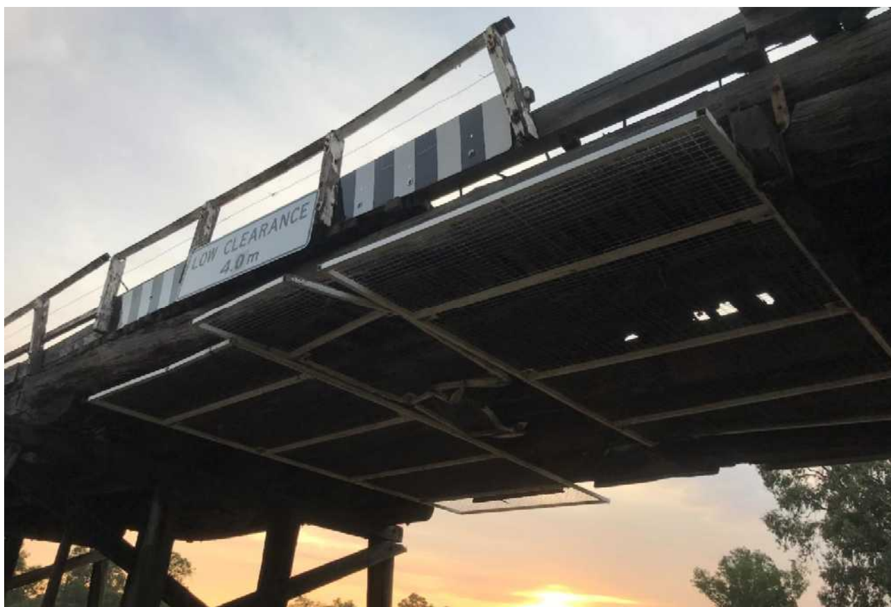
Example of Underbridge Protection (Gundagai, NSW). Note middle panel has been struck resulting in displacement
