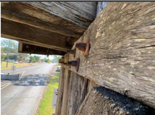
Pier 7 capwales on south side have minor 20mm sag
