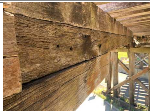
Span 5 centre girder weathered and minor 20mm sag
