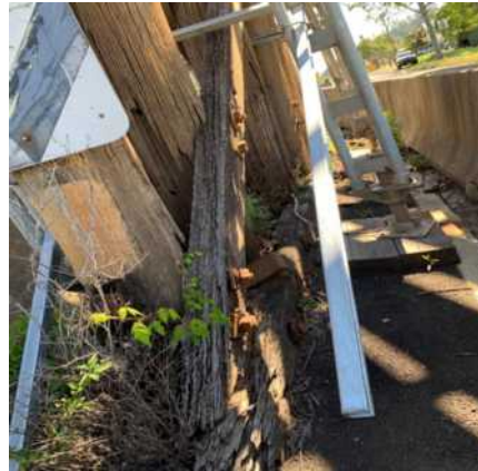
Pier 6 north diagonal brace rotted on lower end
