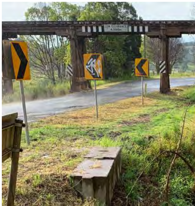
Photo 23: Vandalised signs – Winterton Parade viaduct
