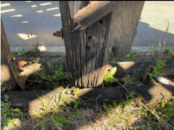
Pier 5 east pile hollow & rotted at base of pile
