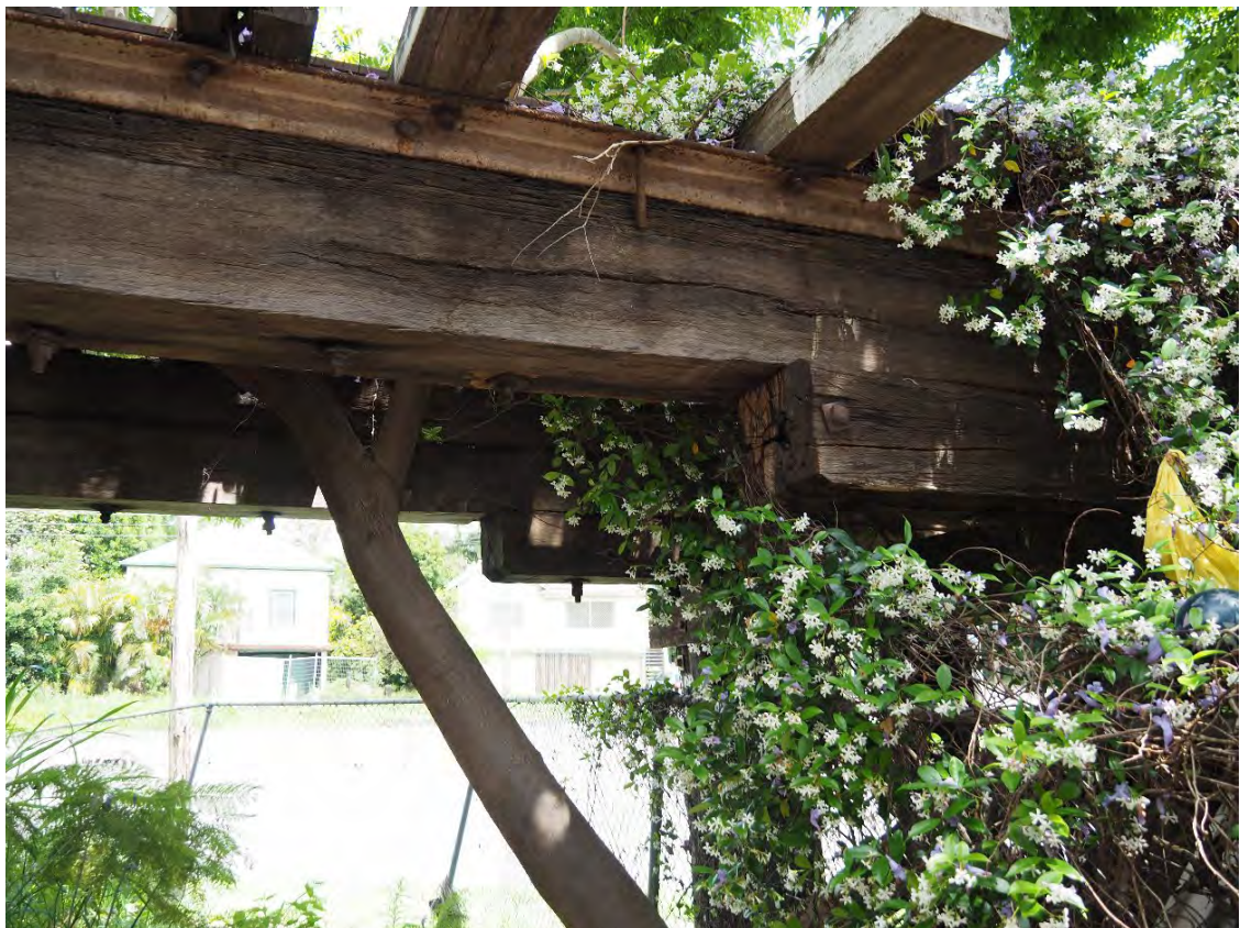
Figure B-20 Union Street – West elevation, typical timber girder condition (Source: FBE)
