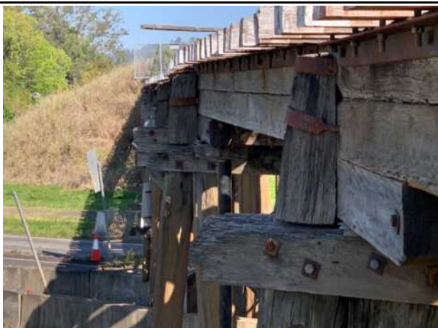
Top of piers 6 & 7 moved to the east from vehicle impact
