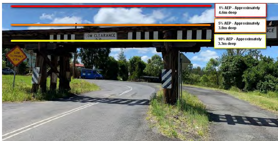
Figure 3: Alexandra Parade Bridge with Flood Depths
