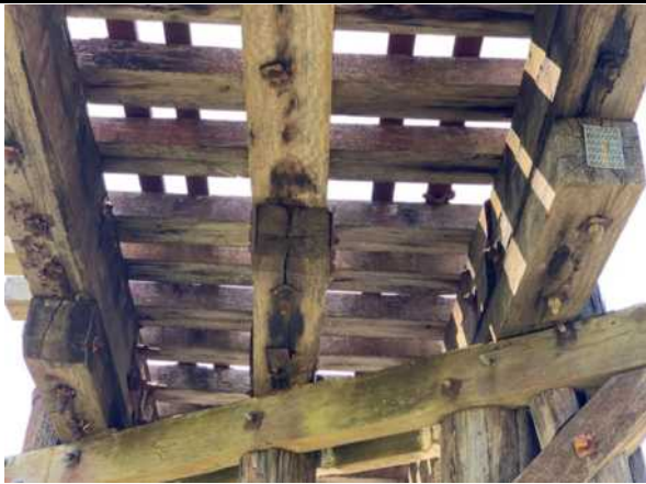
Pier 4 south end of corbels minor splits
