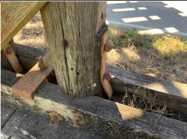
Pier 4 west pile hollow at base of pile
