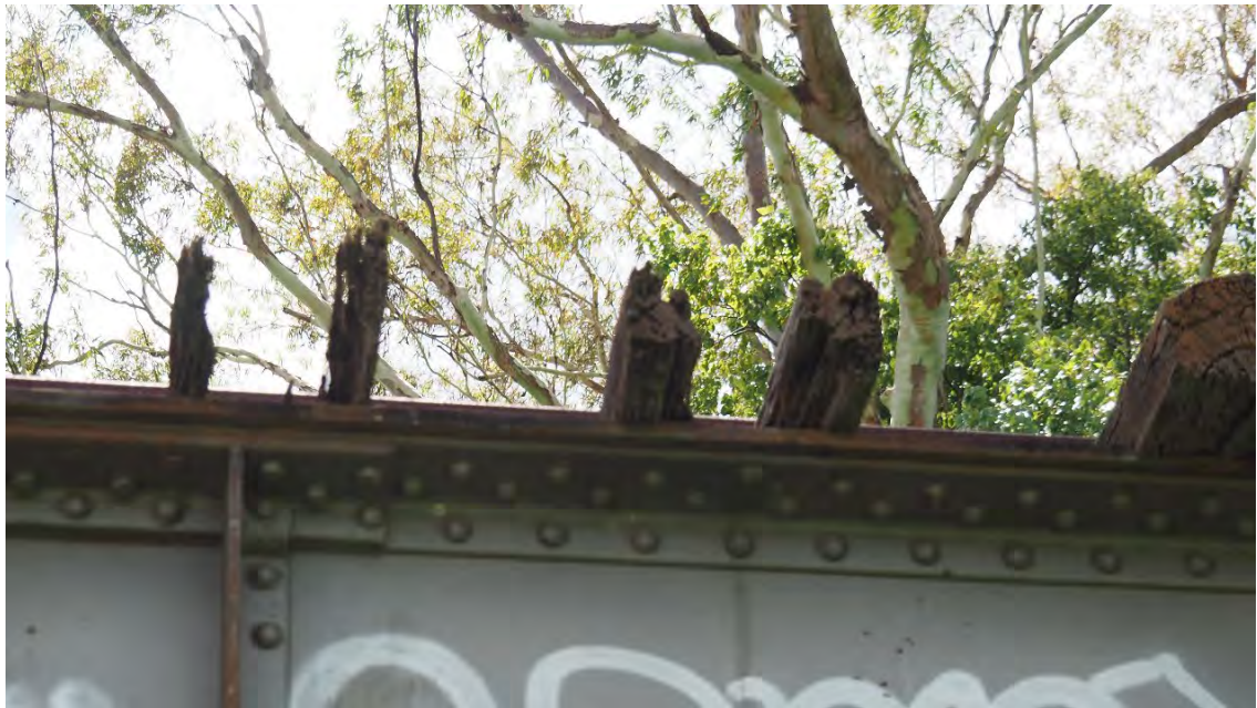
Figure B-10 Crane Street – Decayed transoms at Span 1 (Source: FBE)
