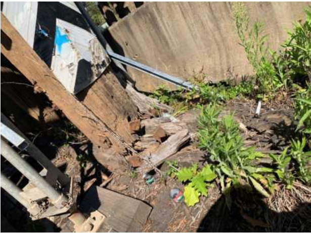
Pier 6 west spur pile broken and moved from vehicle impact
