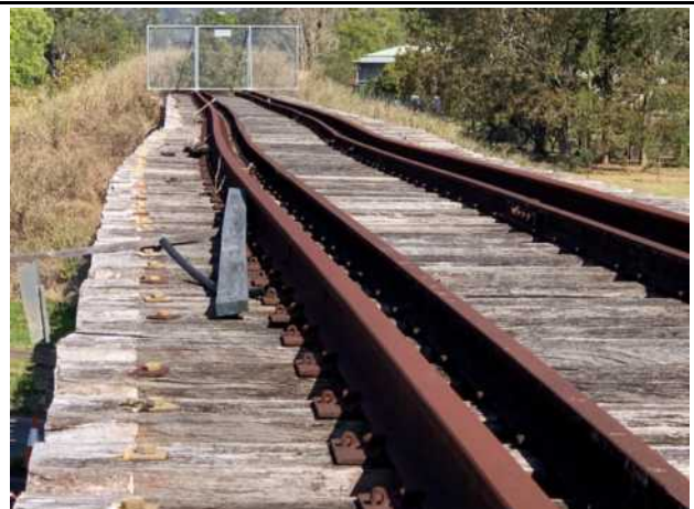
Bend in rail lines and sleepers above piers 6 & 7
