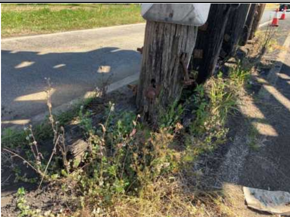
Pier 5 bottom capwales rot and weathered on east end
