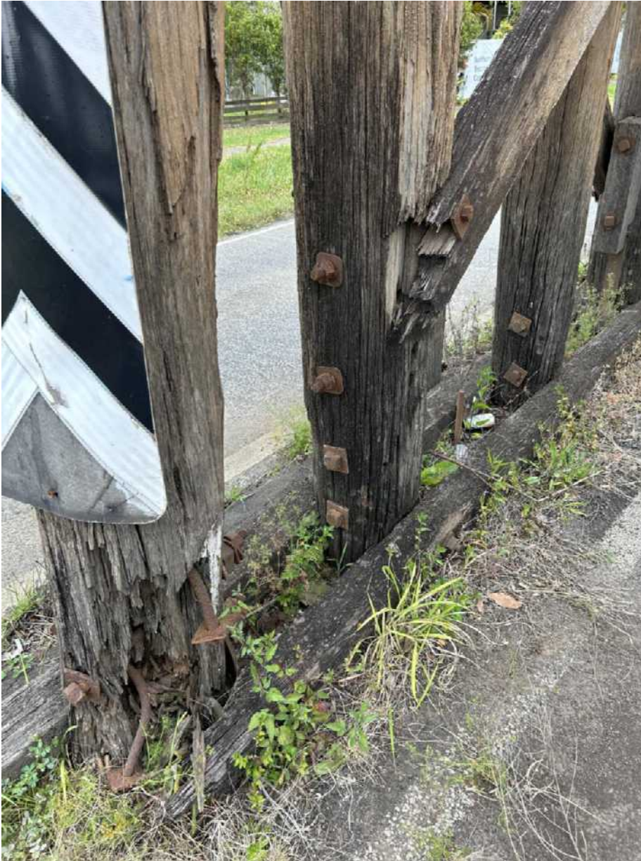
Figure 3: Pier 5 - Inclined post rotted
