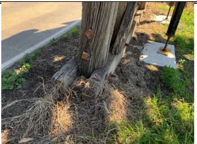
Pier 7 bottom wales weathered east end
