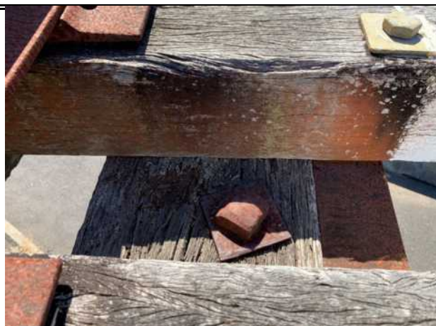
All spans have top section of transoms rotted
