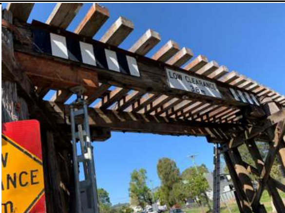
Span 6 centre girder missing
