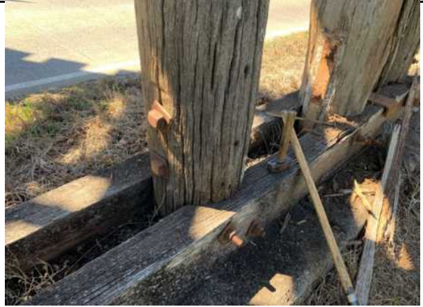
Pier 4 centre pile hollow at base of pile
