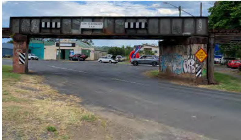
Photo 1: No edge lines - Union Street viaduct
