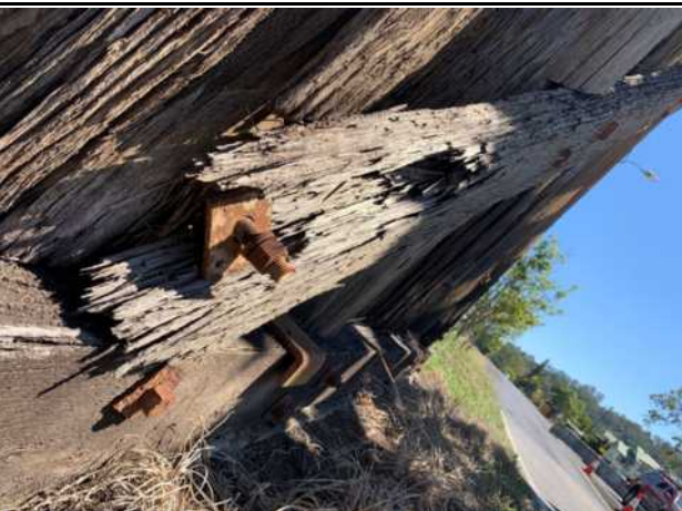
Pier 4 north diagonal brace rot and weathering on lower east end
