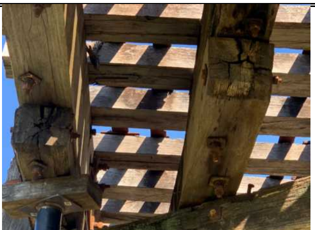
Pier 7 east corbel split & crushed
