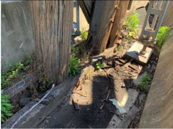
Pier 6 bottom capwale rotted & collapsing northside
