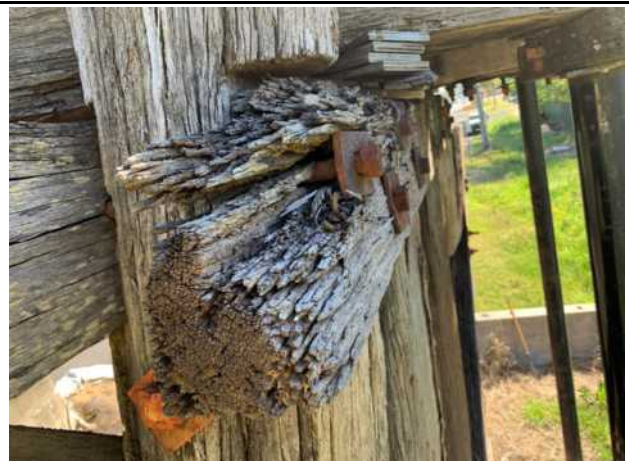
Pier 7 top capwales rot and weathered north side
