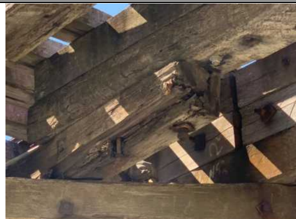
Pier 5 centre corbel southend split and damaged from vehicle impact
