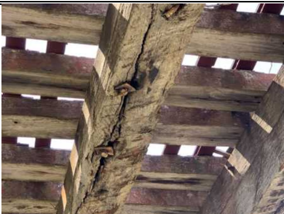
Span 5 centre girder longitudinal crack from vehicle impact
