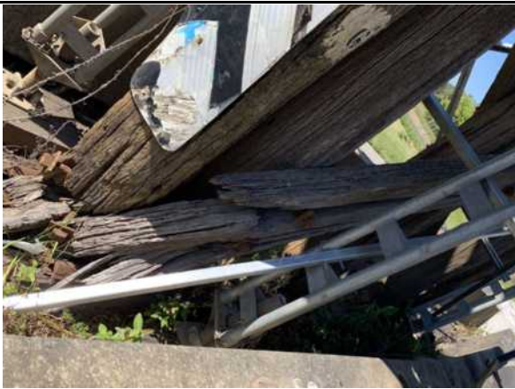
Pier 6 southern diagonal brace broken from vehicle impact
