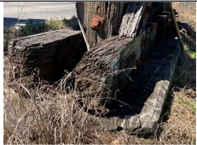
Pier 4 bottom capwales ends weathered west end
