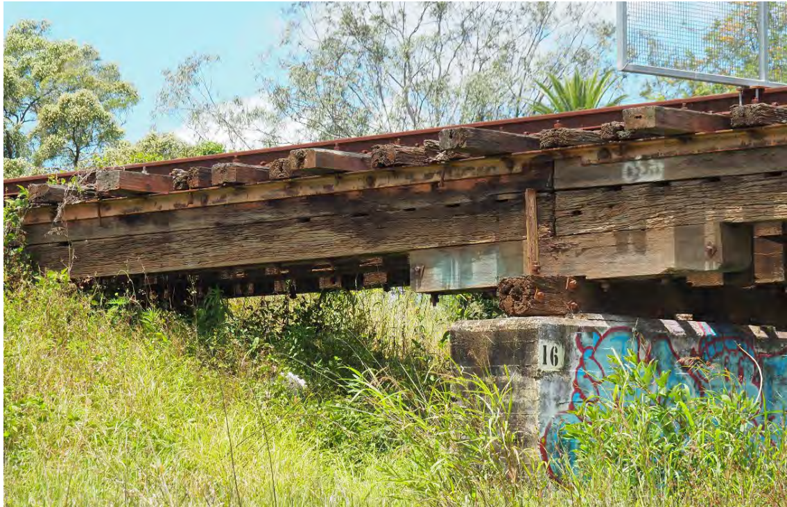
Figure B-5 Alexandra Parade – Decayed and infested transoms at Span 27 (Source: FBE)
