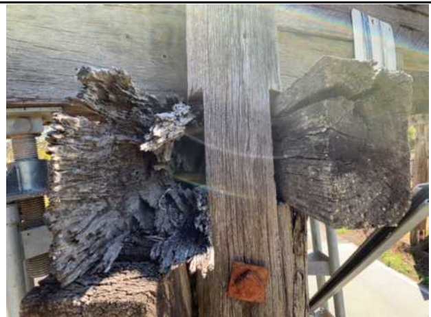
Pier 6 top capwales rot and weathered east end
