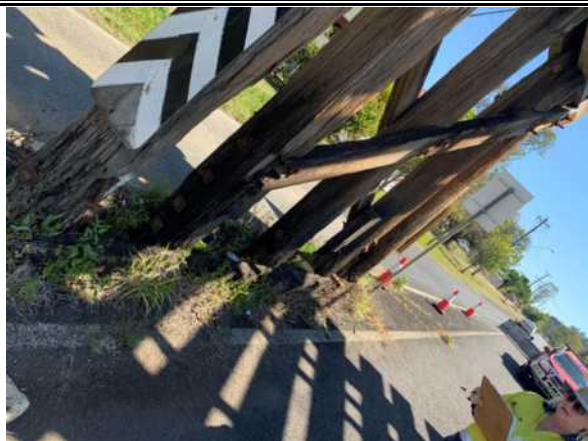
Pier 5 north diagonal brace broken lower end
