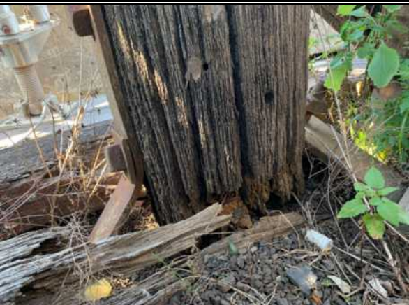
Pier 6 east pile rotted at base
