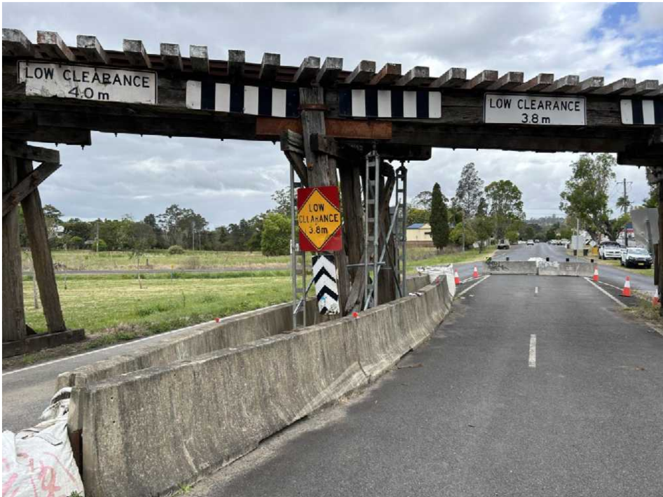
Figure 4: Pier 6 – Props and pier not vertical
