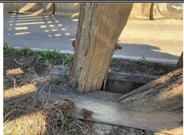
Pier 7 east spur pile hollow at base of pile
