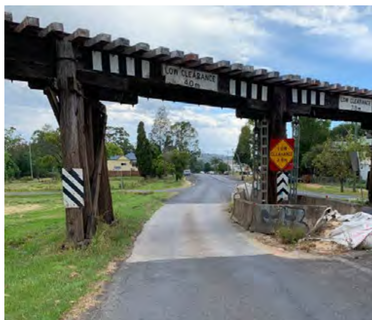
Photo 9: No edge lines - Terania Street viaduct
