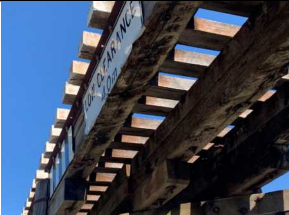
Span 5 east girder has vehicle impact damage centre of girder
