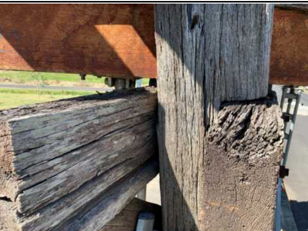
Pier 6 top capwales weathered west end
