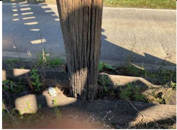
Pier 5 centre undersized pile hollow at base
