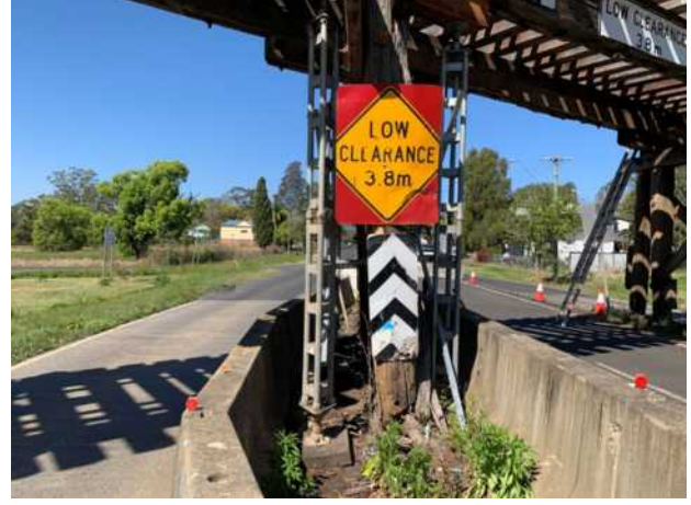
Pier 6 west end not vertical 300mm - leaning to north end of bridge
