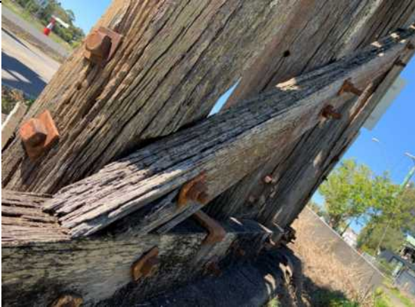
Pier 4 south diagonal brace rot and weathering on lower west end
