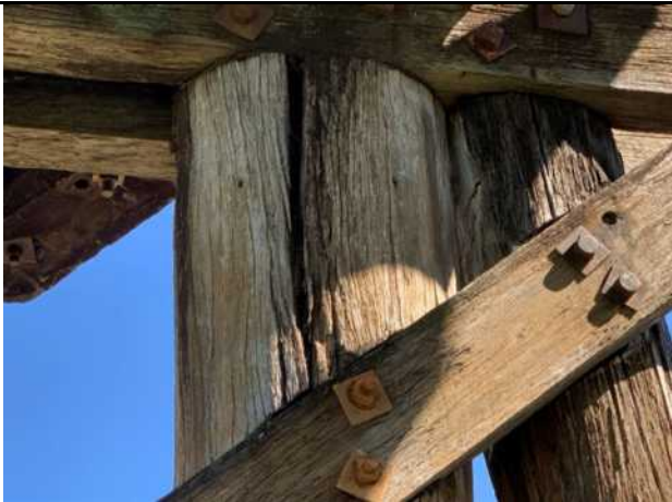
Pier 7 top of west pile split & evidence of white ants
