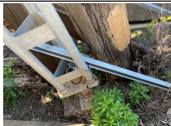
Pier 6 bottom capwale rotted & missing southside
