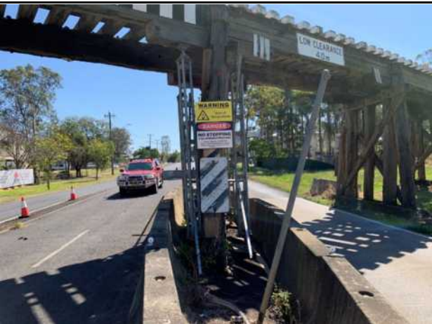
Pier 6 east end not vertical 300mm - leaning to north end of bridge
