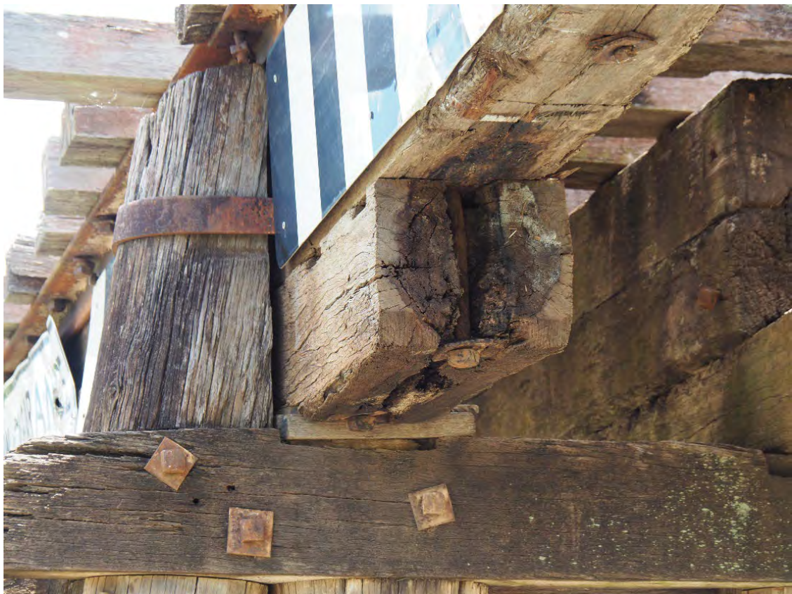
Figure B-4 Alexandra Parade – Rotten/Infested corbel, typical condition (Source: FBE)
