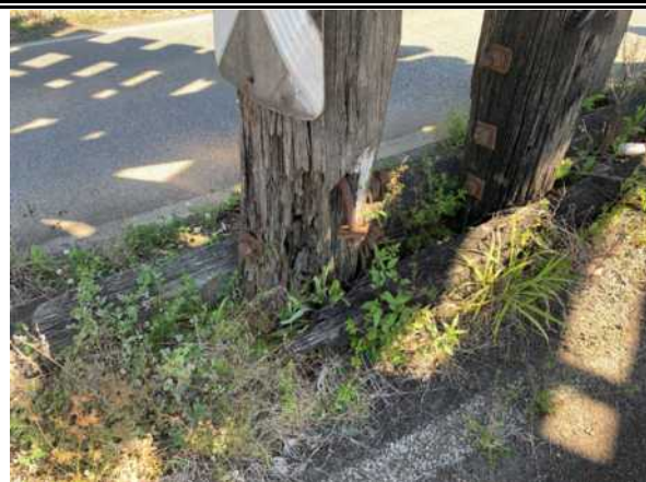
Pier 5 east spur pile rotted, hollow & damaged at base
