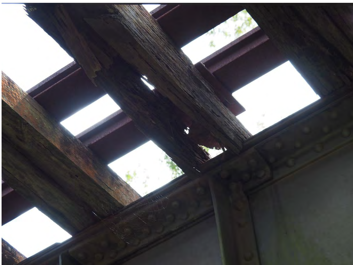
Figure B-9 Crane Street – Decayed transoms at Span 1, typical condition (Source: FBE)
