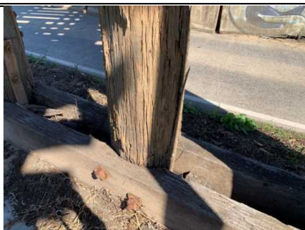
Pier 7 centre pile hollow & evidence of white ants at base of pile
