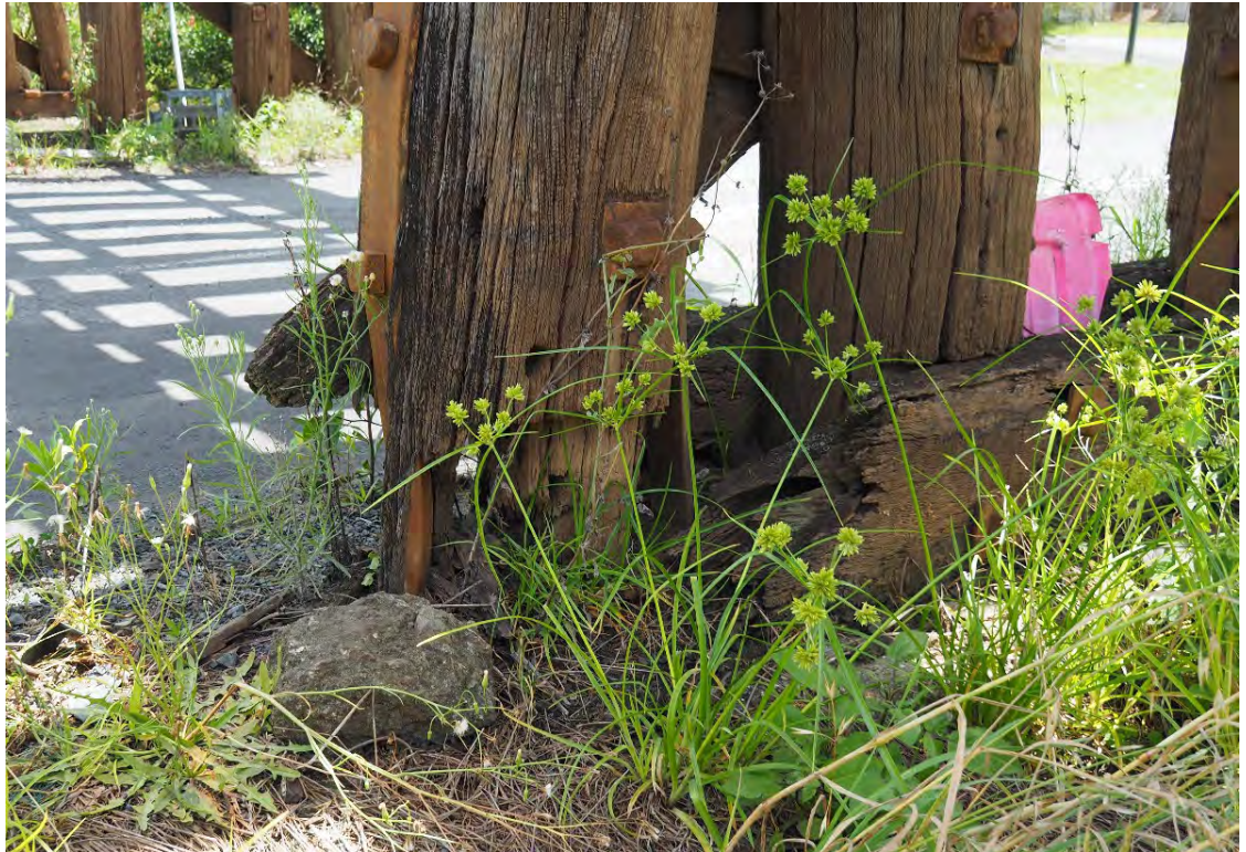
Figure B-3 Alexandra Parade – Rotten/Infested pile & whaling at Pier 23 (Source: FBE)
