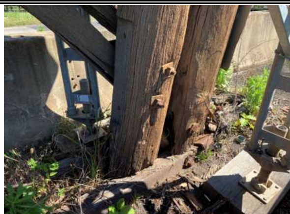
Pier 6 west pile vehicle impact damage and movement towards east at the base of pile
