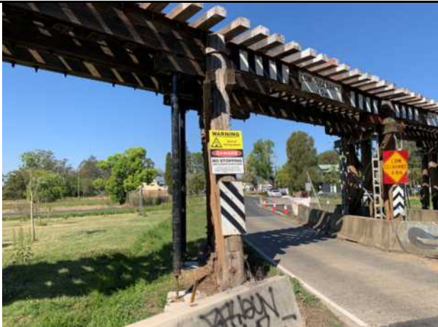
Pier 7 not vertical 150mm - leaning to north end of bridge
