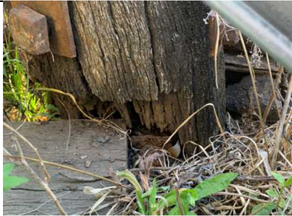
Pier 6 east spur pile rot and hollow at base
