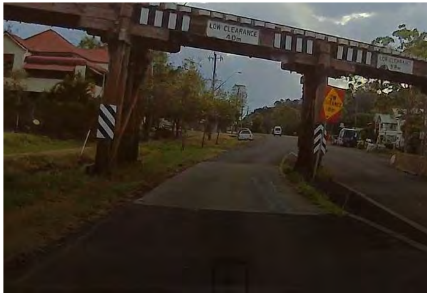
Photo 10: Minimal edge clearance - Terania Street viaduct
