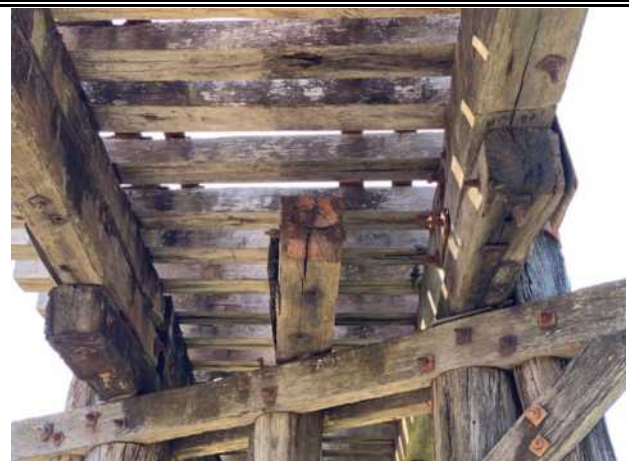
Pier 7 south end of corbels minor splits
