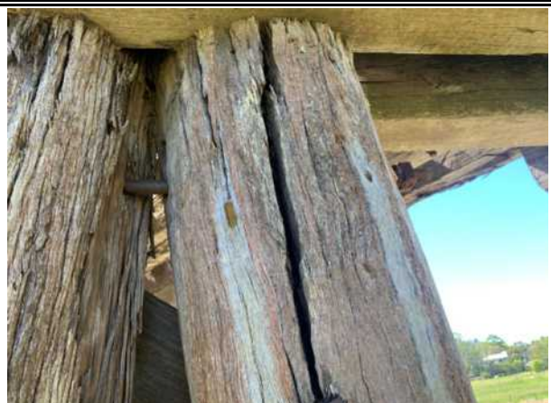
Pier 4 west pile cracked at head of pile
