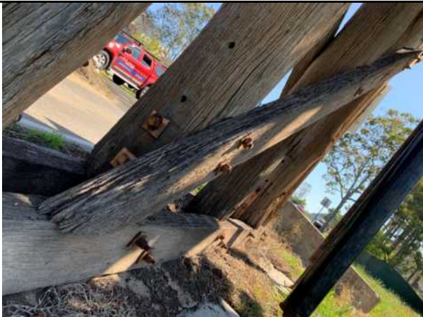
Pier 7 north diagonal brace weathered
