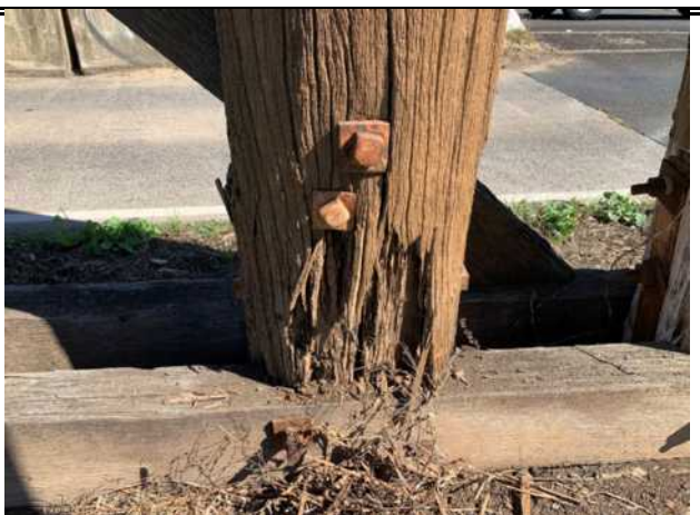
Pier 7 west pile hollow & evidence of white ants at base of pile
