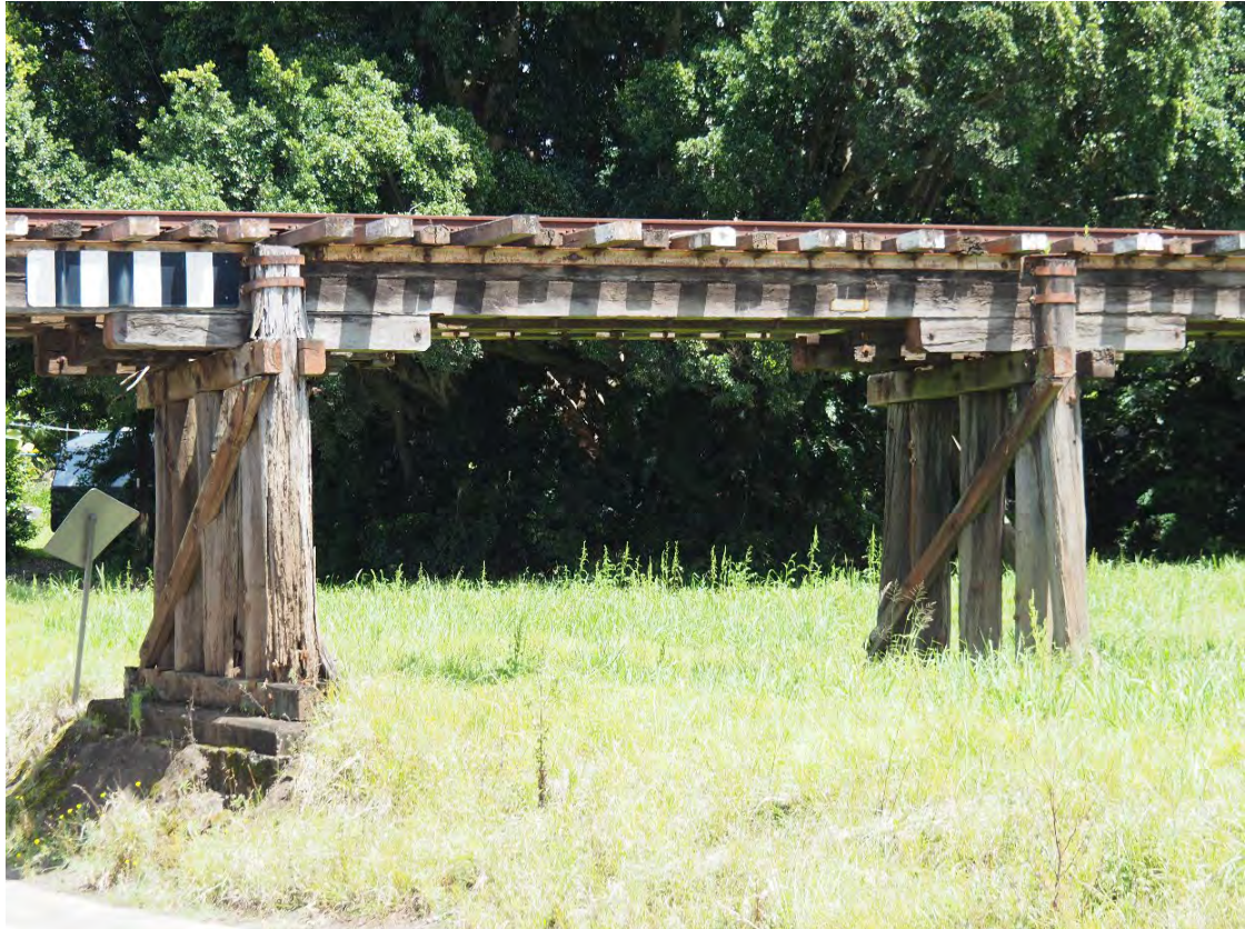
Figure B-18 Union Street – View looking west, typical condition of timber span (Source: FBE)
