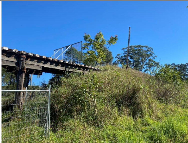
Photo 4: Weedy regrowth on bridge abutments
