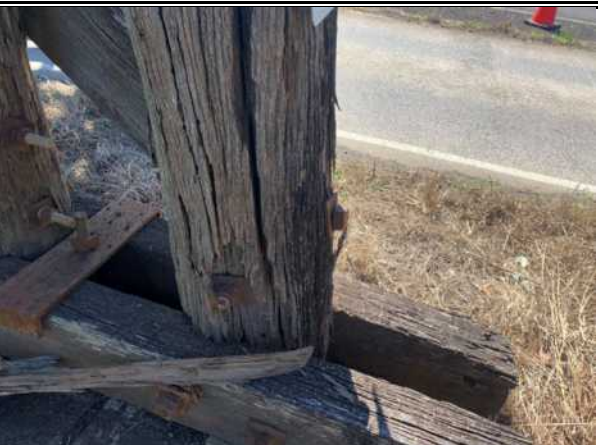
Pier 4 east spur pile cracked & hollow at base of pile
