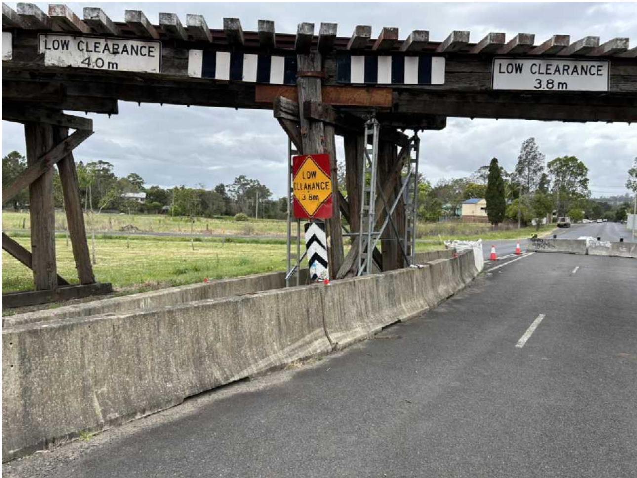
Figure 6: Signs of impacts with superstructure
