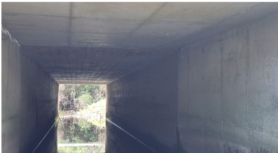
Photo 3-5: Example of culvert condition at Winding Creek
