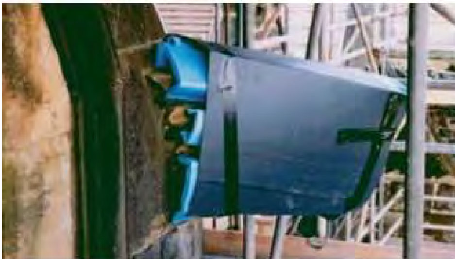
Figure B-3: Wrapping of smaller heritage features with foam and core-flute during construction.
