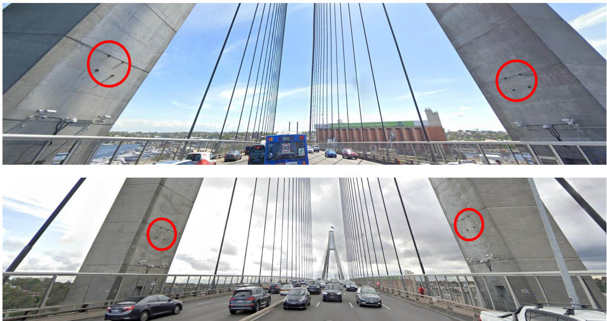
Figure 4.2 Views of the stainless steel bearing housings on both bridge towers of the Anzac Bridge. (Source: Google StreetView, September 2020)
