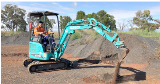
Spoil from the project being spread out at a local business in Dubbo
