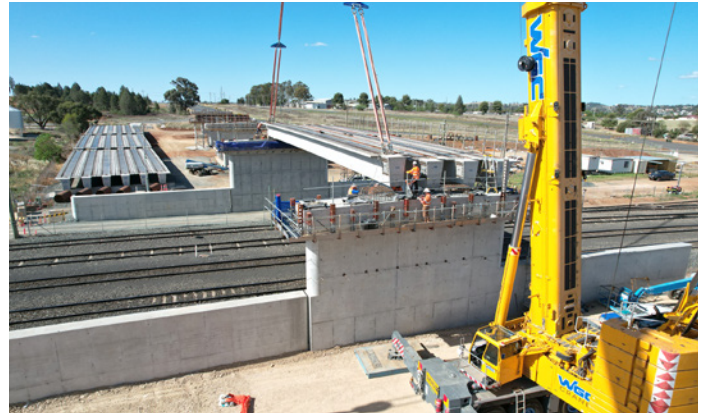
A precast girder being lifted into position for the Bridge over Rail and Hartigan Avenue
