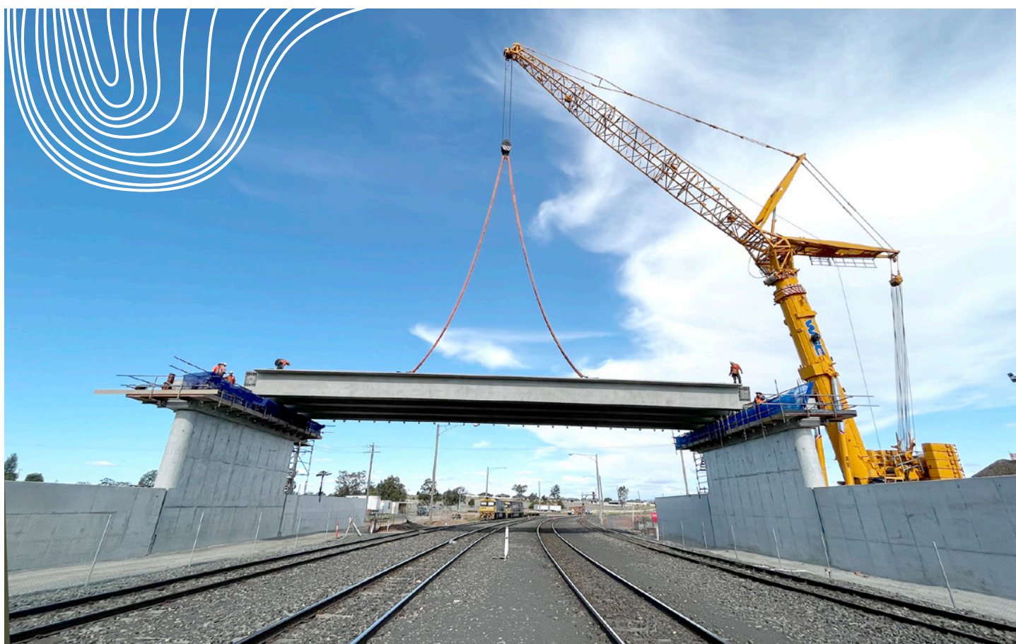
A precast girder being lifted into position for the Bridge over Rail and Hartigan Avenue
