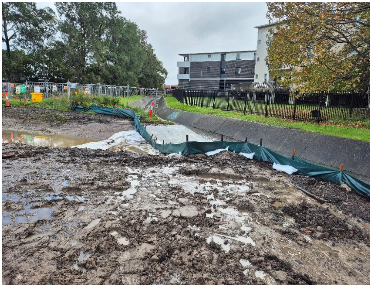
Image 7: ErSed controls around Zone 1, which drains into Dark Creek (concrete culvert). View looking north (downstream).
