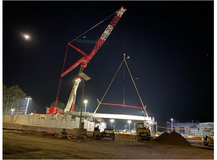
Image 10: Image of the 750 tonne crane lifting the girders for the bridge across Newcastle Road (Image 2)
