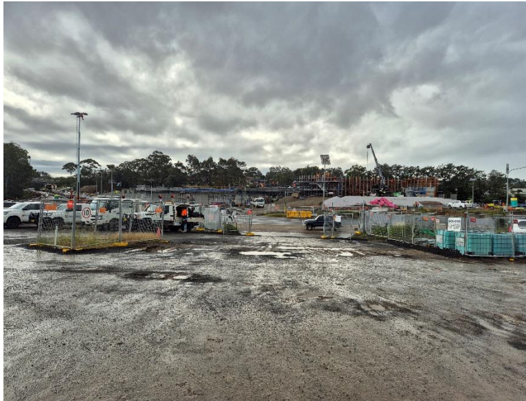
Image 1: Northern Interchange, looking northeast from the Jesmond compound at the entrance to the compound site from Newcastle Road.
