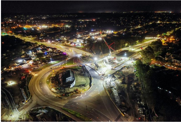
Image 9: Image of the 750 tonne crane lifting the girders for the bridge across Newcastle Road (Image 1)
