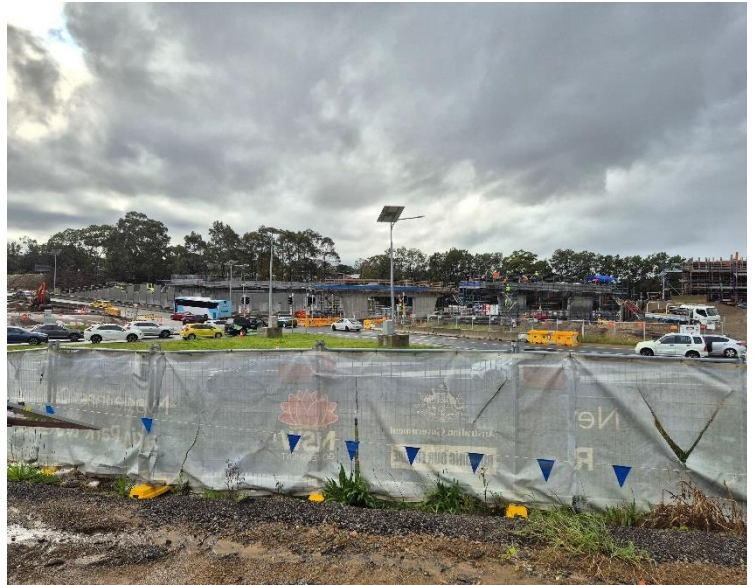
Image 2: Northern Interchange, looking northeast from the Jesmond compound across to the Newcastle roundabout and the new bridge piers.
