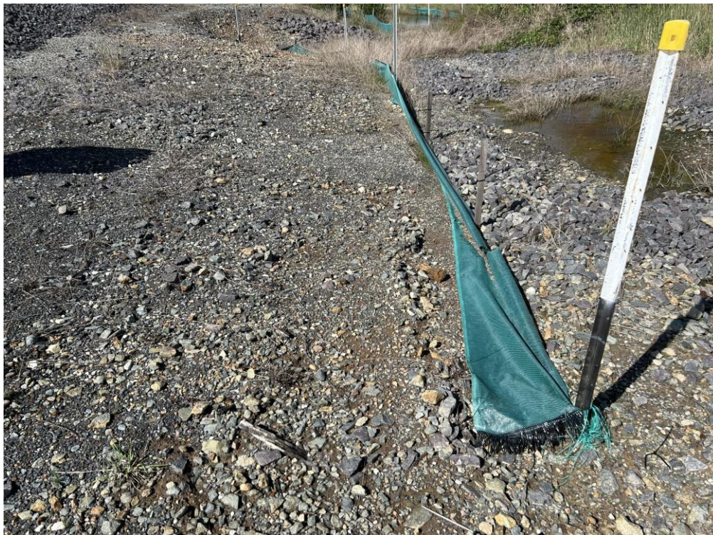
Photo 9: Sign of damaged sediment fencing at the diddle culvert upgradient of the railway line.
