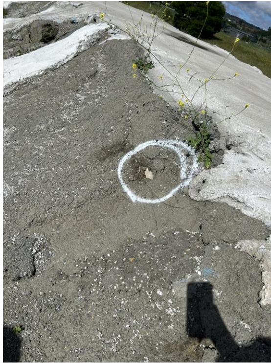
Photo 13: Concrete capped stockpile. New signs of damage (2). Facing north.
