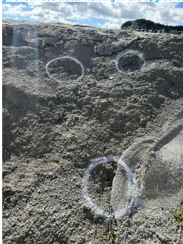
Photo 12: Concrete capped stockpile. New signs of damage (1). Facing north.
