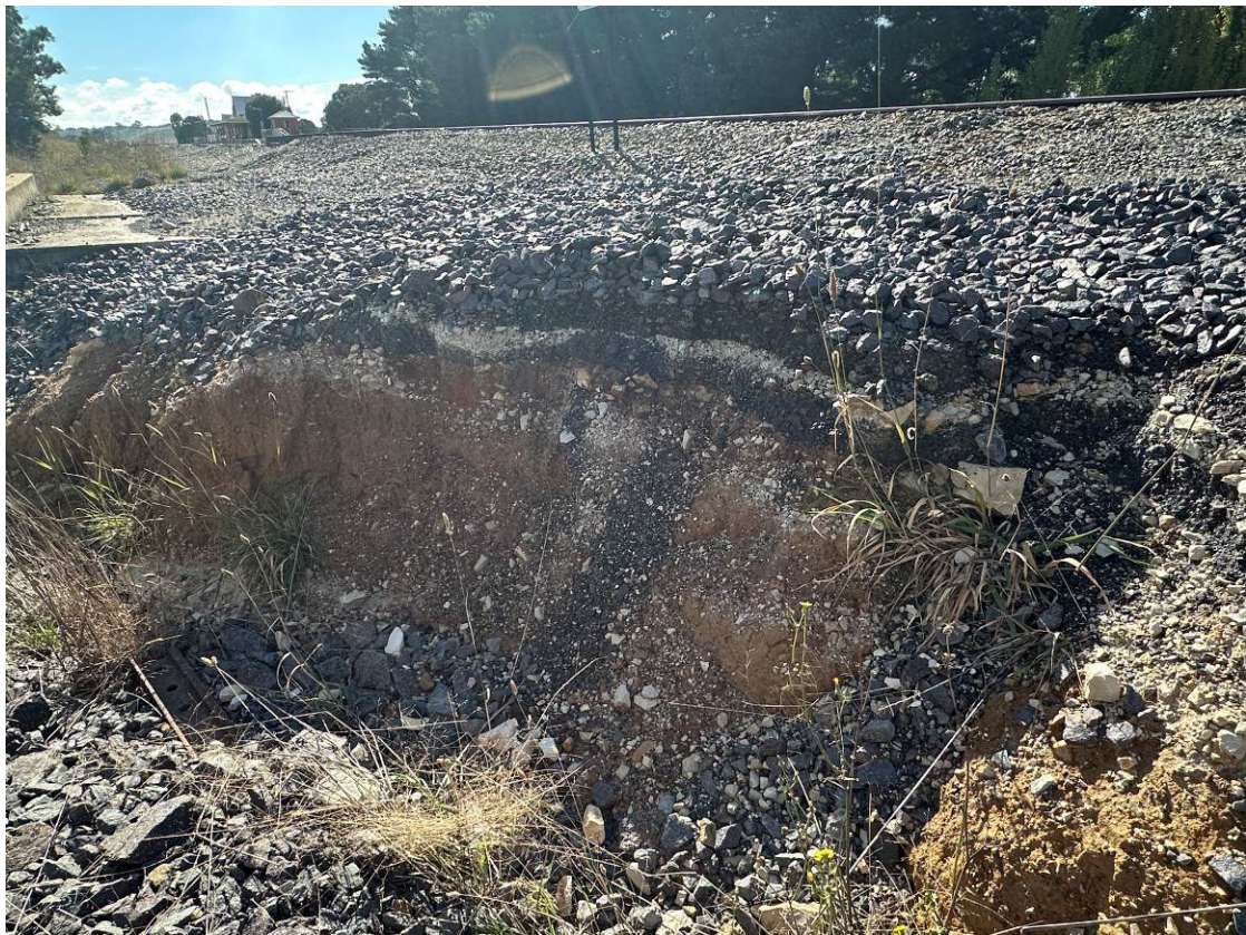
Photo 11: Southernmost culvert upgradient of the railway line. Evidence of erosion due to lack of ground cover. Minor to no changes since previous inspection.
