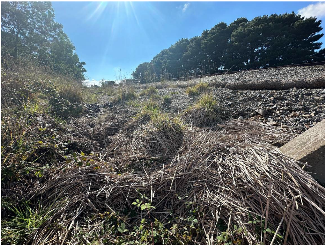
Photo 12: Drainage line leading to southernmost culvert upgradient of the railway line. Evidence of previous high surface water flow (build-up of vegetation debris).
