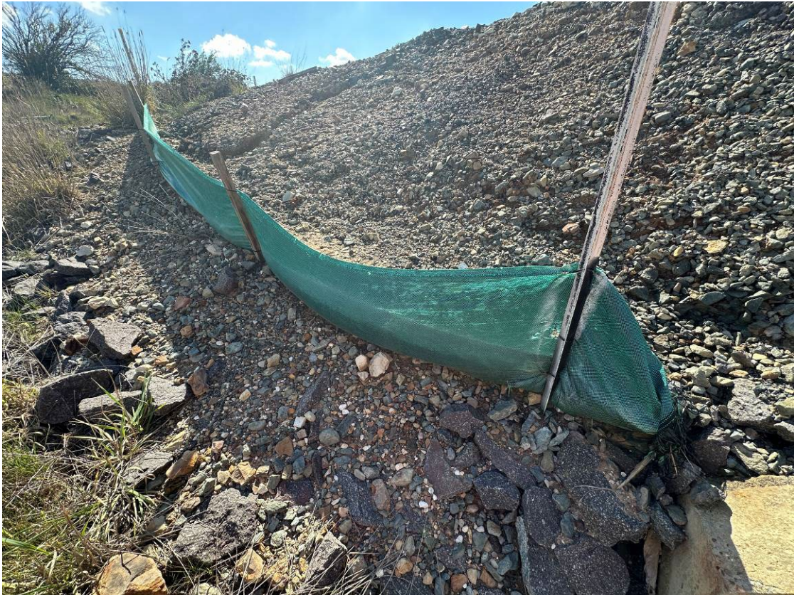
Photo 17: Upgradient of railway line to the north of the middle culvert. Sediment fencing in place with large build-up of sediment.
