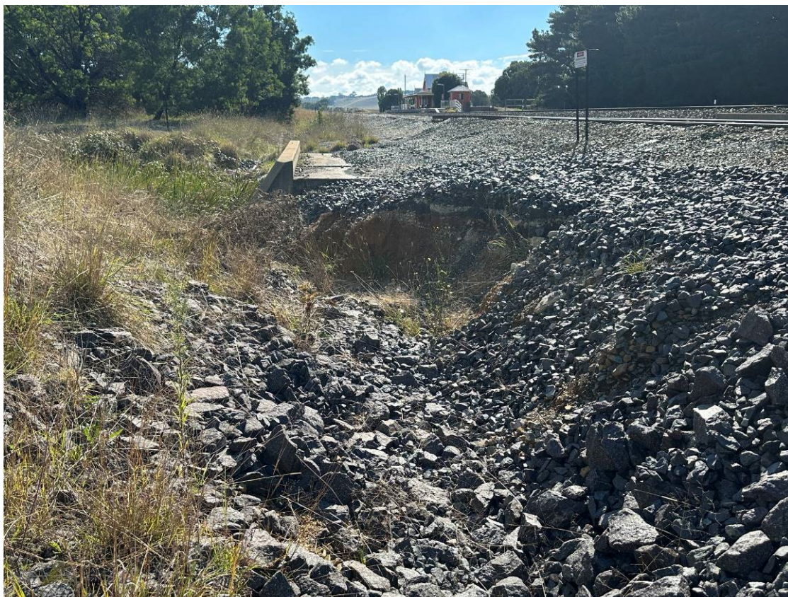
Photo 10: Facing towards southernmost culvert upgradient of the railway line. Rock armoury within drainage line to culvert. Some evidence of erosion.
