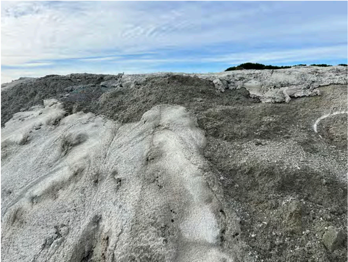
Photo 19: Minor hairline cracking is present on the stockpile
