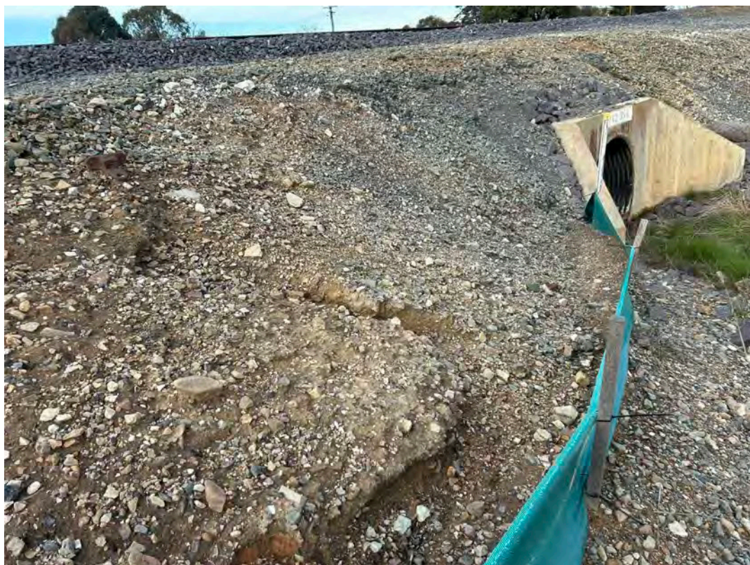
Photo 12: Upgradient of railway line to the north of the middle culvert. Sediment fencing in place with large build-up of sediment. Some minor erosion due to inadequate ground cover was observed.
