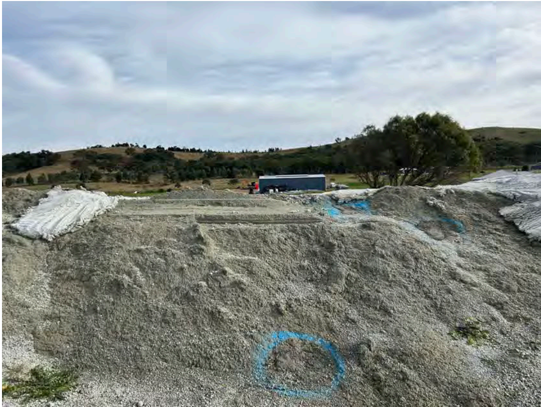
Photo 17: Three locations of exposed geofabric layer marker on stockpile noted during previous inspections appeared to have been filled with cement.
