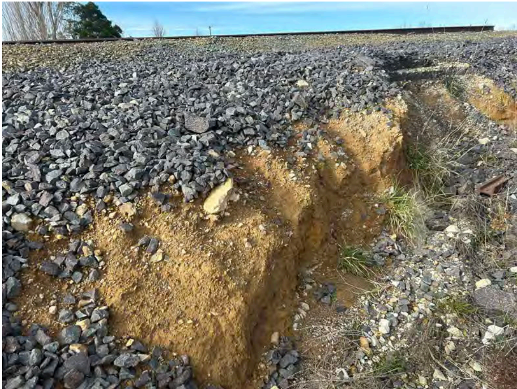
Photo 7: Southernmost culvert upgradient of the railway line. The erosion due to lack of ground cover observed during previous inspections is still present.
