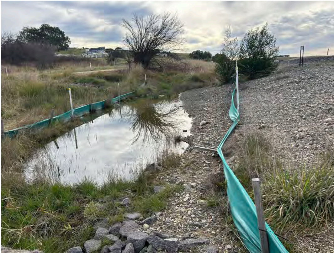
Photo 13: Previous inspections noted that the sediment fencing in drainage line north of middle culvert has some damage and needs to be replaced. No change was noted in this inspection.
