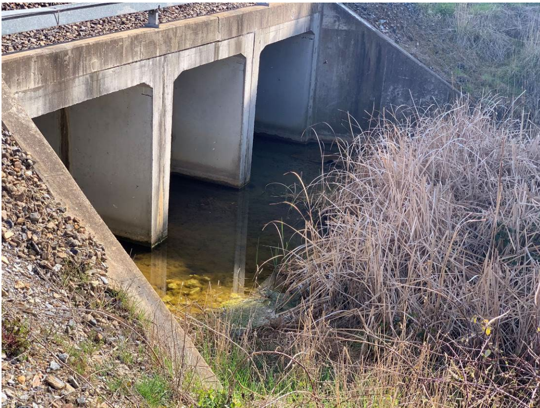
Photo 3: Southern most culvert downgradient of rail line, with slow moving surface water travelling off-site. Water is clear, low turbidity, minimal observable sediment, long grass and some algae present.
