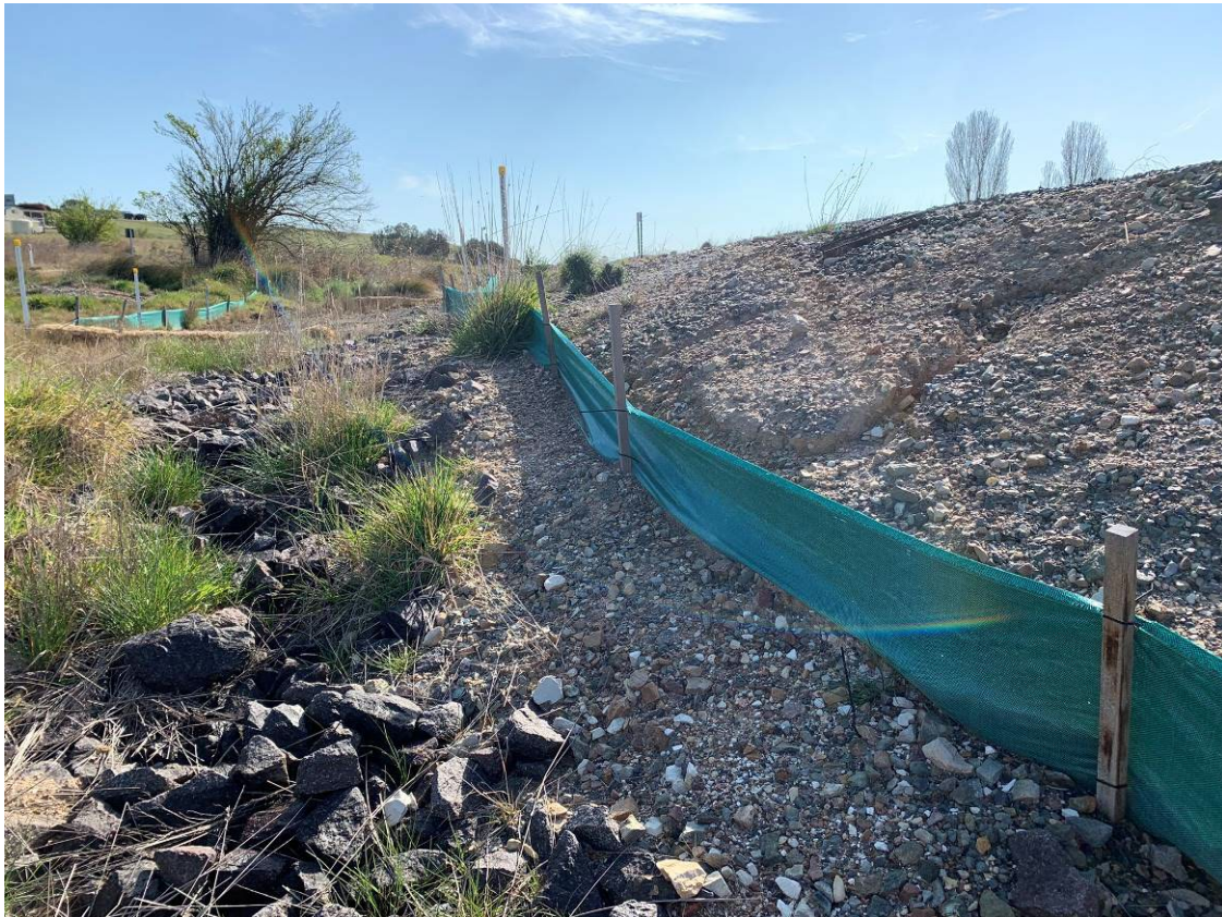
Photo 14: Upgradient of middle trainline culvert facing east. Silt fencing is clear with no sediment visible.
