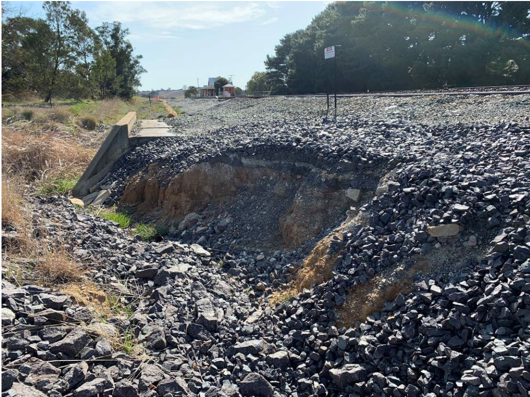
Photo 9: Visible evidence of erosion due to loss of ground cover (ballast material) upgradient of southernmost culvert. Remaining stable and no major further erosion since last inspection. Facing north-east.
