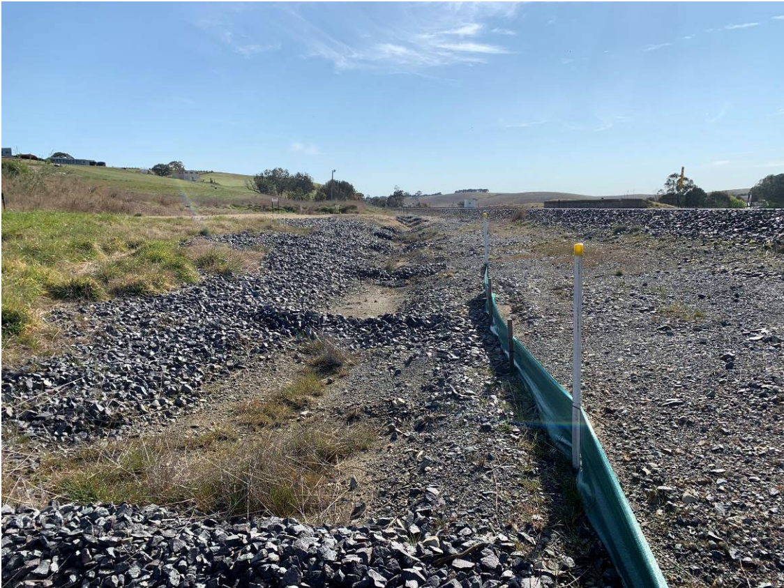
Photo 15: Rock armour upgradient of trainline running from the middle to the north culvert. Some sediment visible on rock armour. Facing north-east.
