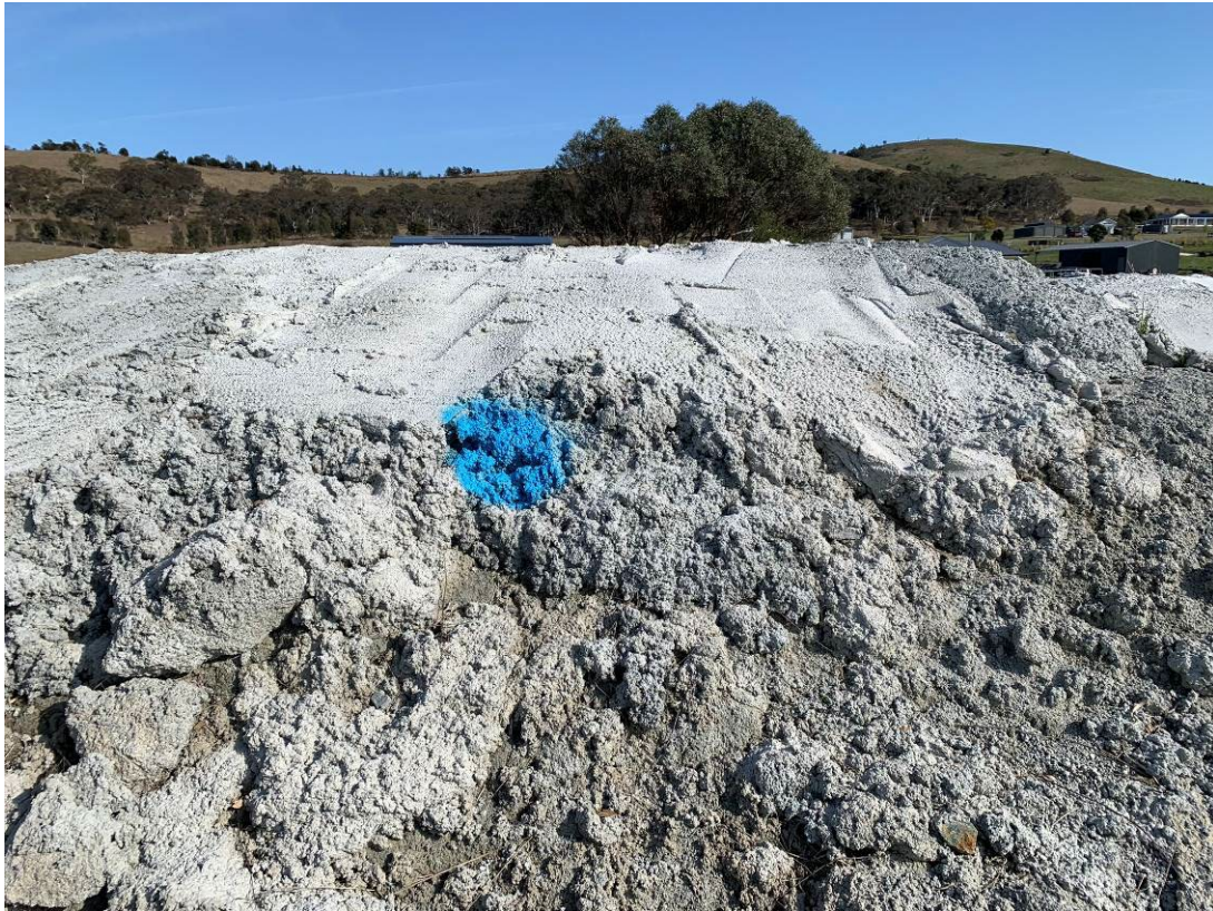
Photo 21: Exposed geofabric layer marker on main stockpile newly identified during the inspection. Marked with blue paint. Facing the north-western side of stockpile.
