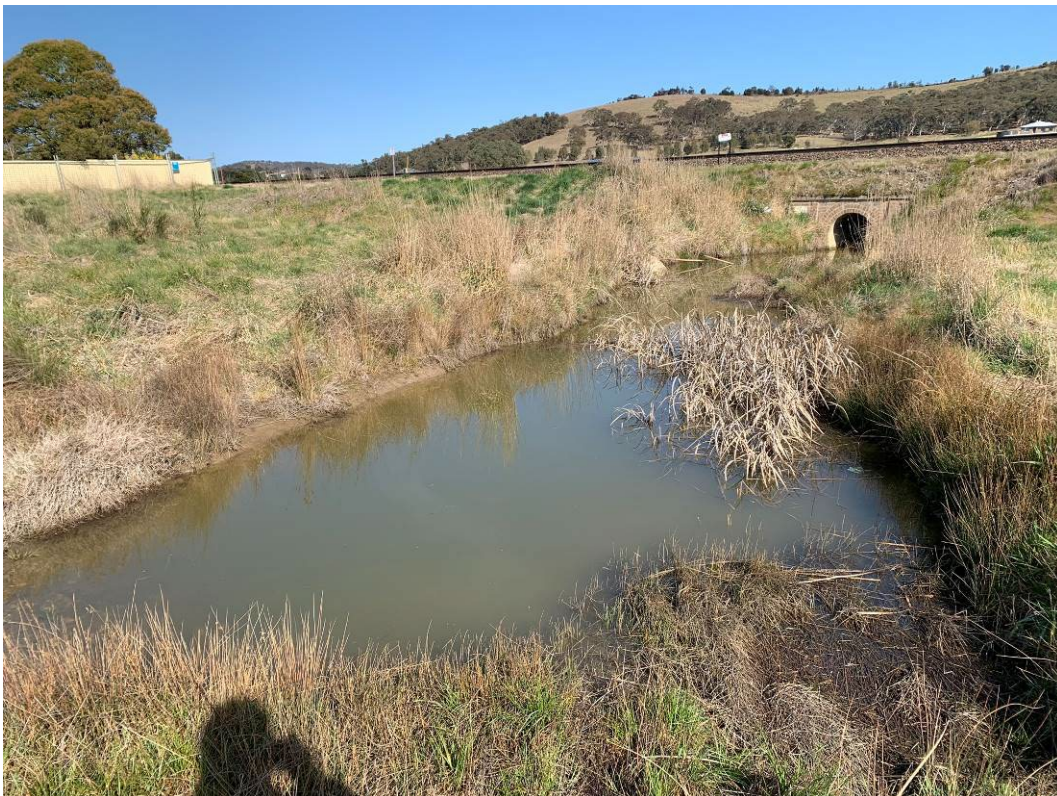
Photo 4: Downgradient of middle culvert showing brown turbid water on site. No surface water currently running off site at middle culvert.
