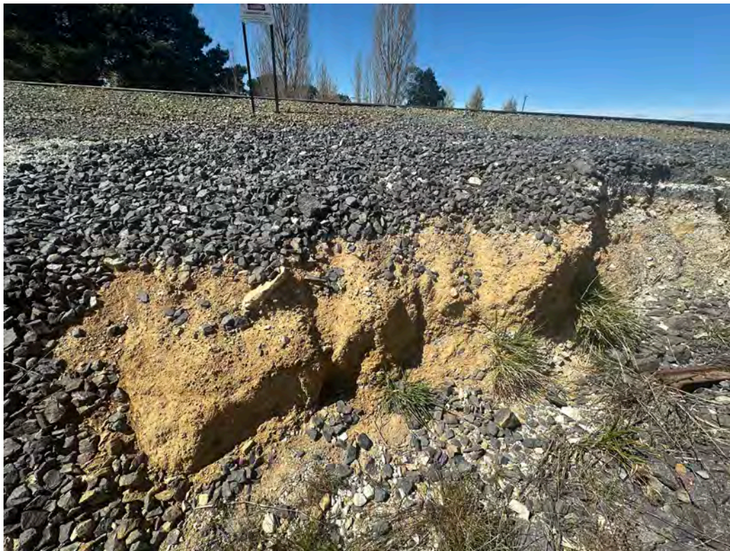
Photo 7: Southernmost culvert upgradient of the railway line. The erosion due to lack of ground cover observed during multiple previous inspections is still present.
