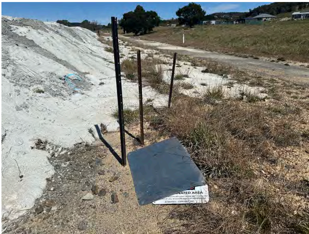
Photo 17: Minor damage to signage surrounding concrete-capped stockpile. UGL representative fixed and replaced ties after the site inspection.
