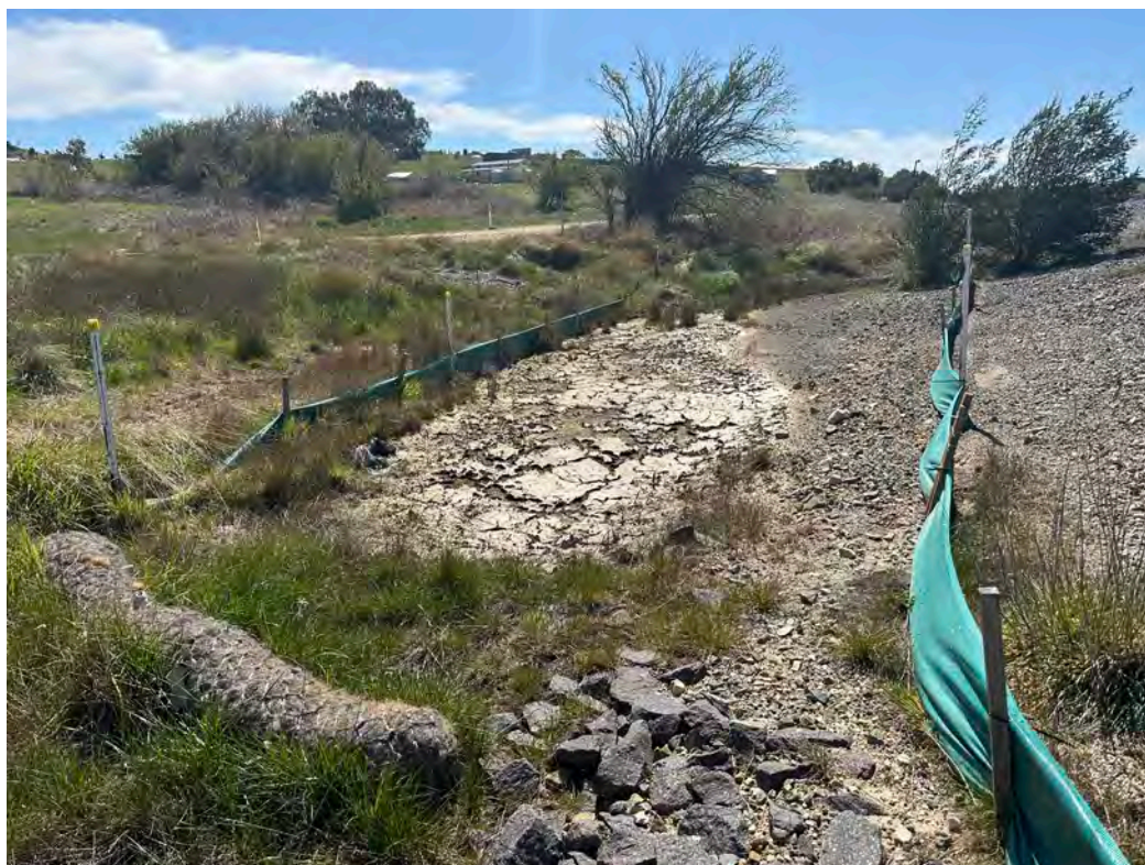
Photo 12: Sediment fencing in drainage line north of middle culvert has some new damage and sediment build up and needs to be replaced.
