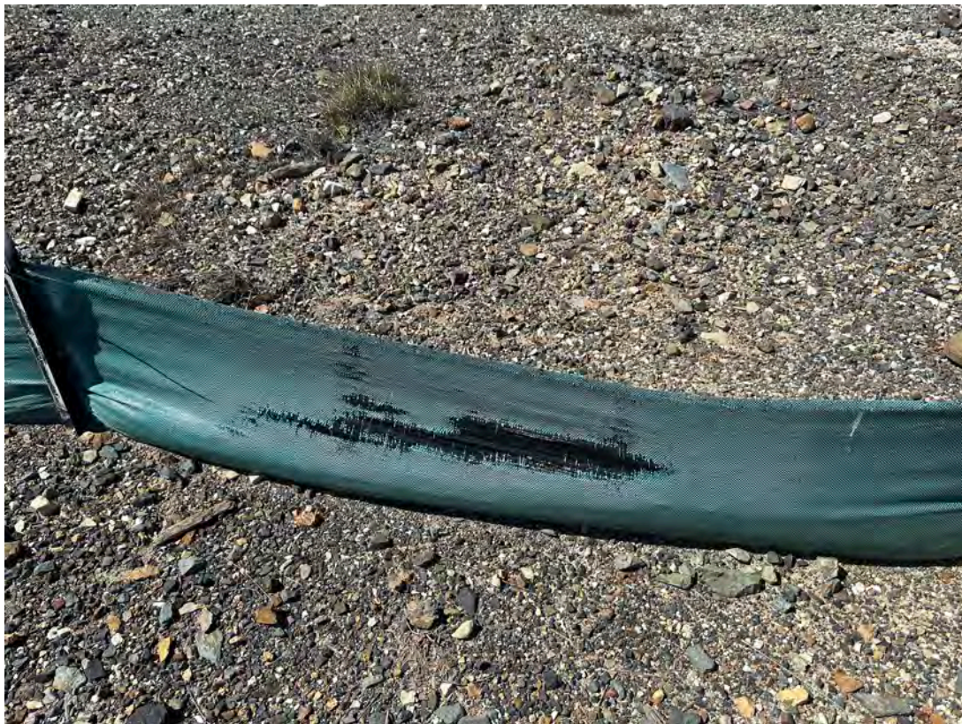
Photo 13: Damage to sediment fencing in drainage line north of middle culvert that needs to be replaced.
