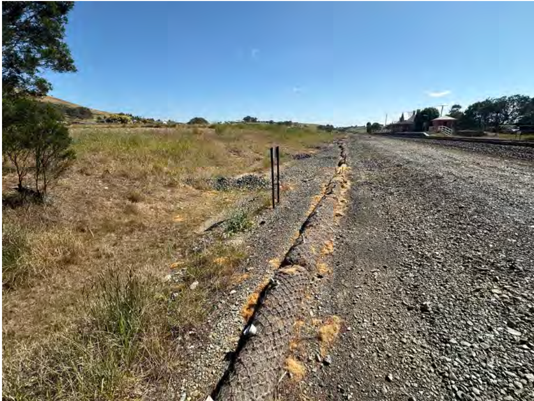
Photo 19: Minor damage to sediment coir logs between southern and middle curvet. Suspected to be caused by birds.
