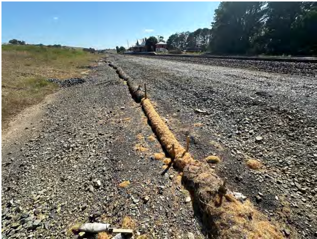
Photo 11: Damage to sediment control coir logs between southern and middle culverts has been maintained and some logs replaced. Suspected damage caused by birds.
