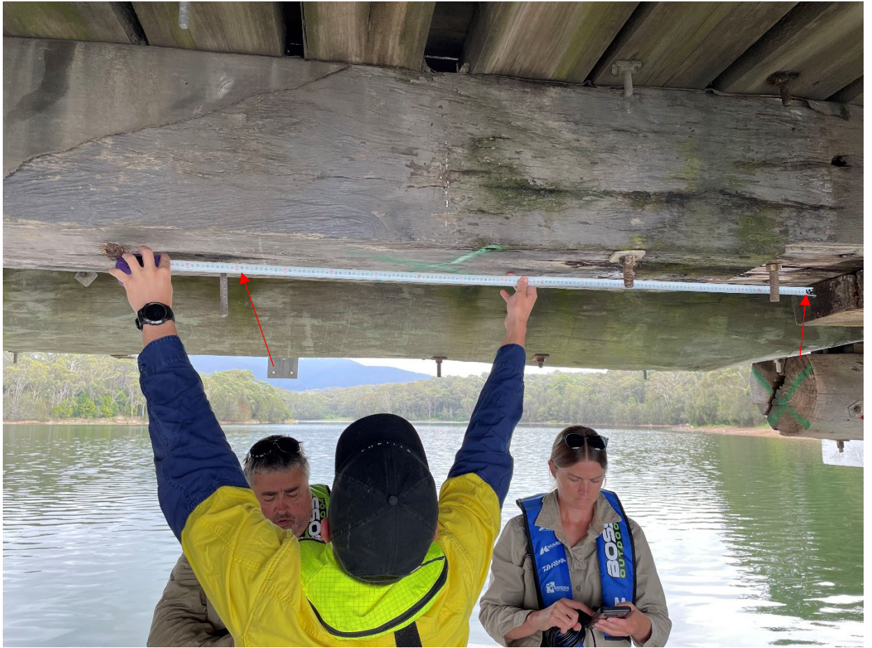
Figure 1-5: Photograph of Girder 19 detailing gap between the two entry holes used by Southern Myotis to enter this girder.
