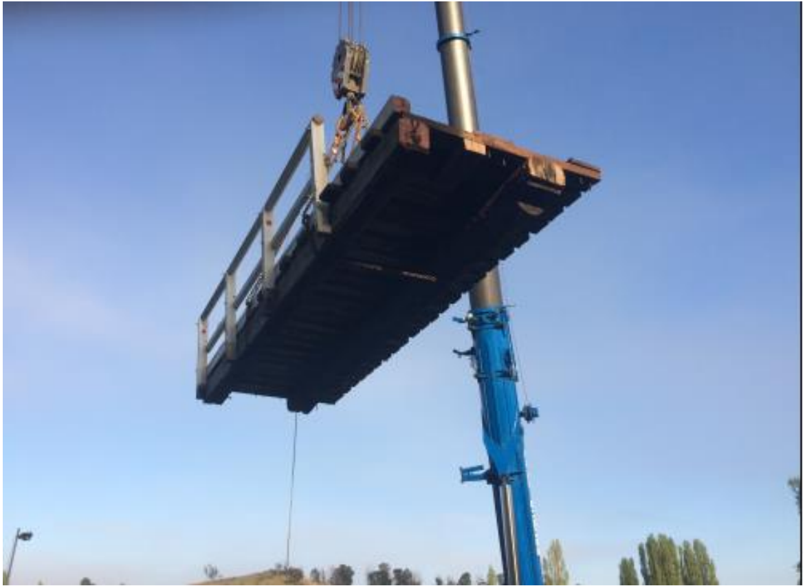
Figure 3-5: Example of deck removal in spans which encompasses 2 girders, cross decking, kerb and handrail
