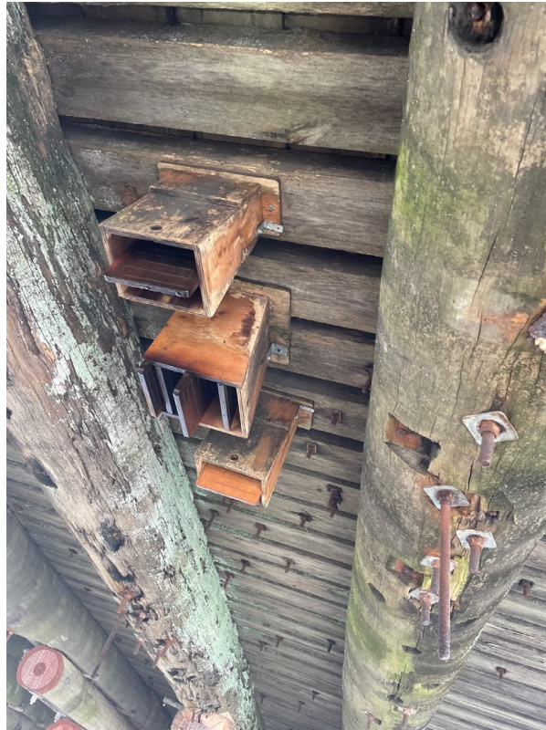
Figure 2-2: Example of two and four chambered bat boxes installed on a Transport bridge project
