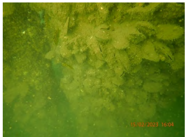
Photo 4. Mussels were common on all piles with abundant on piles of pier 6.
