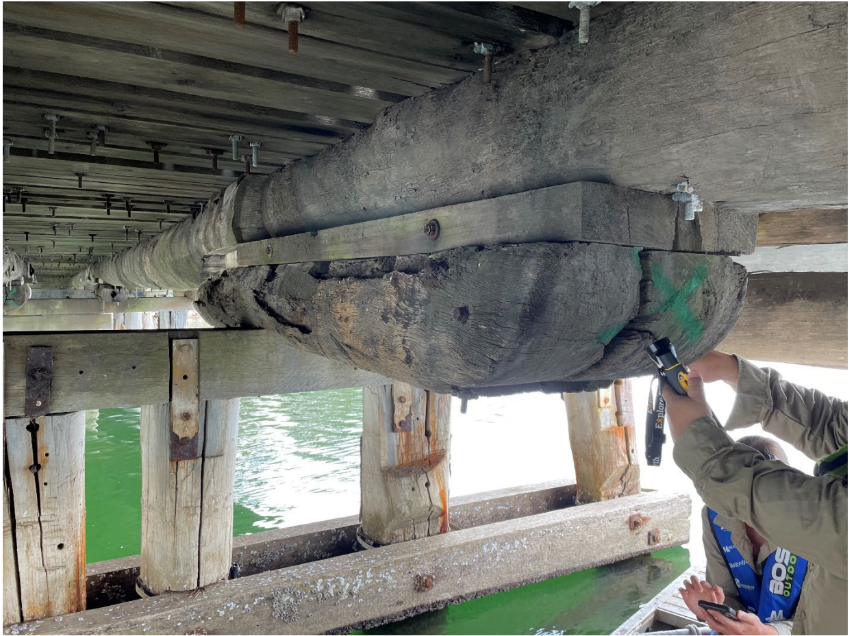
Figure 1-6: Photograph of Corbel 22 showing crack at end of corbel which is the entry/exit point for Southern Myotis.
