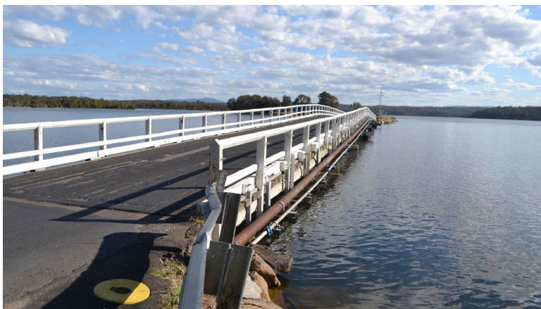
Figure 2: View of the bridge looking south detailing the subtle arch of the deck and superstructure along with attached services.
