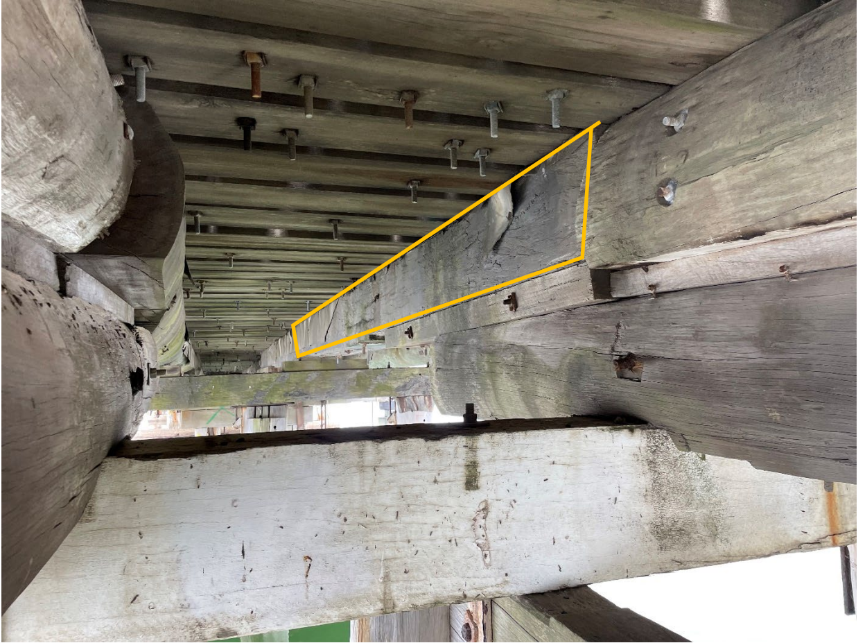
Figure 1-4: Photograph of Girder 19 (currently labelled as Girder 20 due to temporary girders having been installed) – to be referred to as Girder 19 within this document.
