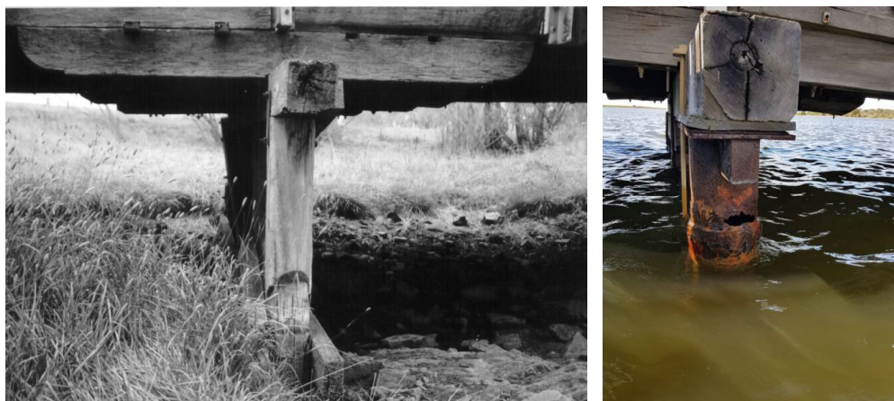
Figure 4a: Typical early headstock detail at top of pier. Figure 4b: Same headstock detail in place on Wallaga Lakes Bridge.
