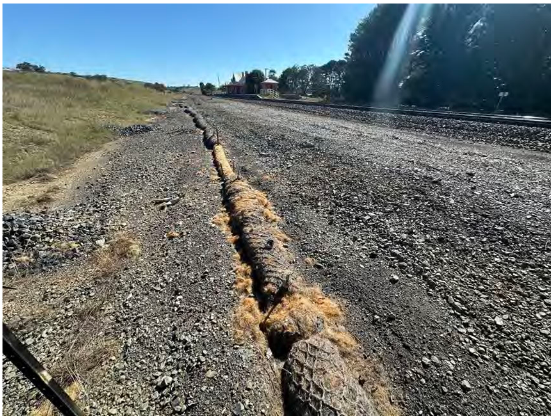
Photo 12: Damage to sediment control coir logs between southern and middle culverts maintained appropriately. Suspected damage caused by birds.
