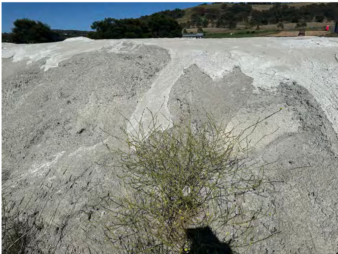
Photo 20: Minor vegetation and weeds growing out of stockpile capping.
