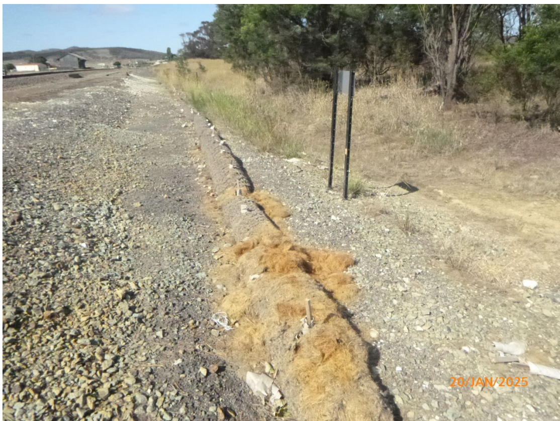
Photo 10: Damage to sediment control coir logs between southern and middle culverts.
