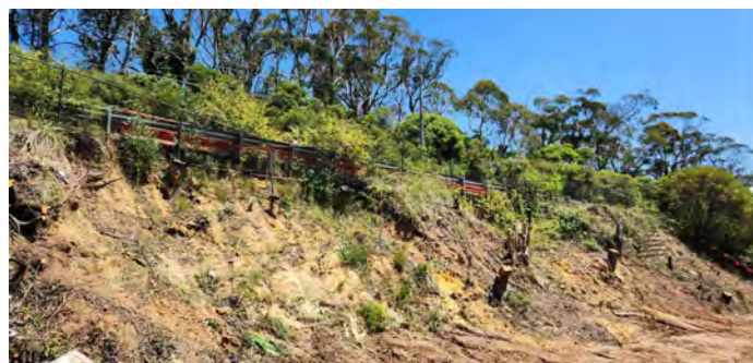
Katoomba U-turn Bay slope before work began, showing the extent of the failure
