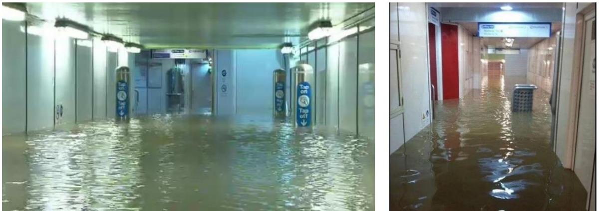
Figure 6-19: Flooding at Lewisham Station underpass (source: 9News Sydney October 2014)
